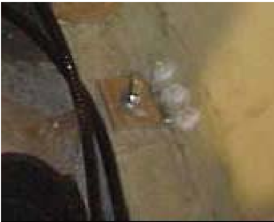
Figure 2 - Radome mounting to the tower platform - galvanized steel plates
