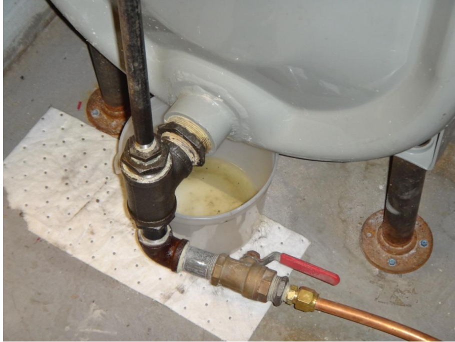
Photo-1: Oil Leak Location at the Day Tank
