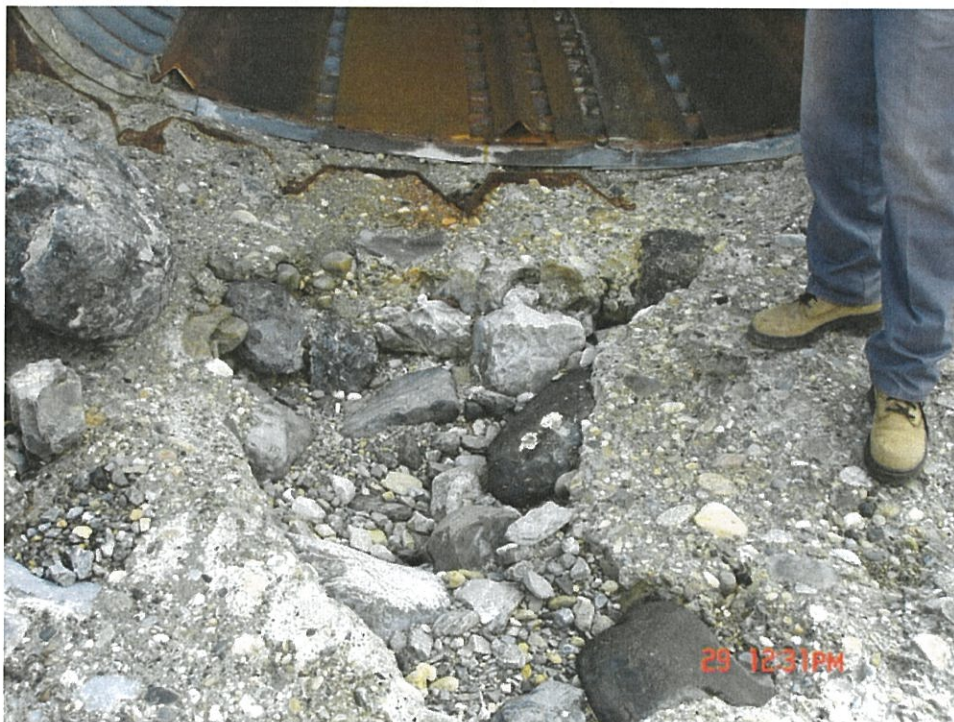
26.2 – Fill Outlet Scour Hole and Apron with RipRap (Details for Handplaced RipRap in Appendix A)
