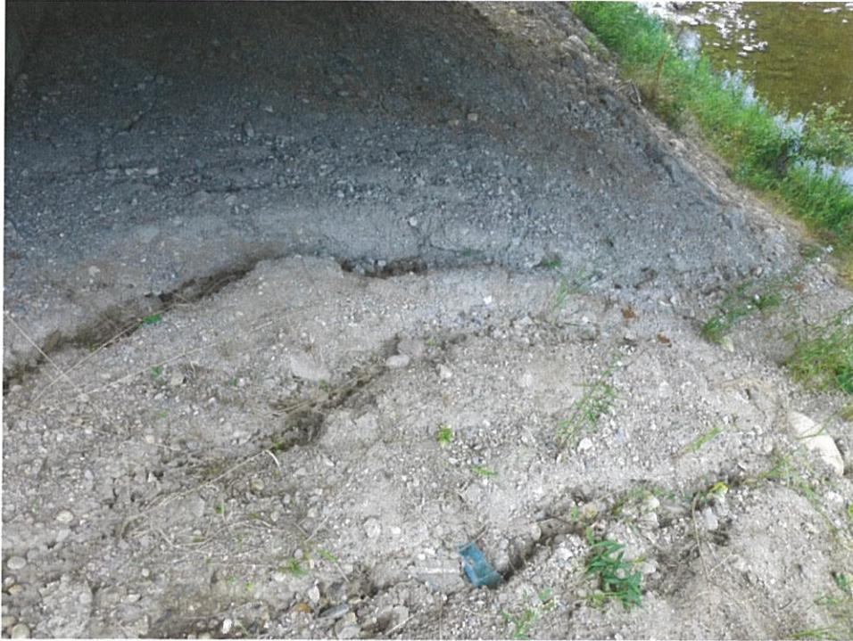
6.1 – Repair Erosion at Top of Embankment and at Approach Barrier Drains
