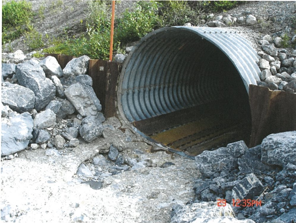
26.1 – Fill Outlet Scour Hole and Apron with RipRap (Details for Handplaced RipRap in Appendix A)
