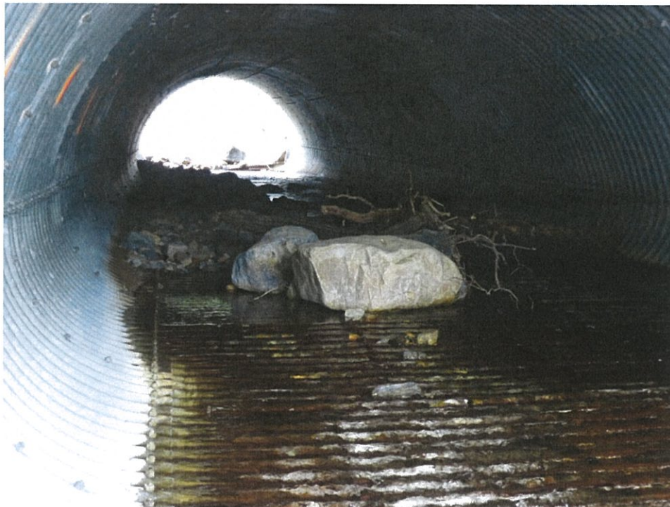
16.2 – Remove Large Boulders from the Interior of Both Barrels. Do Not Remove Boulders from Inlet or Outlet
