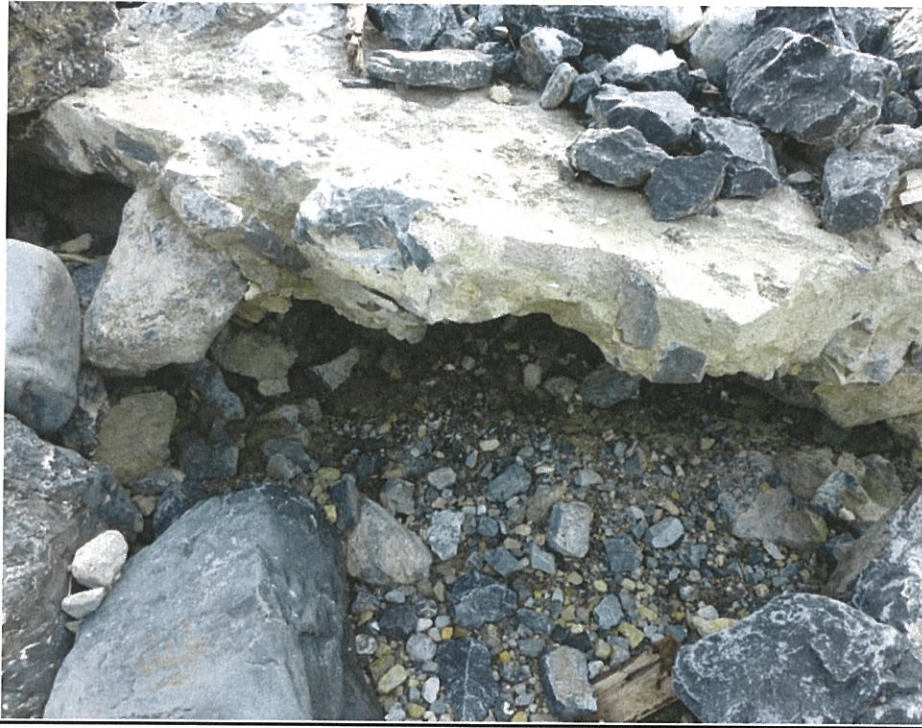
27.1 – Fill Scour Hole at Outlet with Concrete
