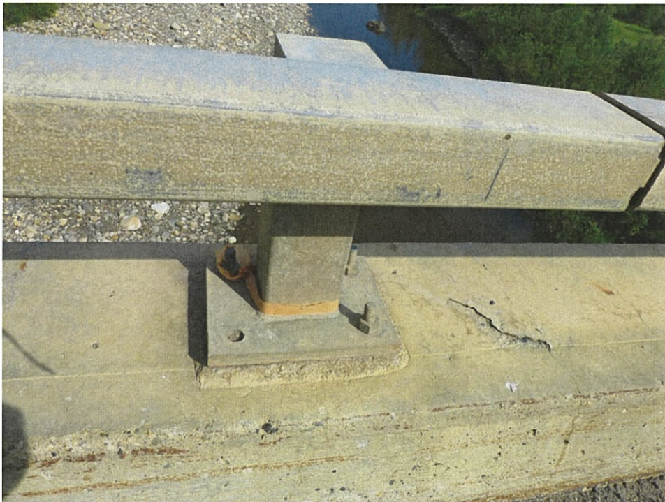
3.3 – Install Missing Barrier Bolts
