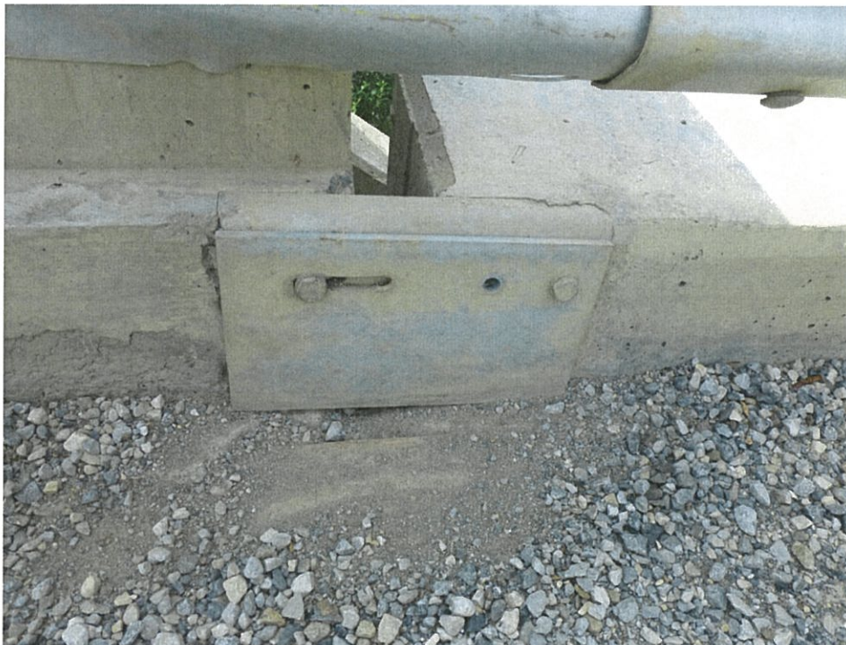
18.2 – Curb Joint Steel Cover Plates Restricted. Install ½" Notch on Both Sides of Curb Plate
