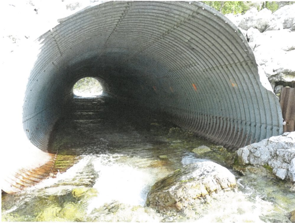
16.1 – Remove Large Boulders from the Interior of Both Barrels. Do Not Remove Boulders from Inlet or Outlet
