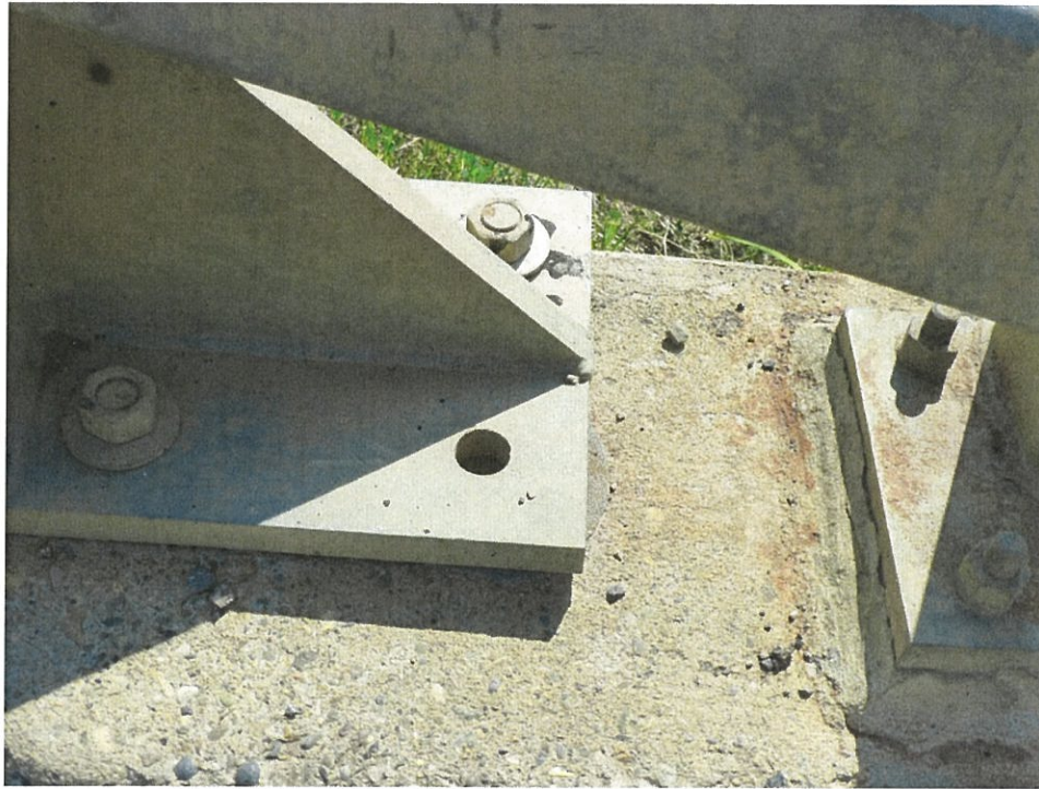
12.1 – Replace Missing Barrier Bolt (SW Barrier Transistion)
