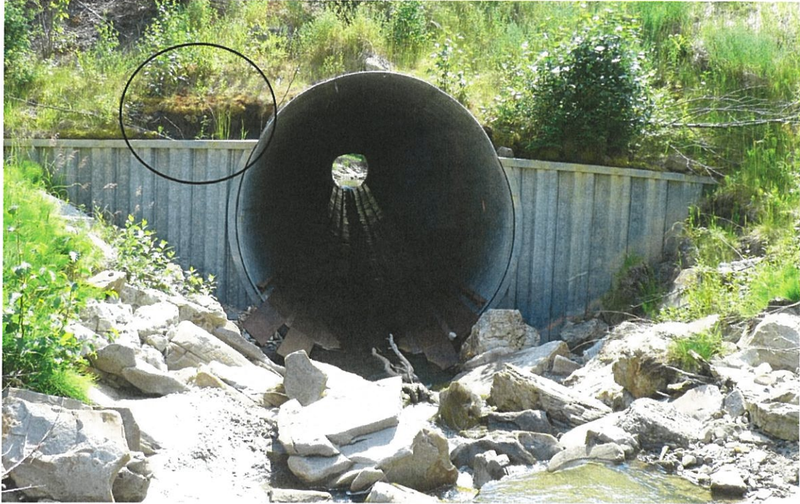
14.1 – Repair the Erosion Around the Inlet
