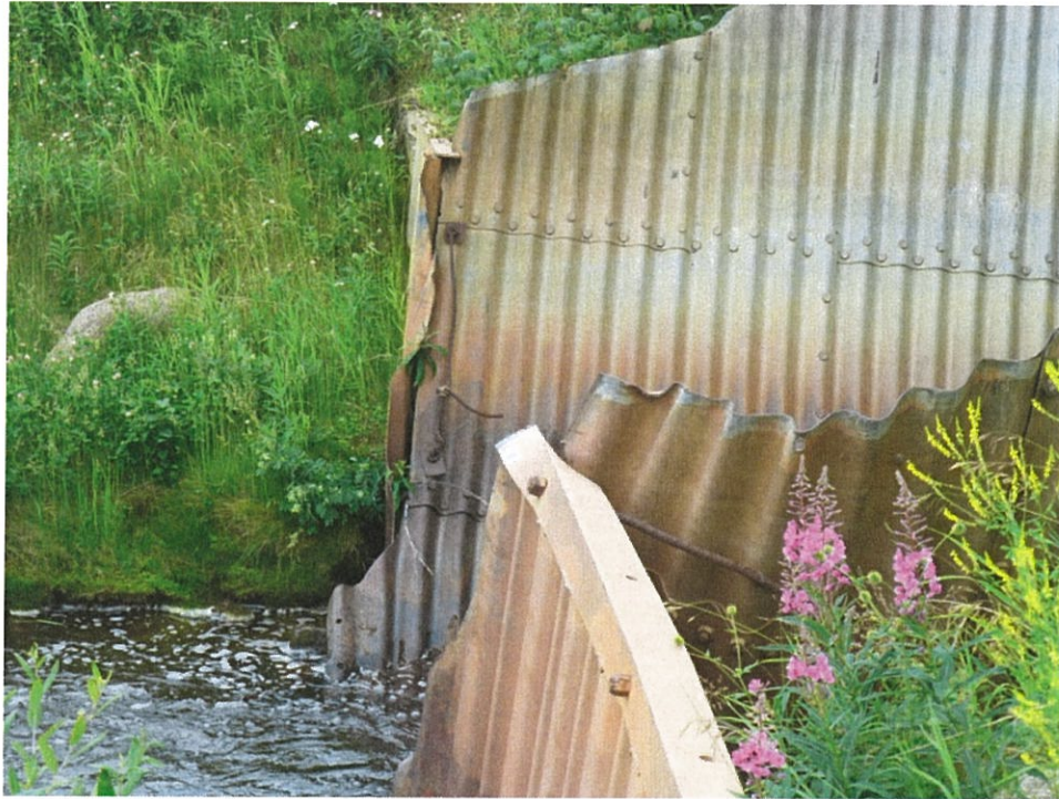
4.1 – Backfill Void Behind the Inlet Binwalls
