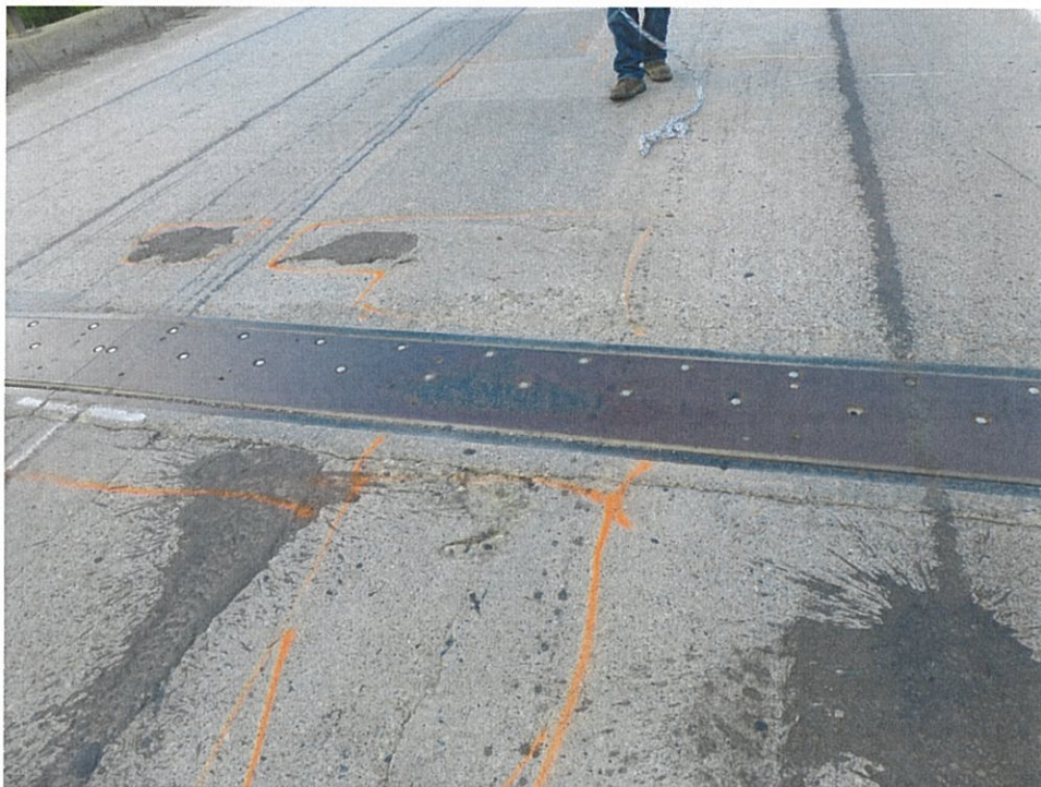
6.2 – Install Two Missing Barrier Bolts at South Deck Joint, Northbound Section
