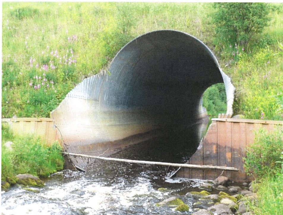
4.2 – Backfill Void Behind the Inlet Binwalls
