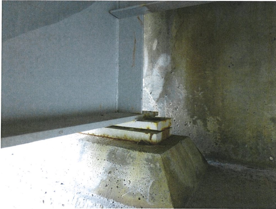
18.3 – Install 2 Missing Bearing Bolts (Details Located in Appendix A)
