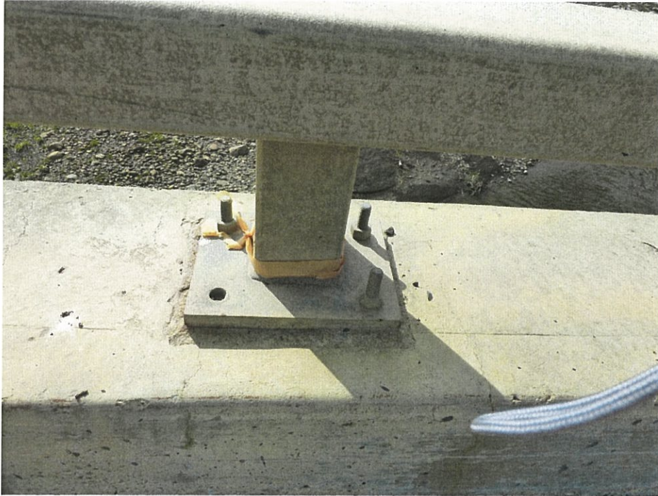
3.4 – Install Missing Barrier Bolts
