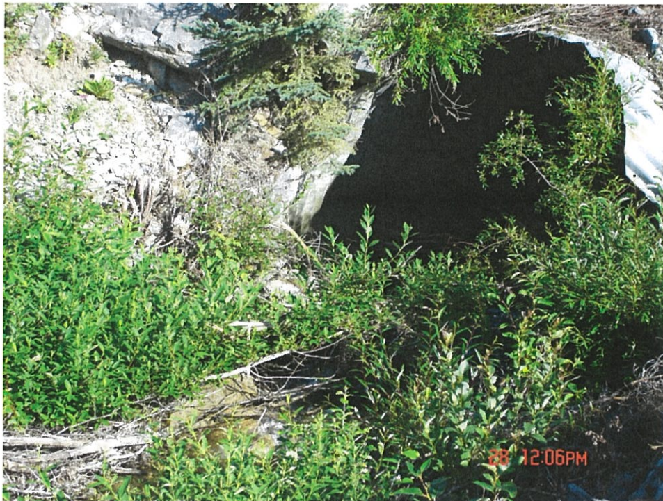
20.2 – Clean the Tree Debris and Branches Inside of Barrel, at Outlet and in the Creek
