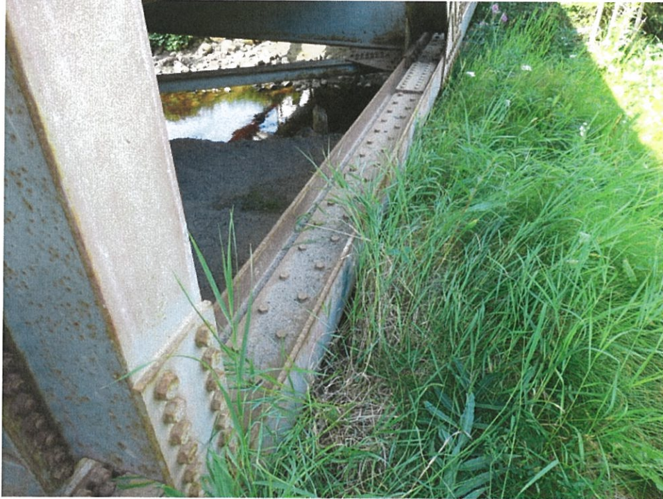
10.1 – Make 6" – 12" Soil Clearance from Bottom Trusses
