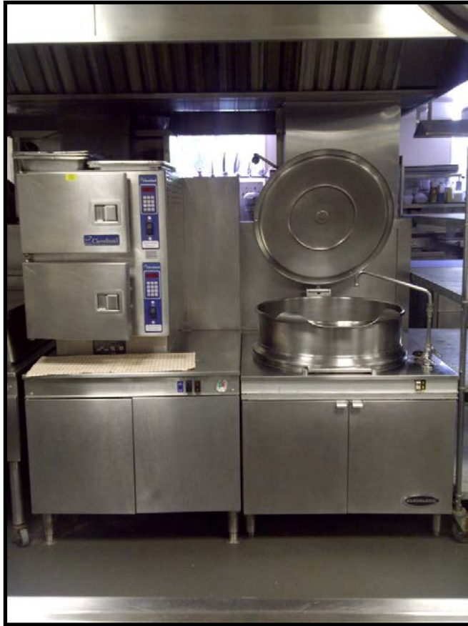
Photo 1: Front view of equipment to be replaced.
