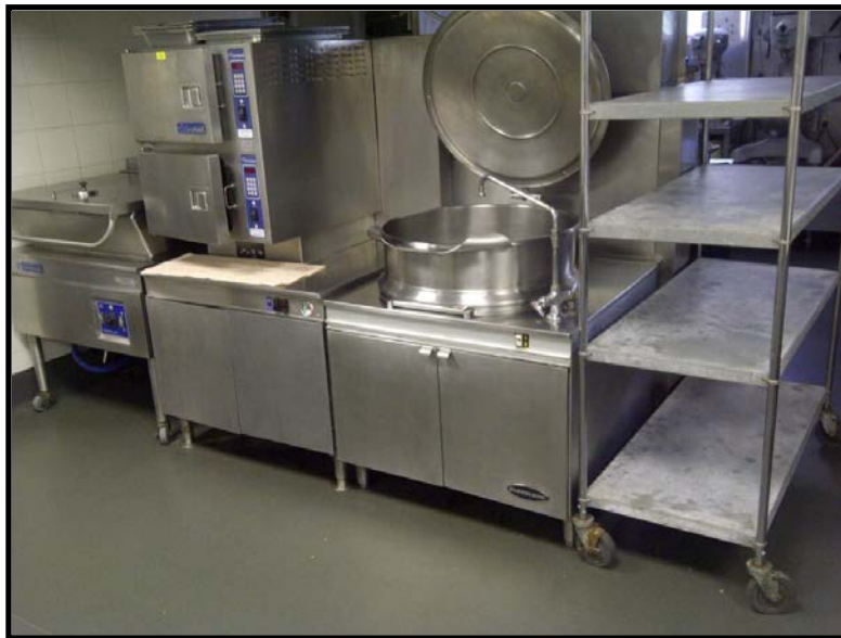
Photo 2: Angled view of equipment to be replaced.
