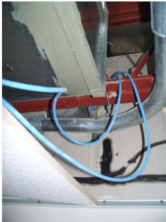
Photograph No. 4 Asbestos-containing black sealant
