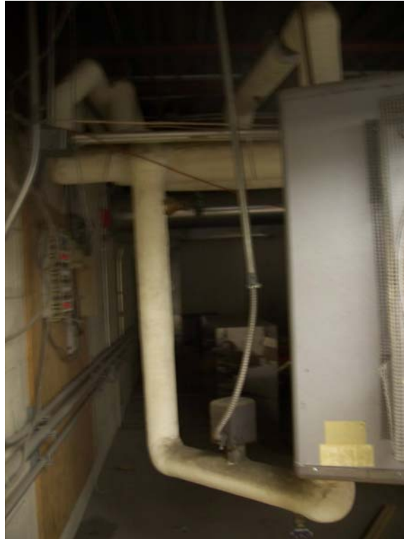
Photograph No. 3 Additional ACM mud elbows on mezzanine
