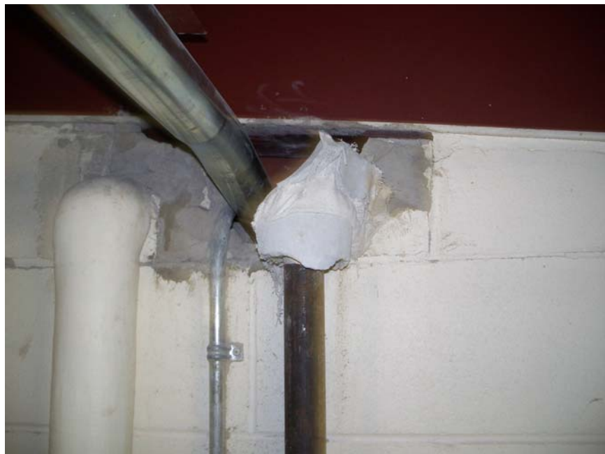
Photograph No. 2 Asbestos-containing mud elbows
