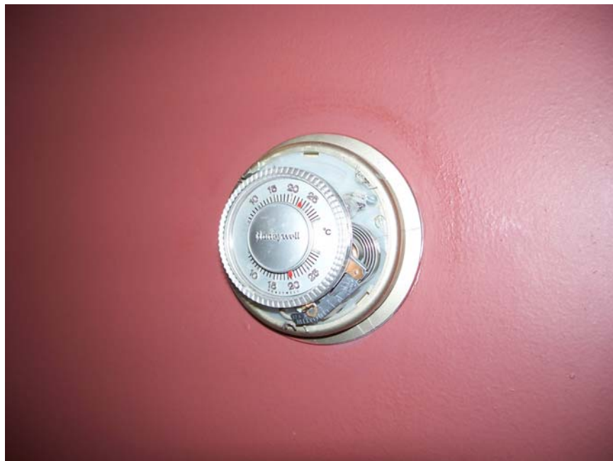
Photograph No. 12 Mercury thermostat identified in offices.
