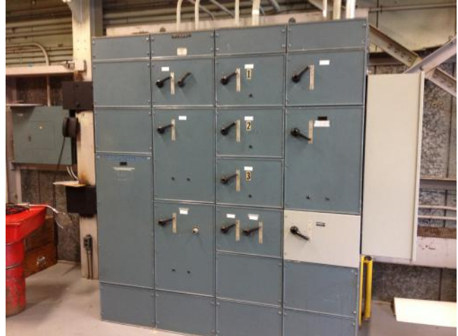
Photograph 6: [North / South Bridge Towers] "MCC" unit to me moved within the mechanical rooms.
