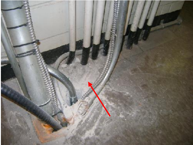
Photograph 1: [Control House Electrical Room - 2 nd Floor] Asbestos-containing grey 9"x9" vinyl floor tile observed to be in fair condition around pipe conduit penetration.
