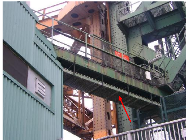
Photograph 4: [Catwalk] Lead-containing green paint application observed to be in poor condition.
