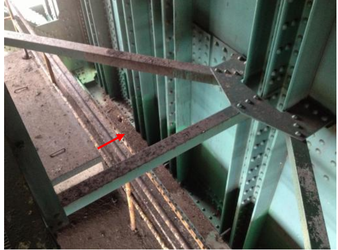
Photograph 10: [Bridge Tower, below Sheave Room] Guano observed on the bridge tower structure.
