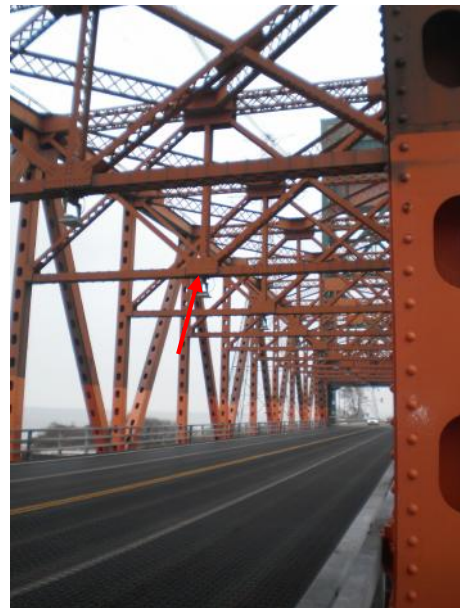
Photograph 8: [Lift Bridge Structure] Lead-containing red primer paint application observed to be in fair condition.
