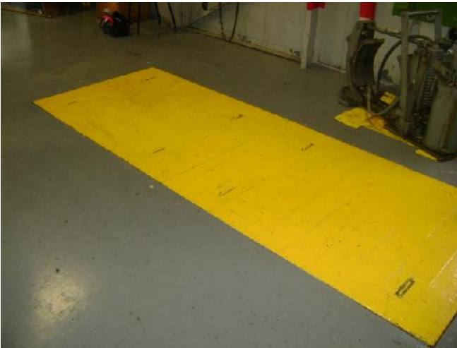
Photograph 7: [North/South Towers Mechanical Room] Lead-containing grey floor paint application observed to be in good condition.
