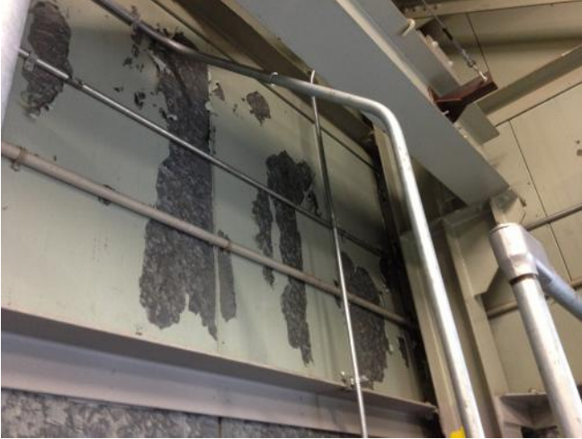
Photograph 5: [North / South Bridge Towers] Lead-containing grey wall paint application in the mechanical room observed to be in poor condition.
