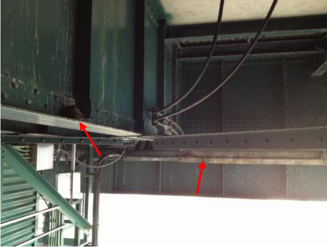
Photograph 9: [Bridge Tower, below Sheave Room] Guano observed on the bridge tower structure.
