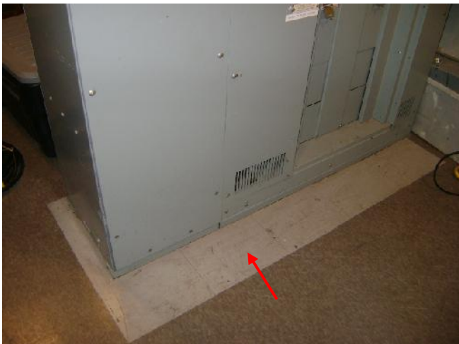
Photograph 3: [Control House Electrical Room - 2 nd Floor] Non-asbestos-containing 12"x12" off-white vinyl floor tile with faint streaks (Sample Set BLB-1).
