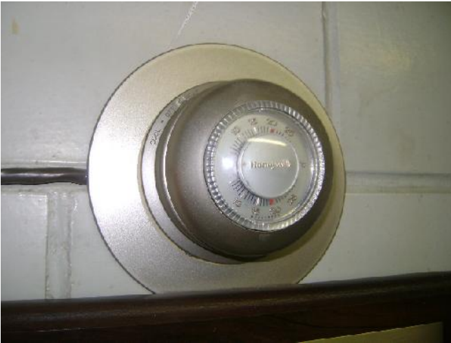
Photograph 11: [Control House – Electrical Room] Mercury-containing thermostat.
