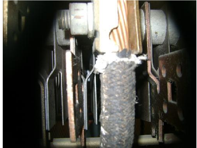
Photograph 2: [Control House Electrical Room (2 nd Floor)] Presumed asbestos-containing electrical cable sheathing observed to be in fair condition.
