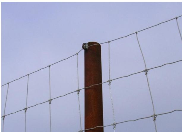
Typical chain link top hook on fence post
