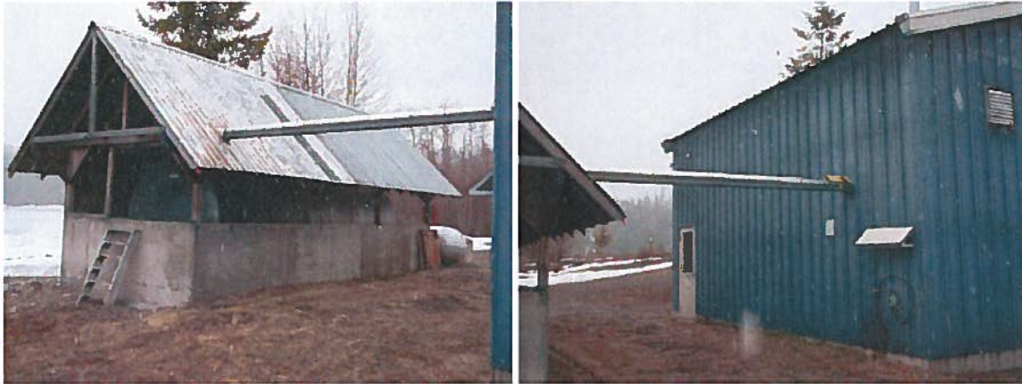
PHOTO 8 & 9: PUMPHOUSE BUILDING AND DIESEL FUEL STORAGE TANK Fuel transfer and Overflow/Vent piping
