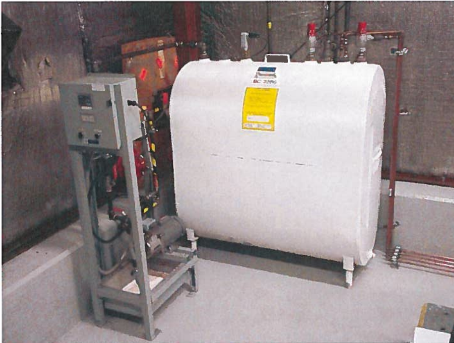
PHOTO 11: PUMPHOUSE BUILDING AND DIESEL AUXILIARY (DAY) TANK Fuel transfer pump and controls
