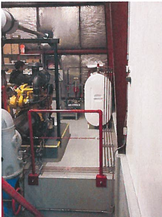
PHOTOS 12: PUMPHOUSE BUILDING AND DIESEL AUXILIARY (DAY) TANK Engine fuel supply and return piping
