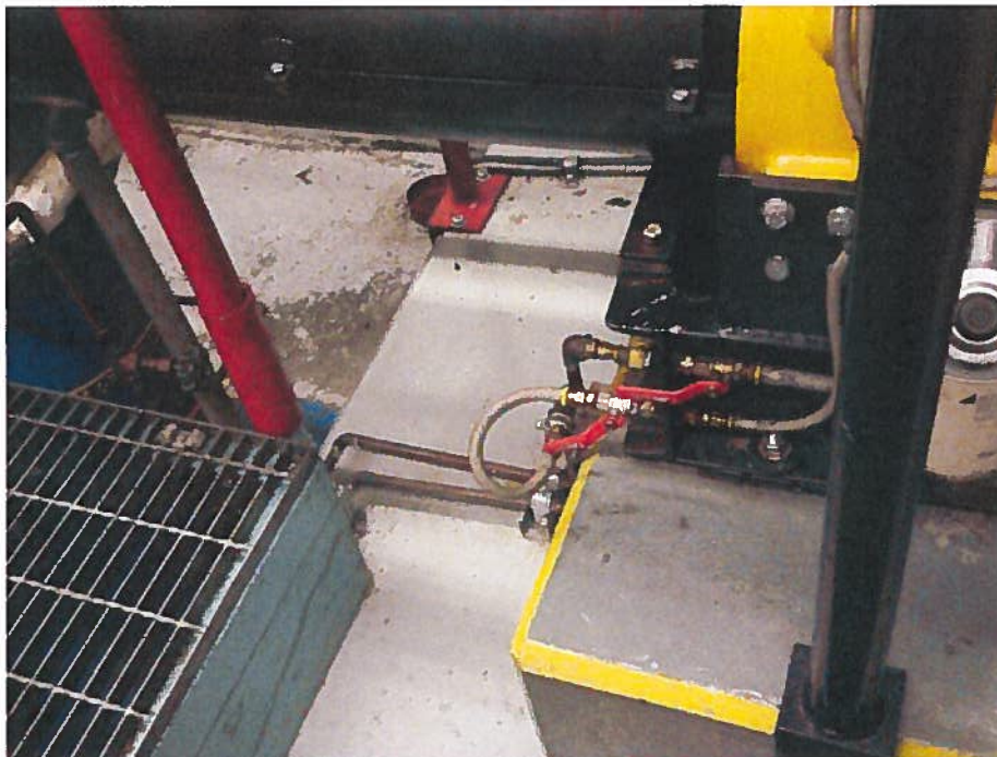
PHOTOS 14: PUMPHOUSE BUILDING Engine fuel supply and return piping, and engine fuel hose connections
