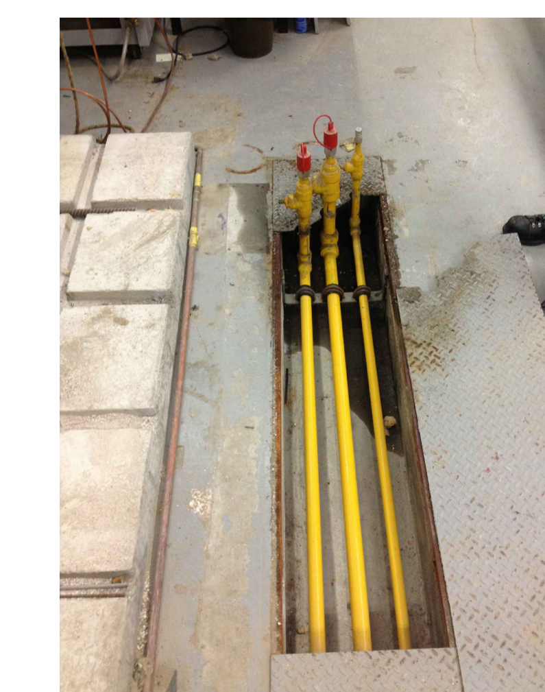
3 G02 BUILDING M-20- BASEMENT- ROOM 007 PHOTO- PIPING TO BE REMOVED FROM TRENCH SCALE: N/A
