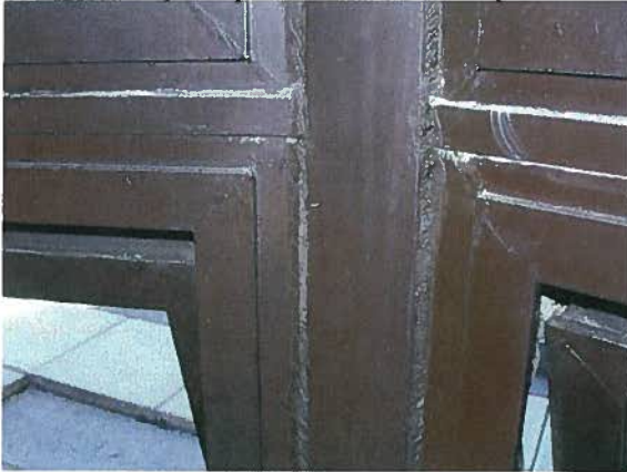
Photo 1: Brown Interior Window Mastic (0.75% chrysotile)
