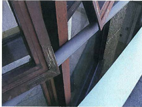
Photo 5: Reddish Brown Paint (assumed to be lead containing)
