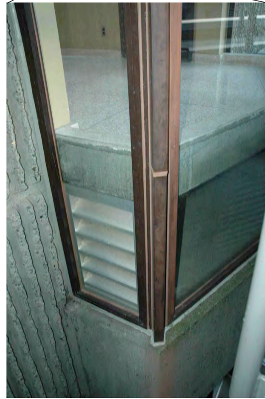
(E) INTAKE GRILL
