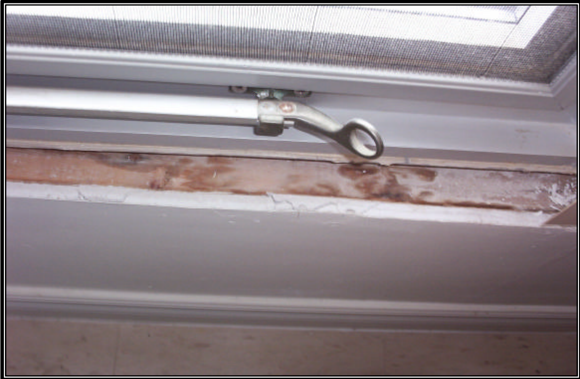
Photo 3: View of water damage on living room window ledge of dwelling Unit E8.
