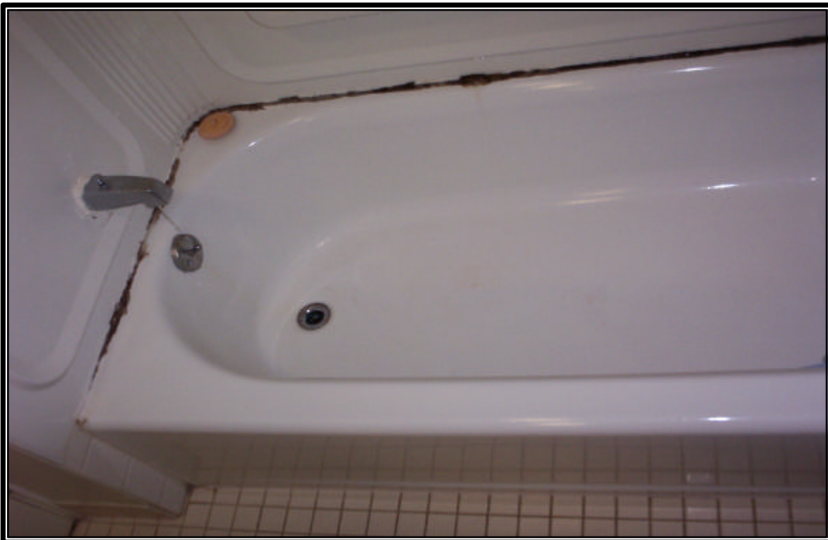
Photo 4:View of dark staining suspected of being mold in the bathroom (108) of Dwelling Unit E7.
