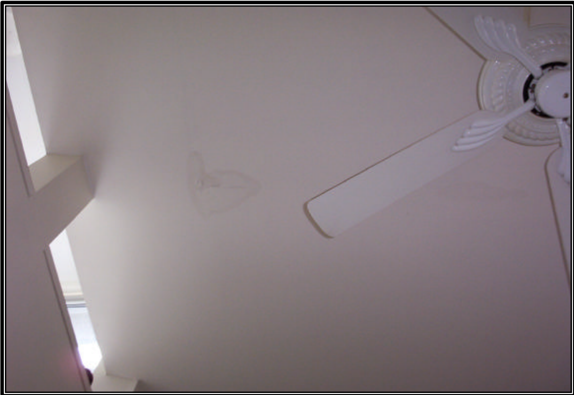
Photo 2: View of water damage on living room ceiling of Dwelling Unit E1.
