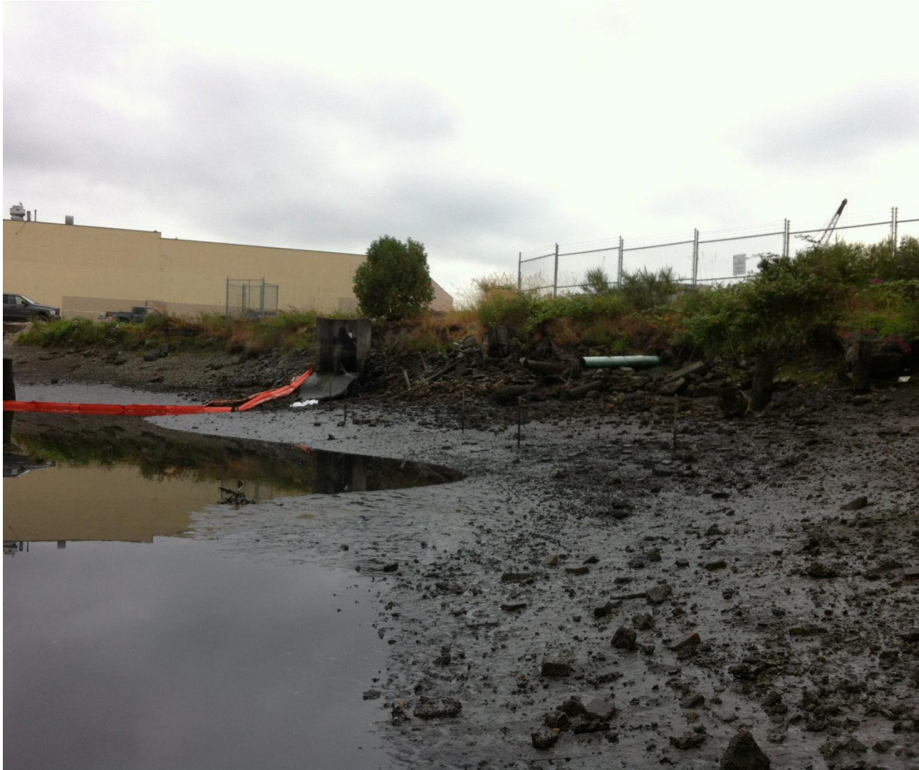
Photo 12: Looking east, along the south shoreline of Rock Bay. Outfall 626 with tidegate shown in centre of photo.
