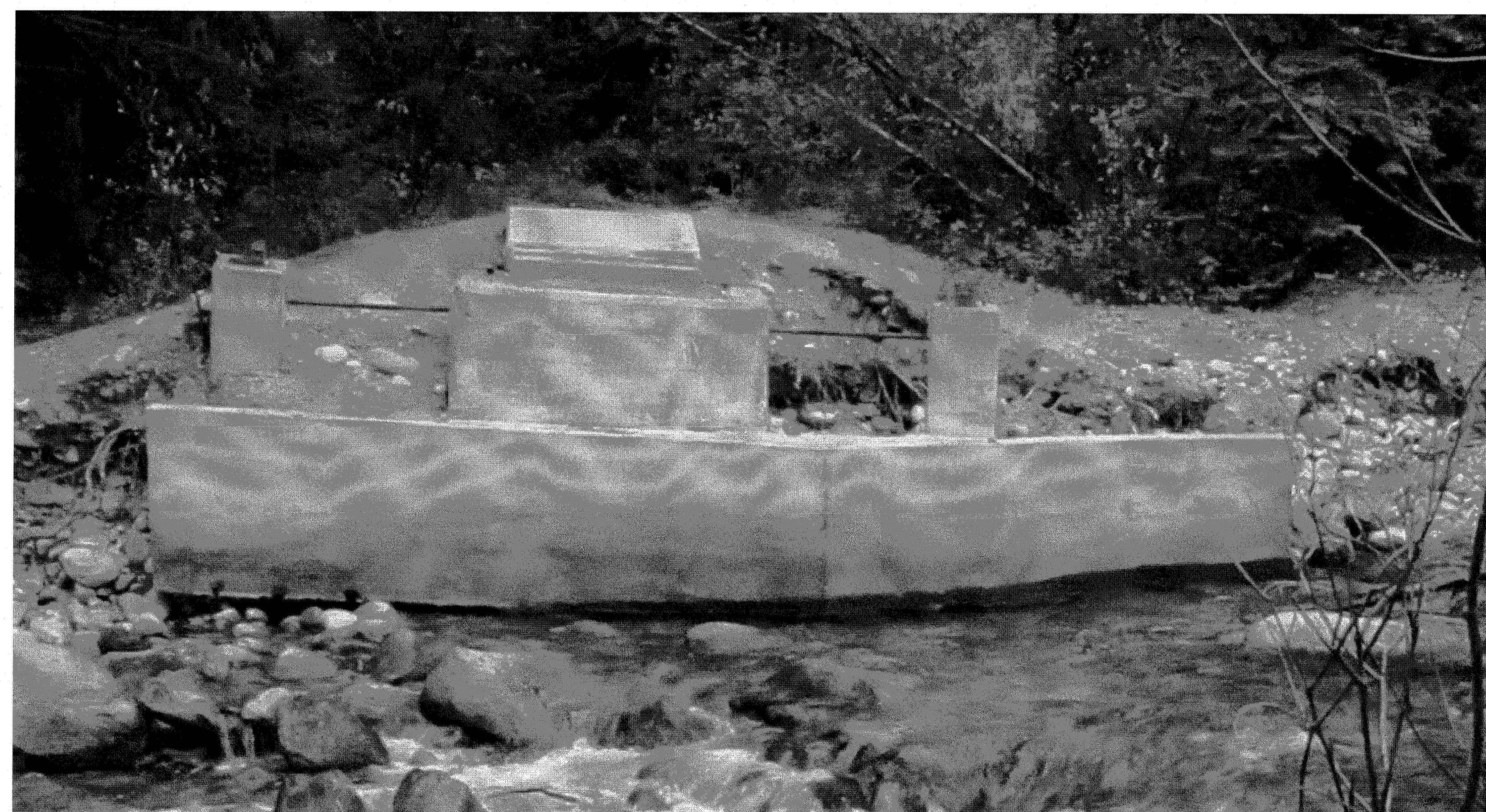
NOTE: PHOTO SHOWS FRONT ELEVATION OF NORTH BANK CONCRETE FOUNDATION THAT IS TO BE REMOVED AND DISPOSED
