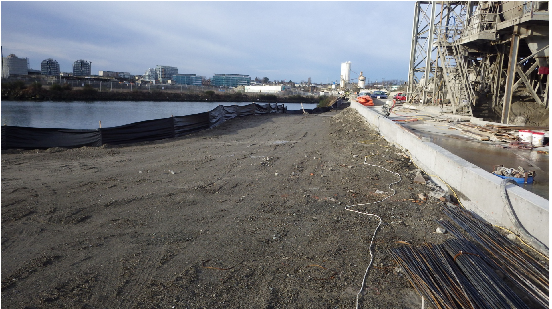
Photo 7: Looking west along the upland area north of Rock Bay (part of South Excavation Area).
