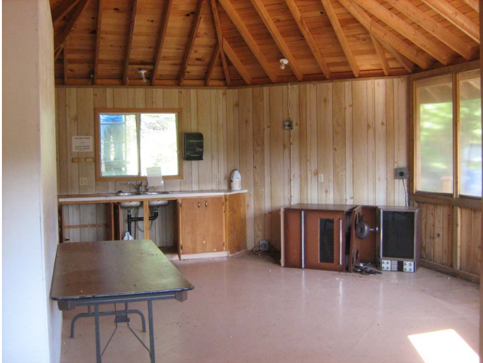
PHOTO No. 7: Cavendish Canteen – Kitchen – north portion of building with handicap washroom.
