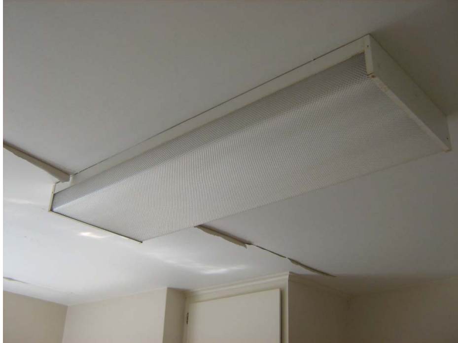
PHOTO No. 50: Asset No. 108 – Fluorescent light (potential PCB/mercury containing).
