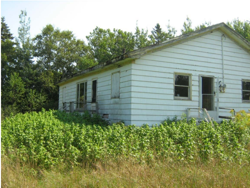
PHOTO No. 29: Asset No. 112 - Sheppard Cottage – Staff House – view from northwest (Asbestos containing siding).
