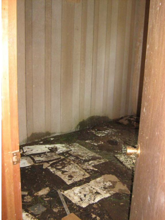
PHOTO No. 34: Asset No. 112 – Bedroom Floor – carpet, ceiling tiles and mold.
