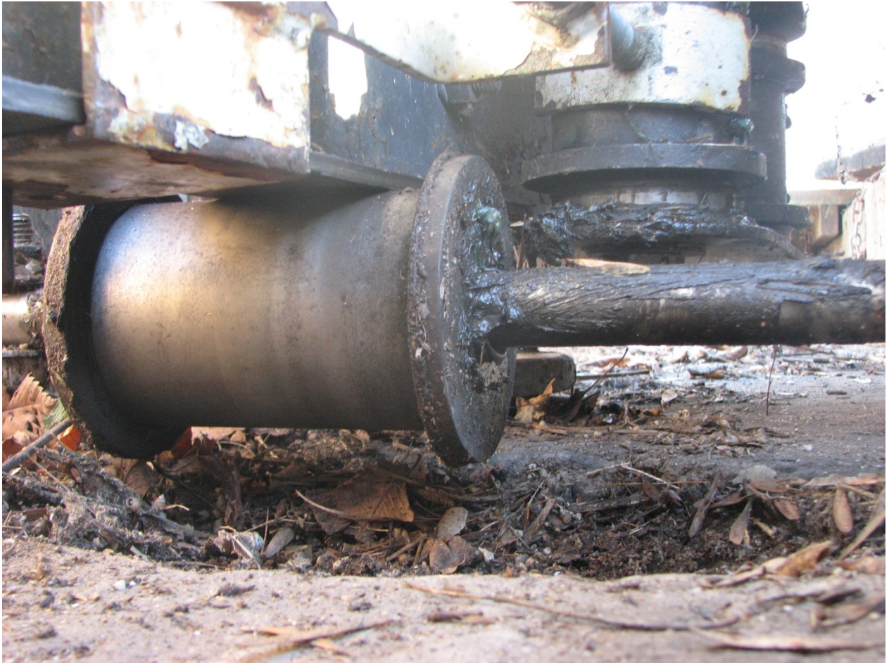
A18- Rack support roller (right bank)
