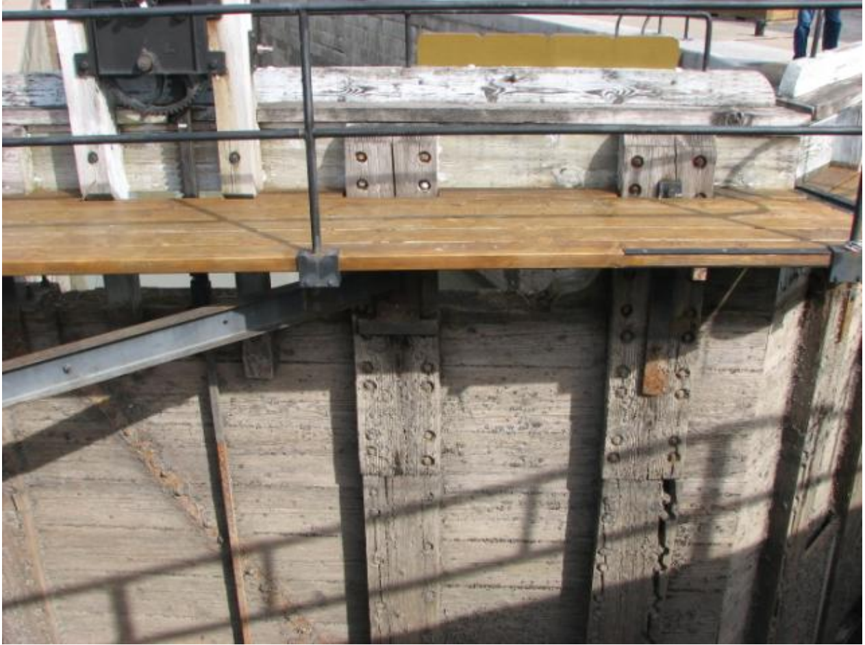
A7 –Rack of the left bank gate
