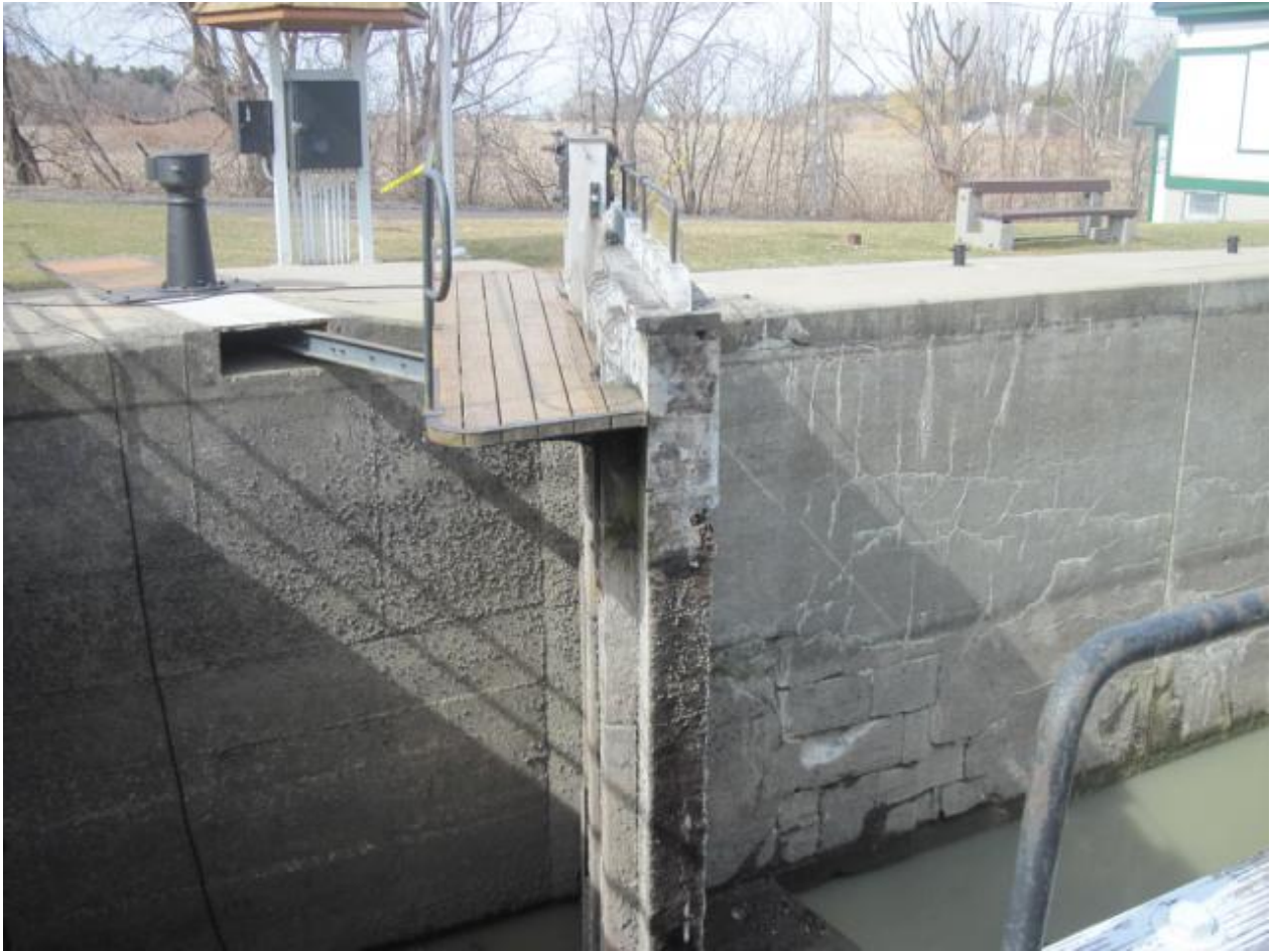
A6 – Left gate opening mechanism
