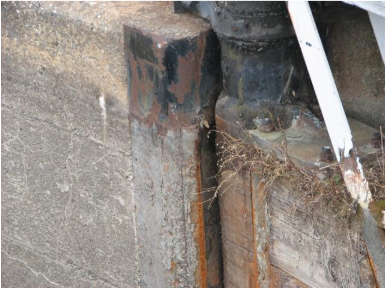
A10 – Upper pivot of right gate
