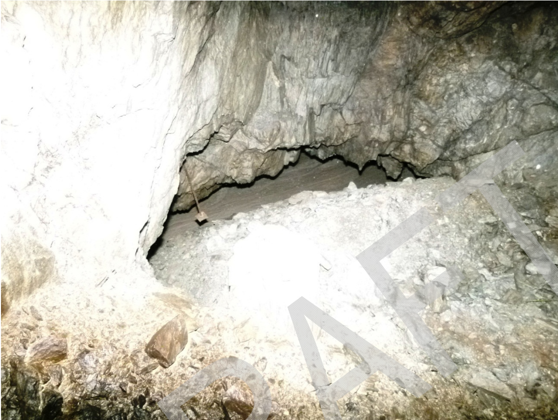
Photograph 1: Partially backfilled connection between voids – example of leakage point that was plugged
