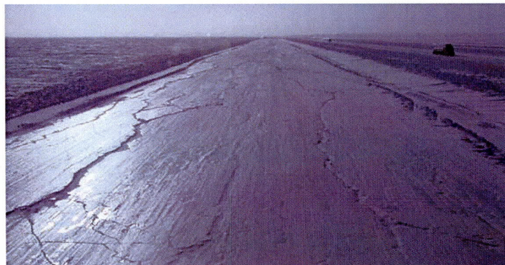
Figure 8 Normal longitudinal cracking caused by buoyancy of the thickened ice over the 20-metre wide travel lane
