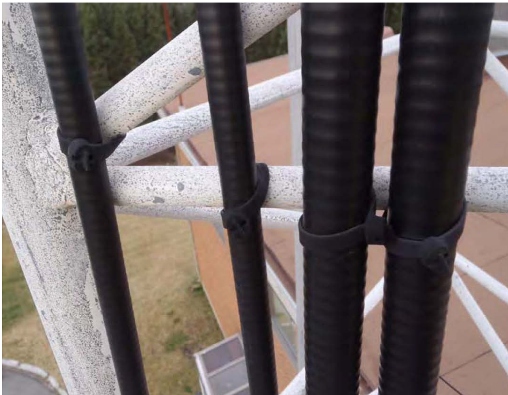
Photo 6 – Tx-lines nylon/vinyl tie wraps
