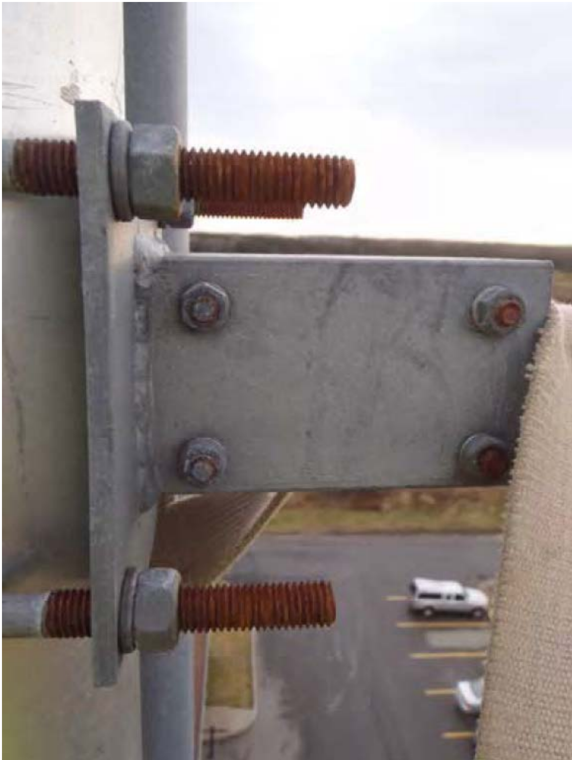
Photo 4 – Corroded 210C-4 Mounting hardware
