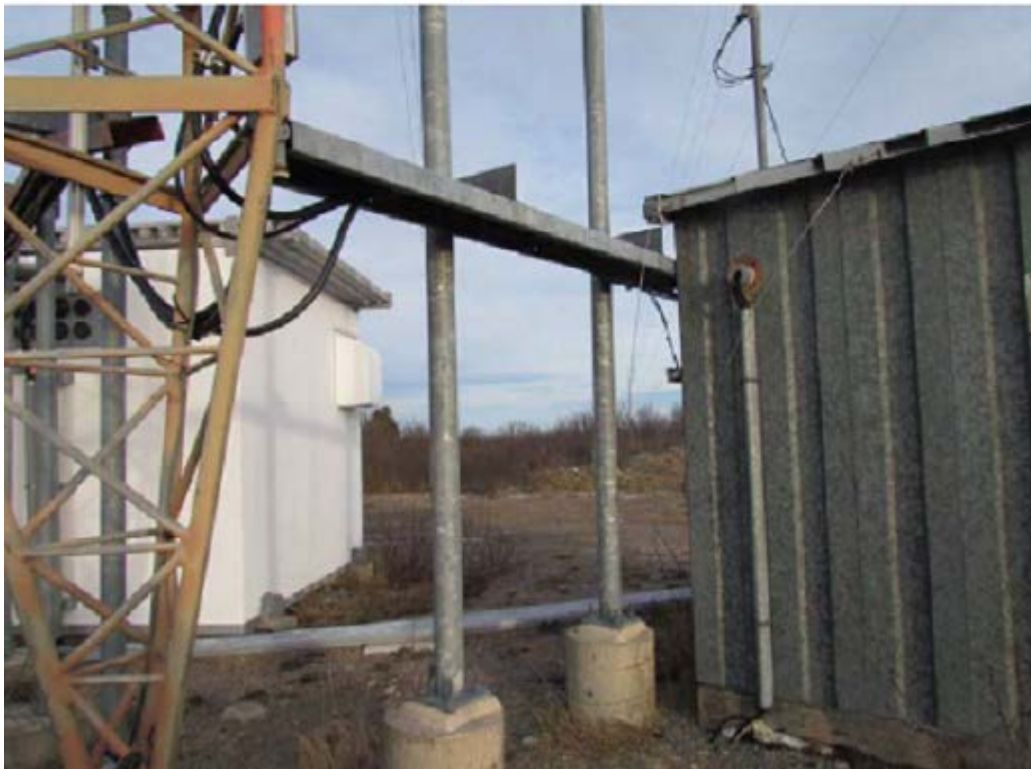
Photo 11 – Wave Guide Bridge RCMP Shelter
