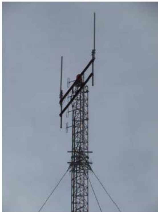
4 Antenna Configuration from anchor 1
