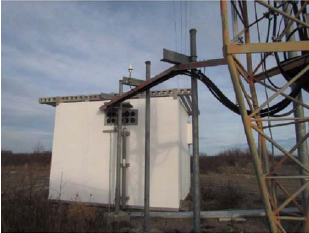
Photo 10 - Waveguide Bridge Bell Shelter
