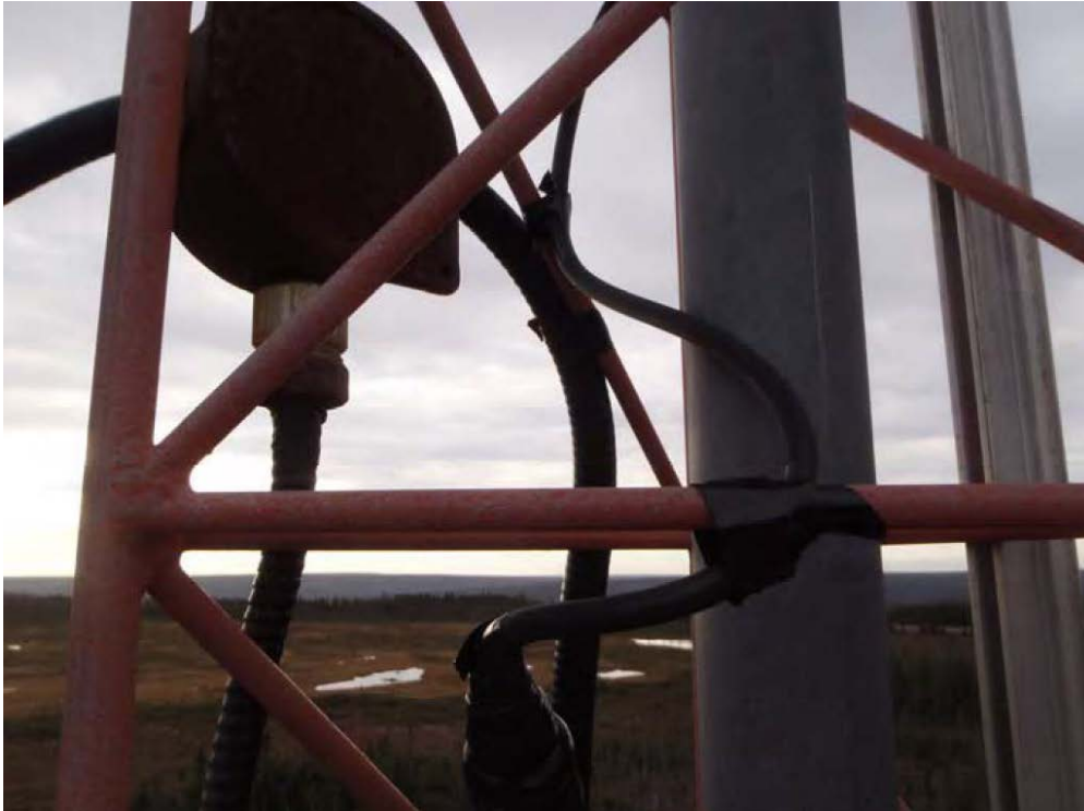
Photo 5 – Tx-line taped to tower
