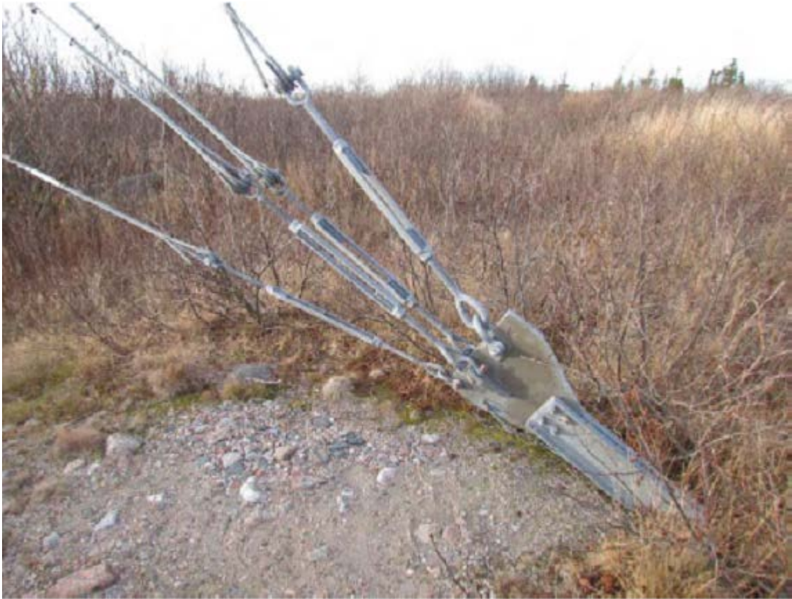
Photo 9 - Typical Guy Anchor
