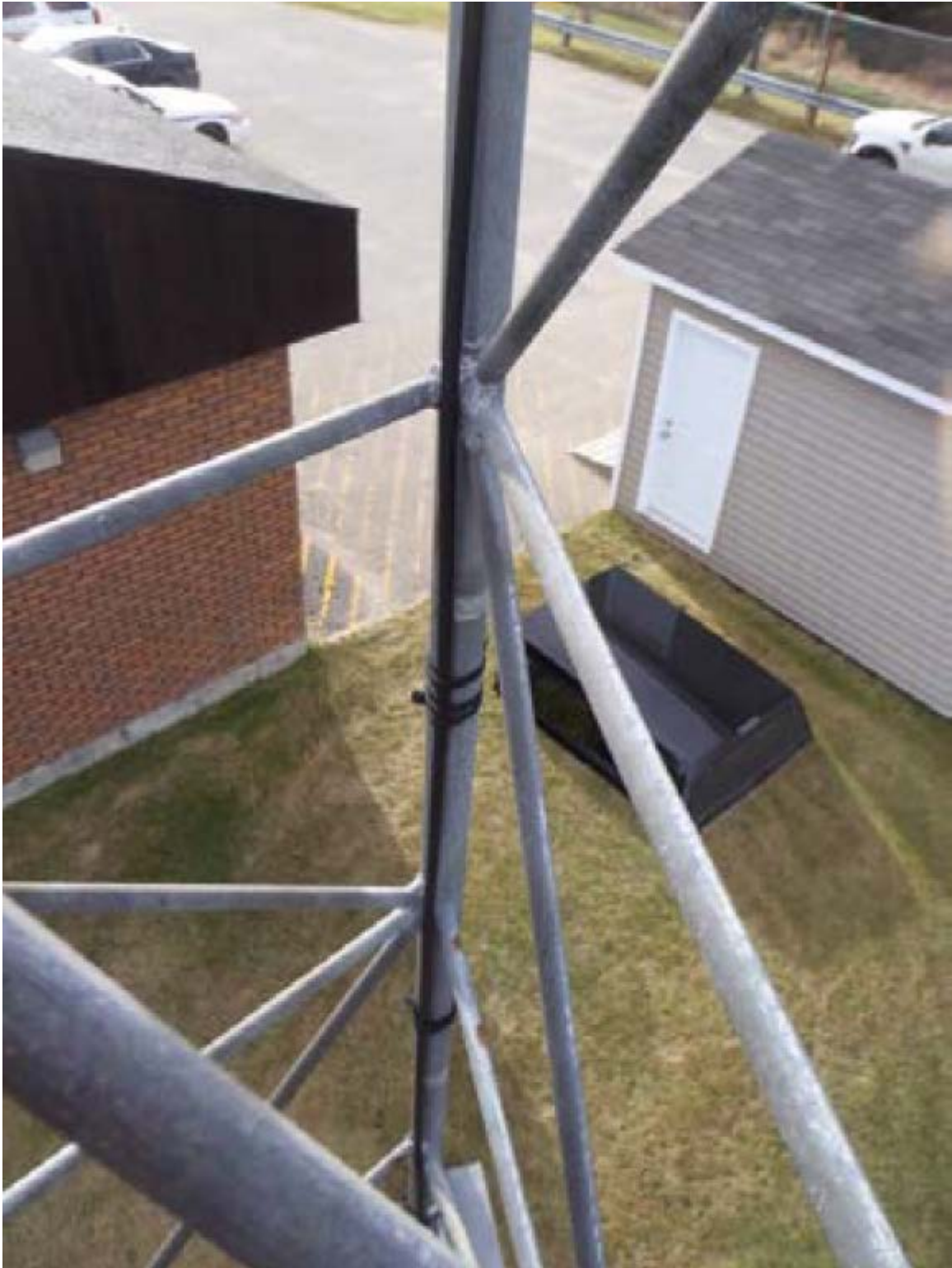
Photo 2 – Tx-lines vinyl tie wraps
