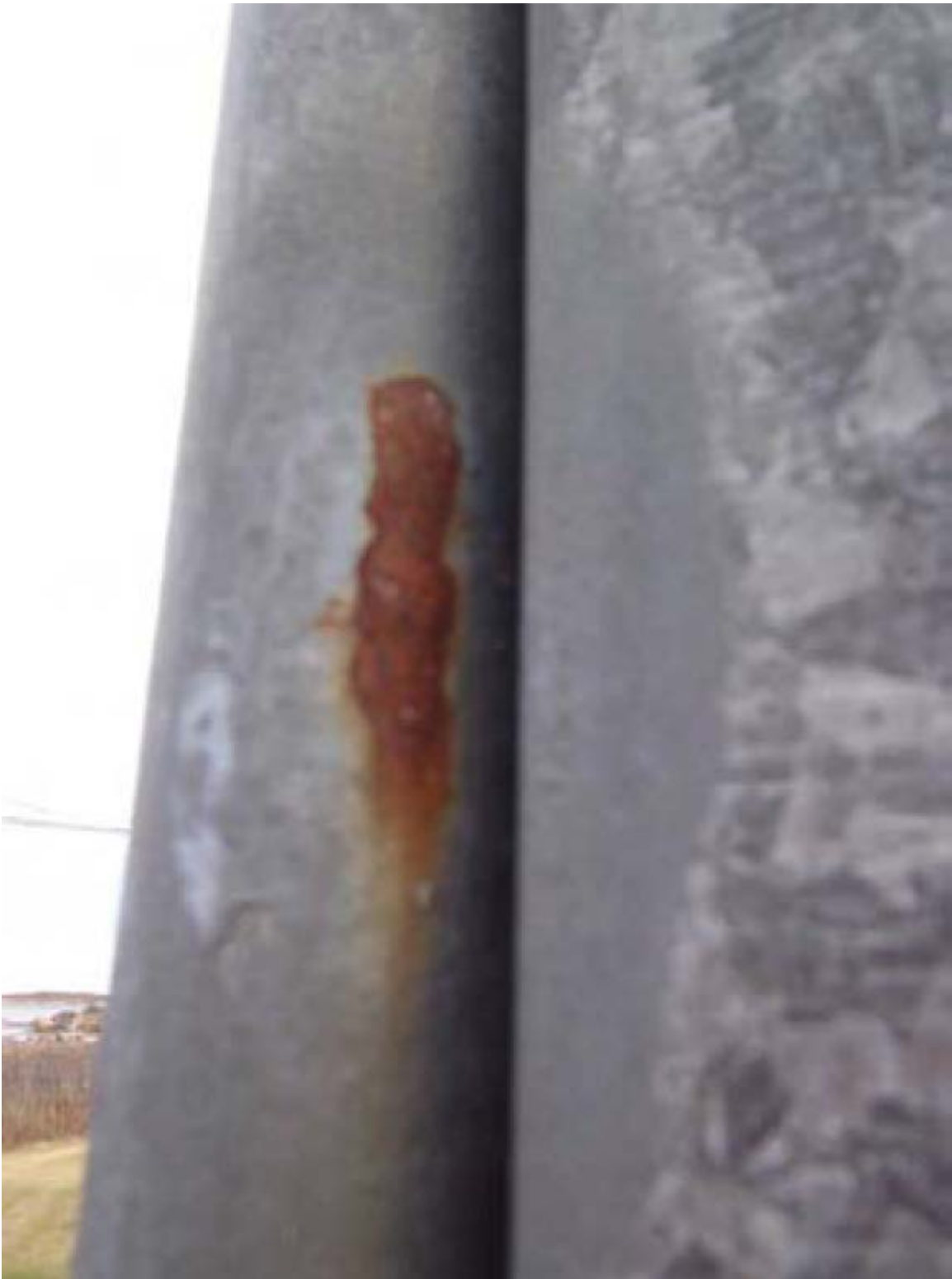
Photo 3: Tower member corrosion
