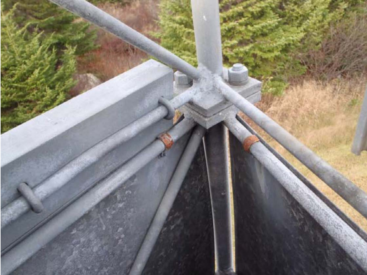
Photo 4 – Anti-climb corroded clamps
