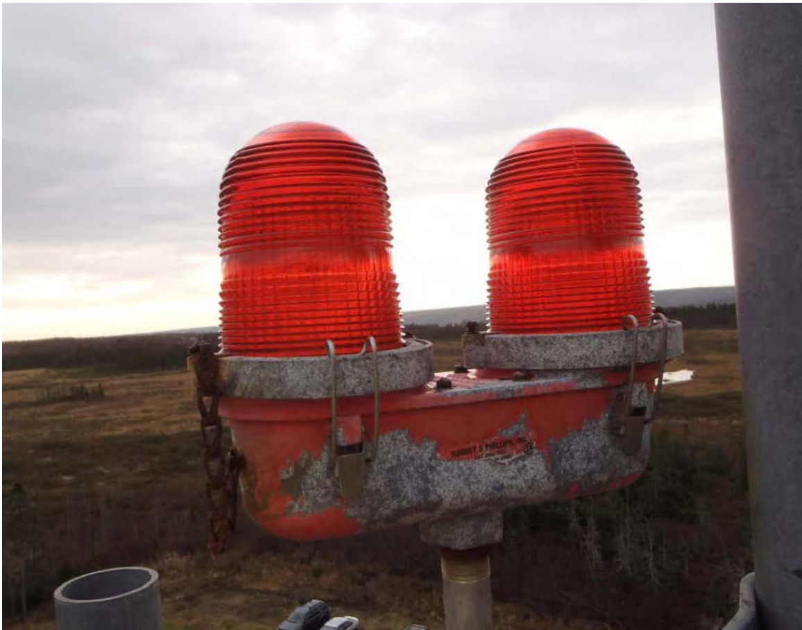
Photo 12 – Tower lights not working
