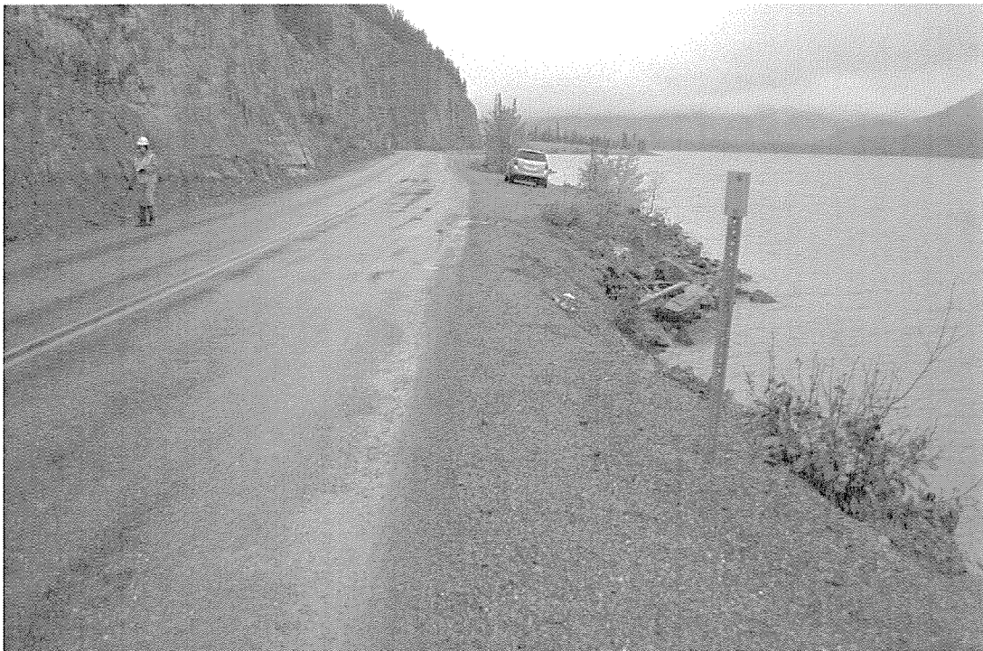
Photo 2: Looking South at Highway Shoulder above Existing Gabions between Stn. 701+628 and Stn. 701+646.
