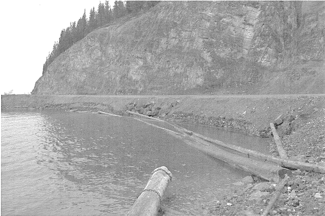
Photo 1: Looking North at Existing Gabions, Riprap, and Logs between Stn. 703+082 and Stn. 703+097.
