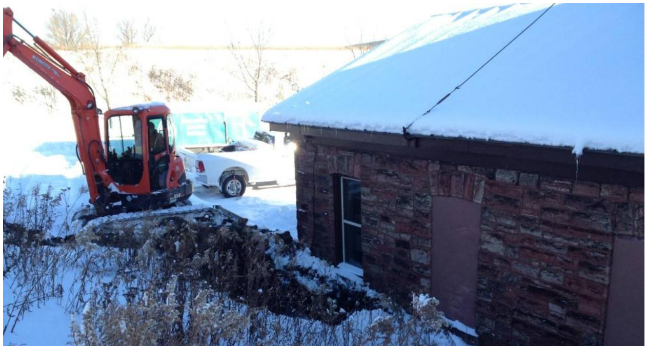
Photo 2: View of TP13-03 excavated at northwest corner of the building. The northern portion of the building does not appear to be moving, so this test pit was for comparative purposes.
