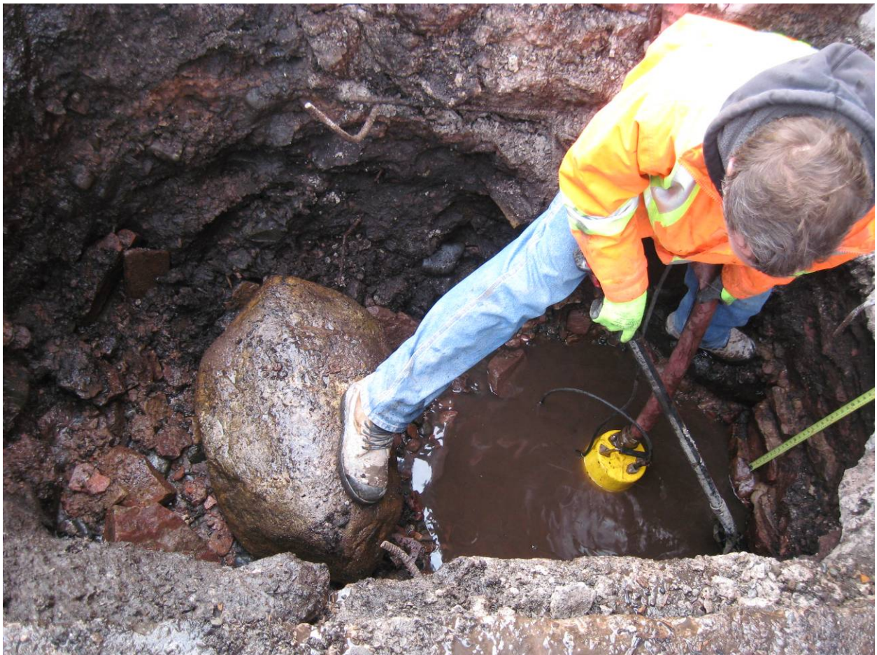
Photo 1: View of TP13-01. Poor quality fill, foundation wall to the right and infiltrating groundwater.
