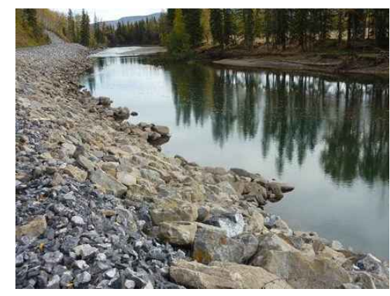
"SCALLOP" RIP RAP WITH SELECT LARGE ROCKS APPROX. 2m PROTRUSION 20m ± SPACING TO ELEV. 961.5m
