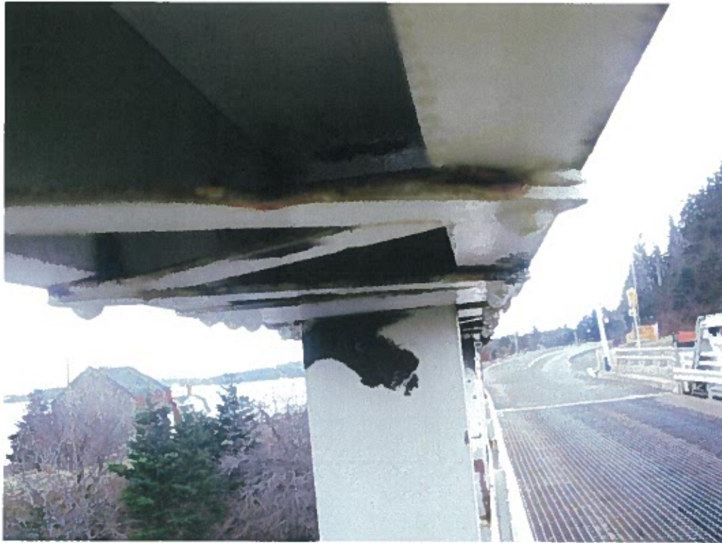
Photograph 3 – Lacing bars along top chord at north truss. Note: Section loss in lacing bars.
