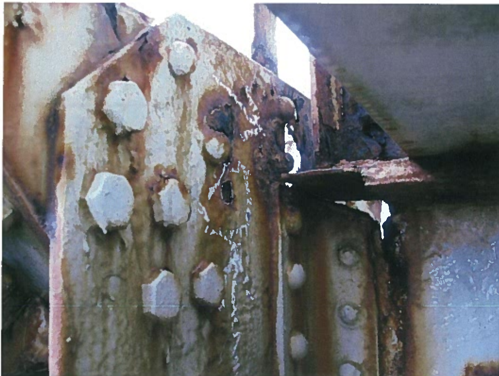
Photograph 16 - Section loss and perforation at gusset plate location at north truss panel point 2W
