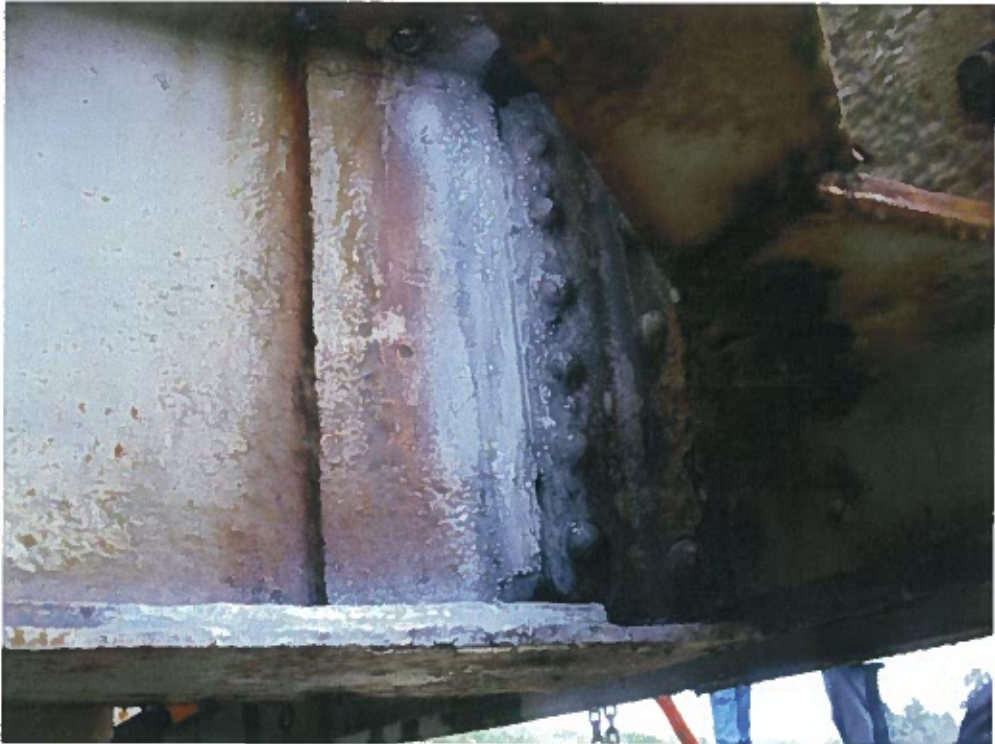
Photograph 47 – Magnetic particle testing of welded reinforcement at the web of the floor beam to the connection angle at panel point 2W.
