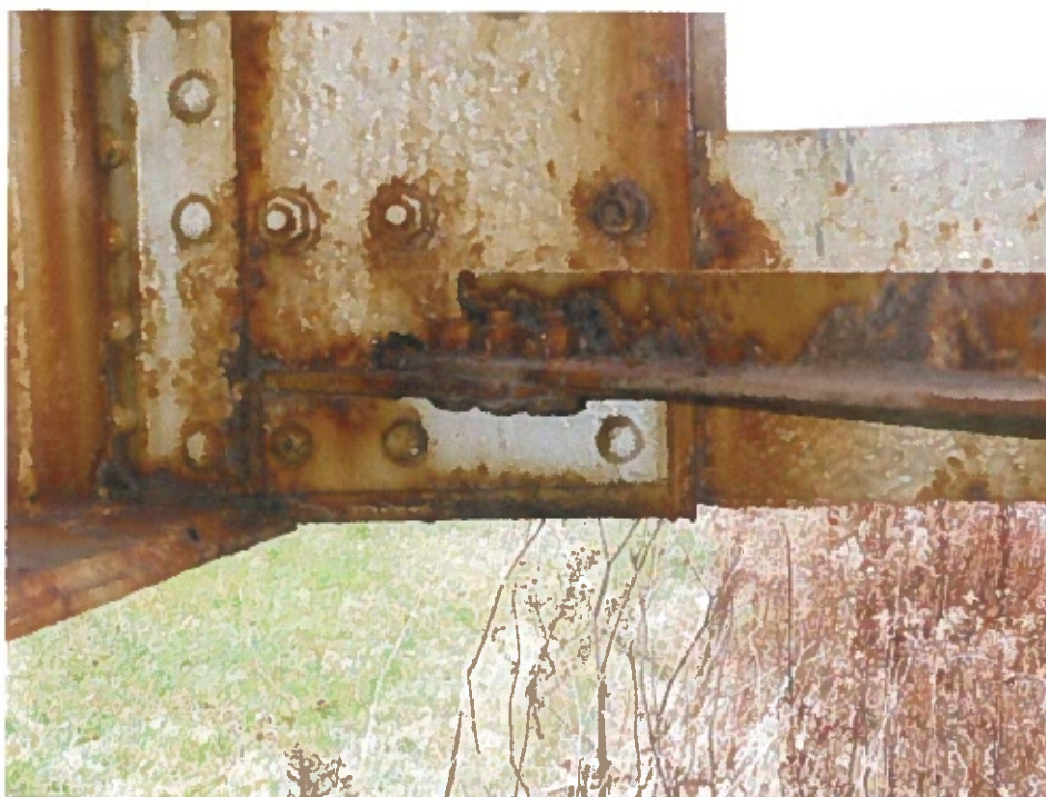
Photograph 35 – Typical condition of horizontal bracing at panel point connection. Note: Medium to severe corrosion.
