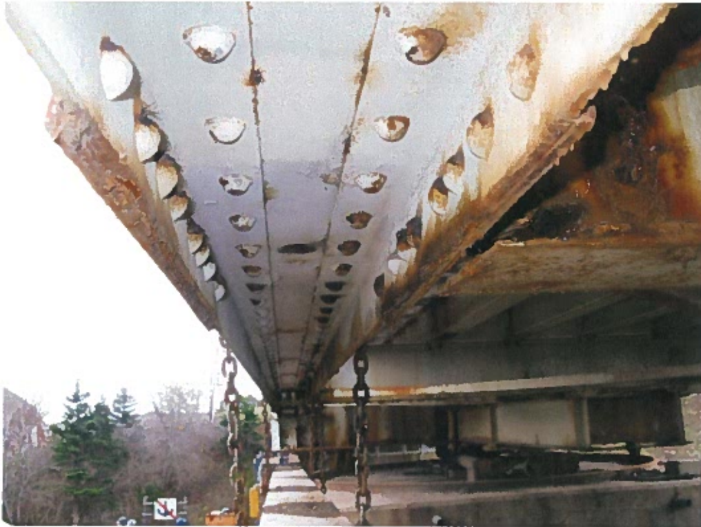
Photograph 9 – Condition of bottom chord along north truss. Note: Medium to severe corrosion.
