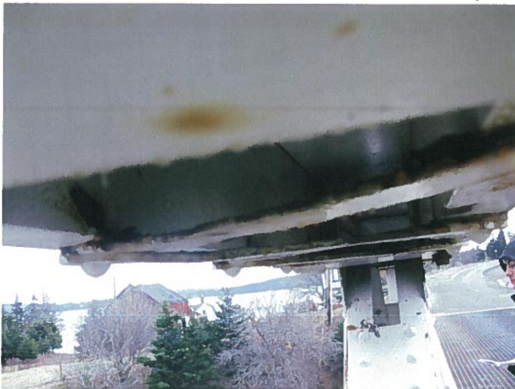
Photograph 4 – Lacing bars along top chord at north truss. Note: Section loss in lacing bars.
