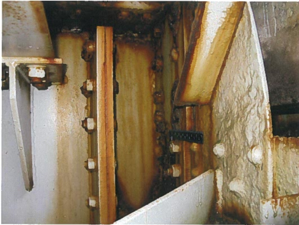
Photograph 17 – Section loss and perforation at gusset plate (panel point 0) at north truss.
