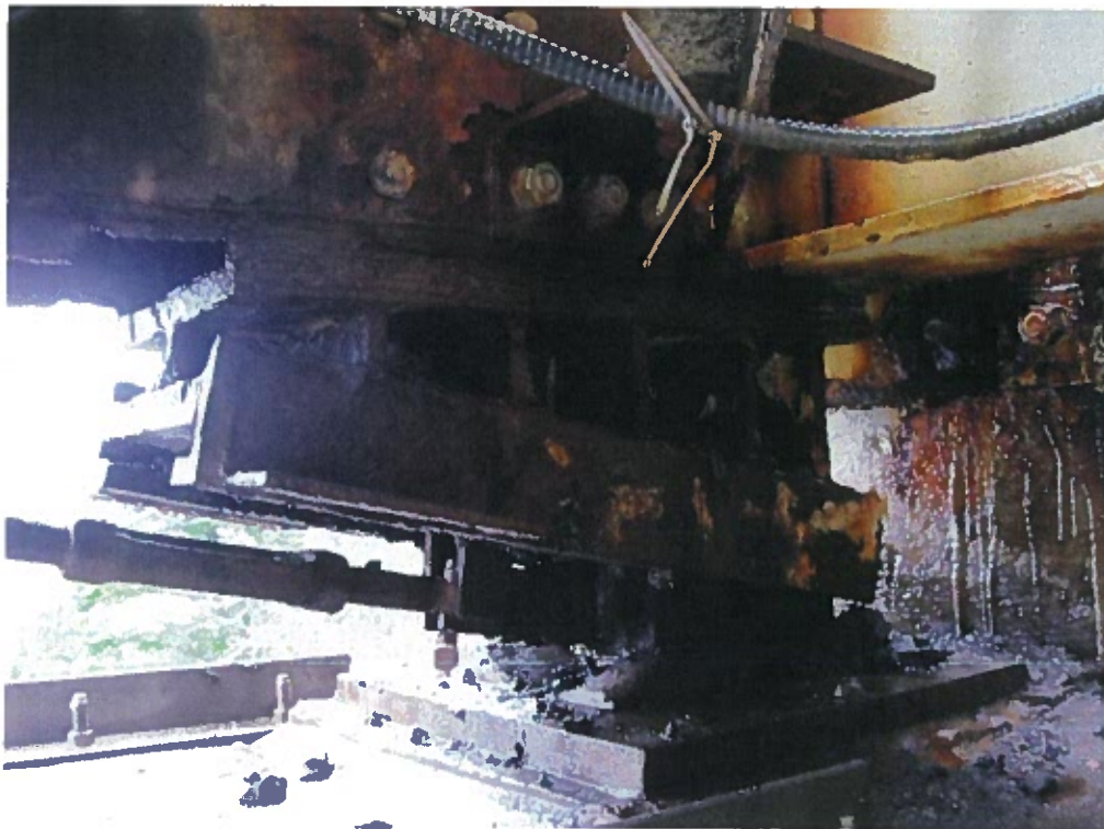
Photograph 2 – North east wedge, note locating feature in wedge and wedge receiver.
