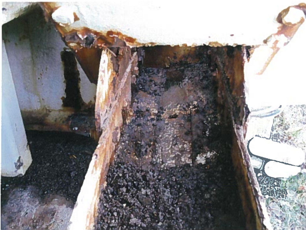
Photograph 12 – Perforation at north truss bottom chord at panel point 3W.
