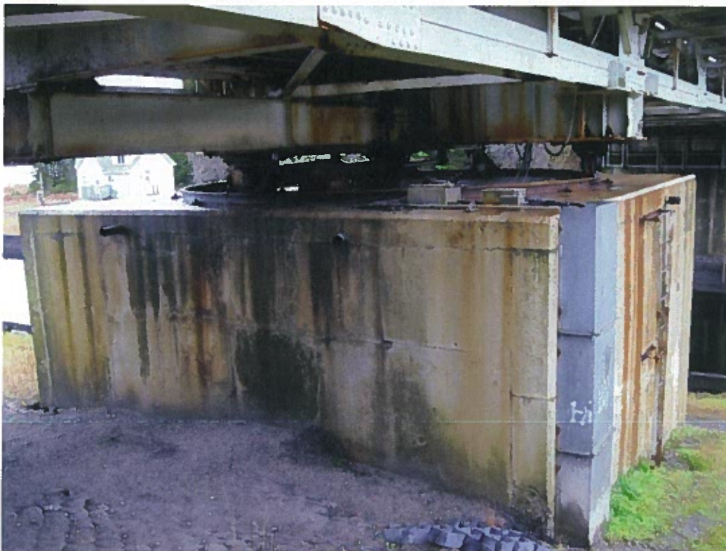
Photograph 8 – Center bearing oil drain line (pipe on the left side)
