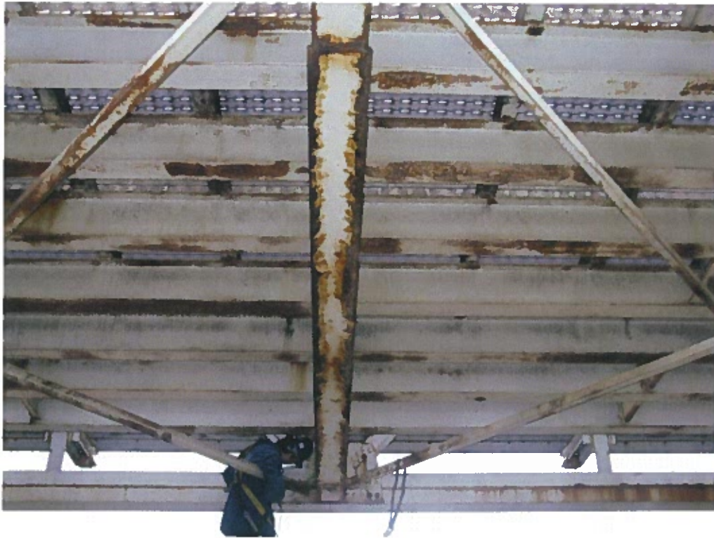
Photograph 31 – Typical condition of floor beams. Note: Welded reinforcement at the bottom flange.
