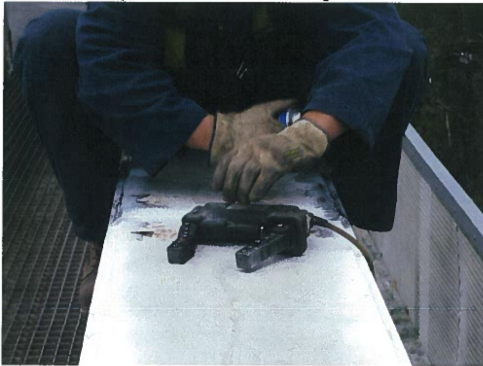
Photograph 40 – Magnetic particle testing of welded reinforcement at south truss top chord between panel points 1E and 3E
