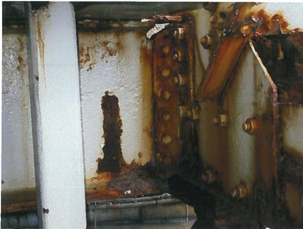
Photograph 32 – Typical condition of connection angles of the floor beam to the lower chord.
