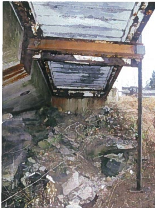
Photograph 38 – Welded reinforcement to existing transverse steel member at the sidewalk near the east abutment.
