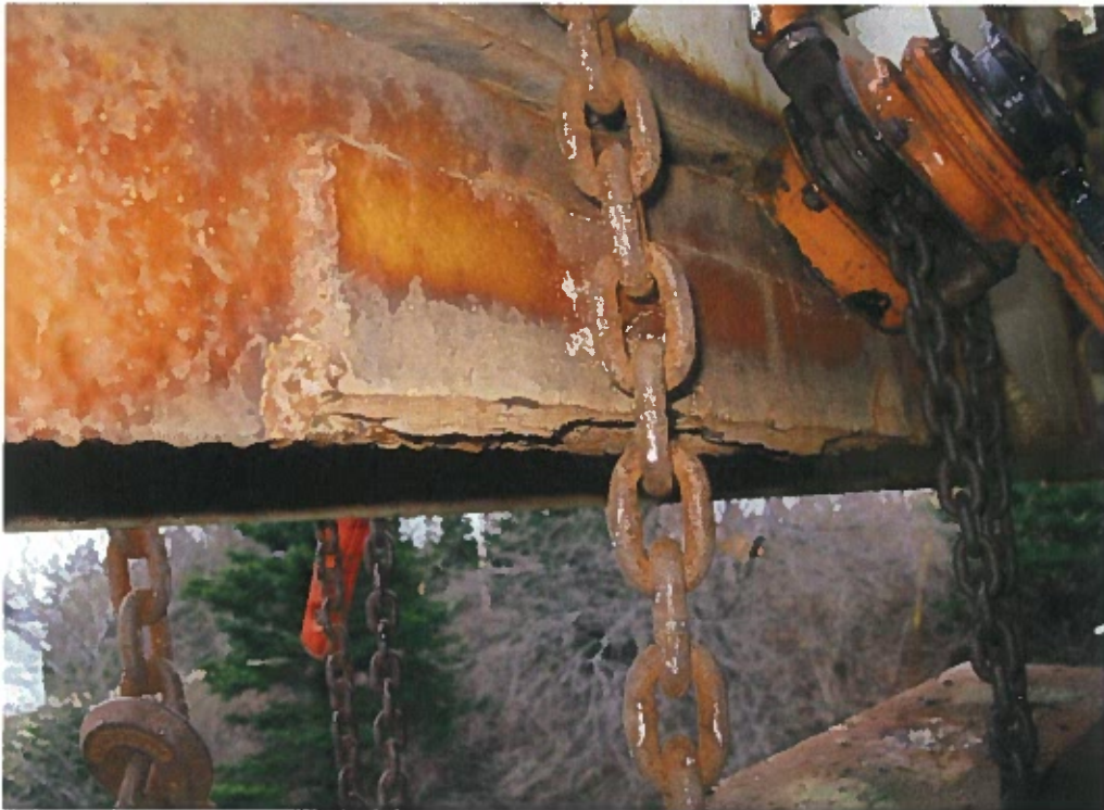
Photograph 19 – Welded reinforcements along north truss bottom chord (between panel points 3E and 4E).
