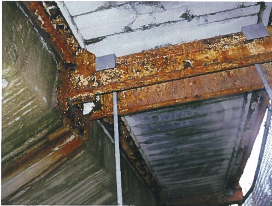
Photograph 37 – Typical condition of structural steel at sidewalk overhang at east approach. Note: Medium to severe corrosion
