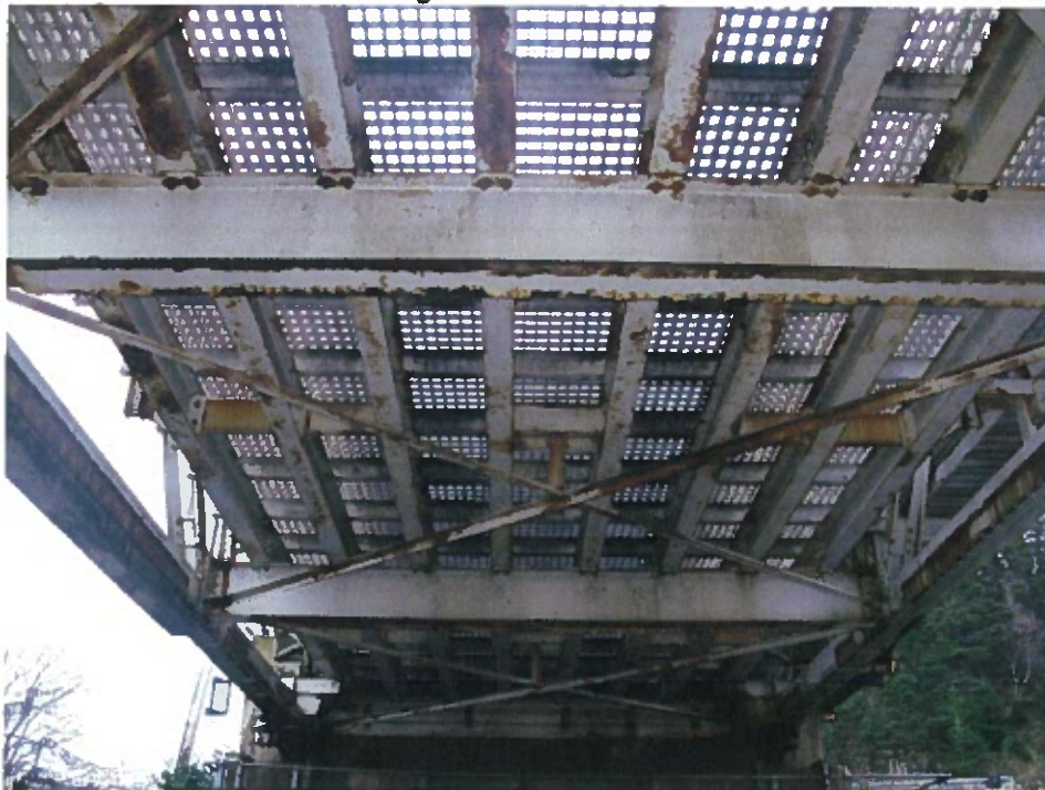
Photograph 30 – Typical condition of stringer/deck beams and grating. Note: the welded reinforcement to the bottom flange of the floor beam.
