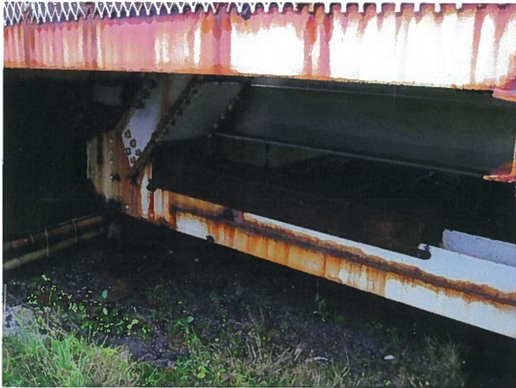
Photograph 17 – Counterweight box for steel counterweights for fine adjustment
