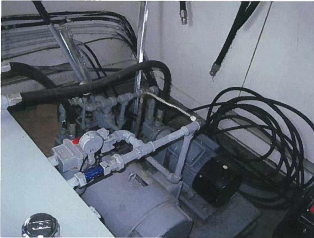
Photograph 9 – Hydraulic power unit 1
