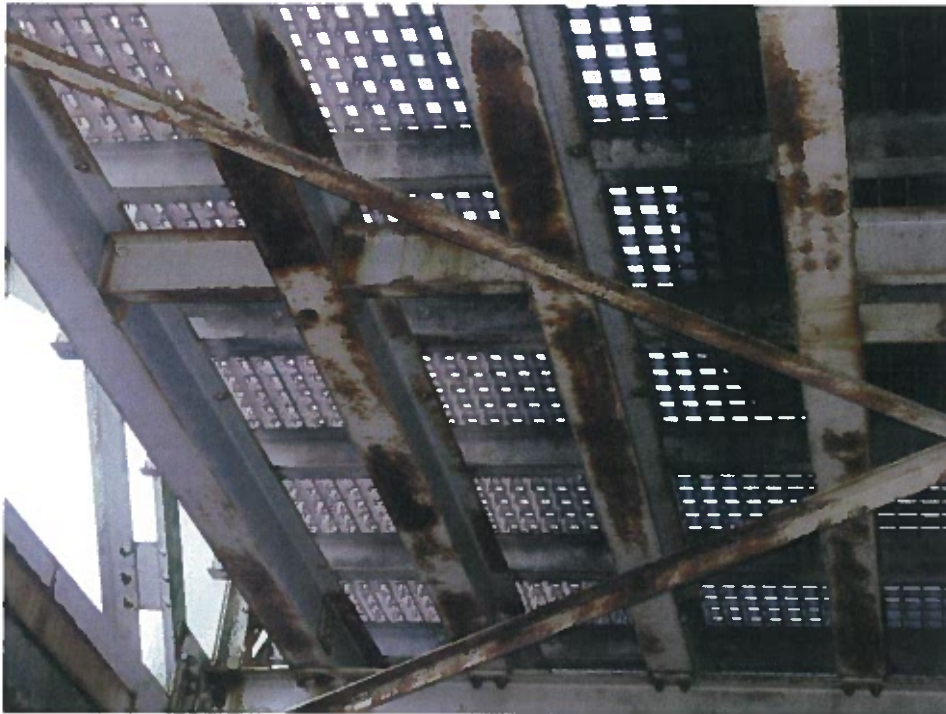
Photograph 29 – Typical condition of stringer/decking beams and grating. Note: coating break down and light to medium corrosion.
