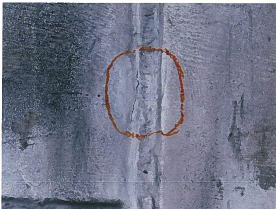
Photograph 44 – Crack in weld at welded reinforcement at panel point 5E south truss bottom chord.
