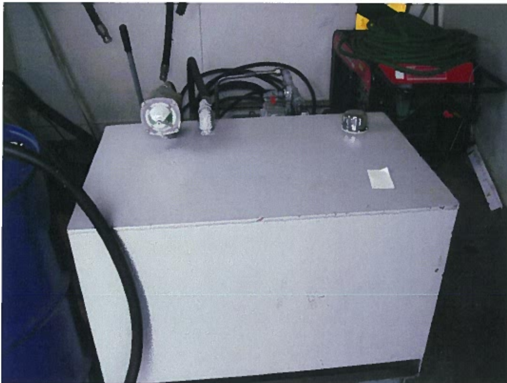
Photograph 10 – Hydraulic power unit 2
