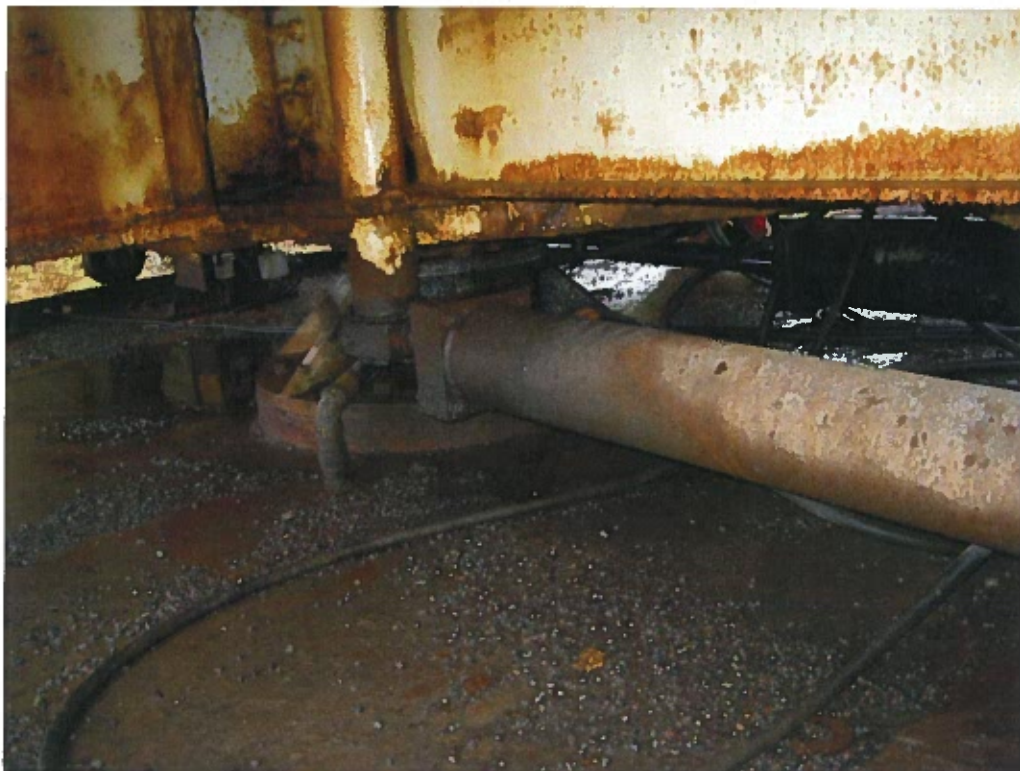
Photograph 6 – South slewing cylinder
