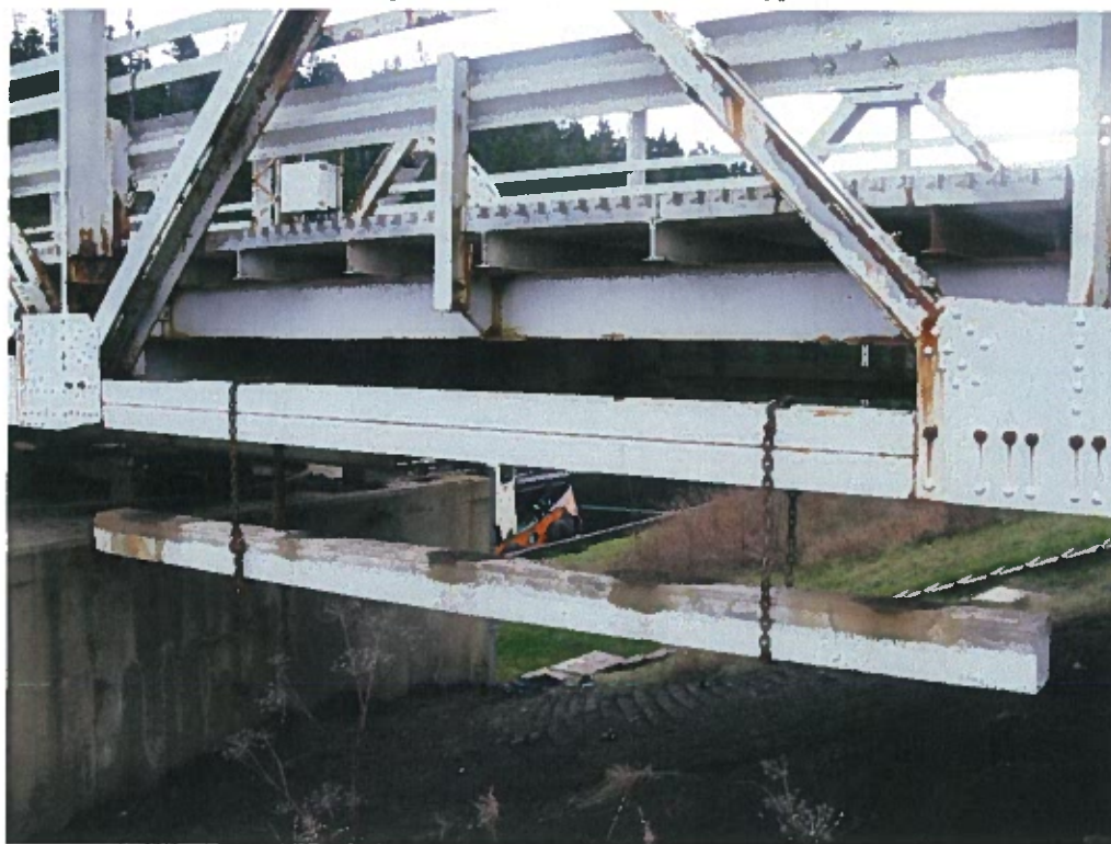
Photograph 8 – Lowering of concrete counter weights along north truss (typ.).
