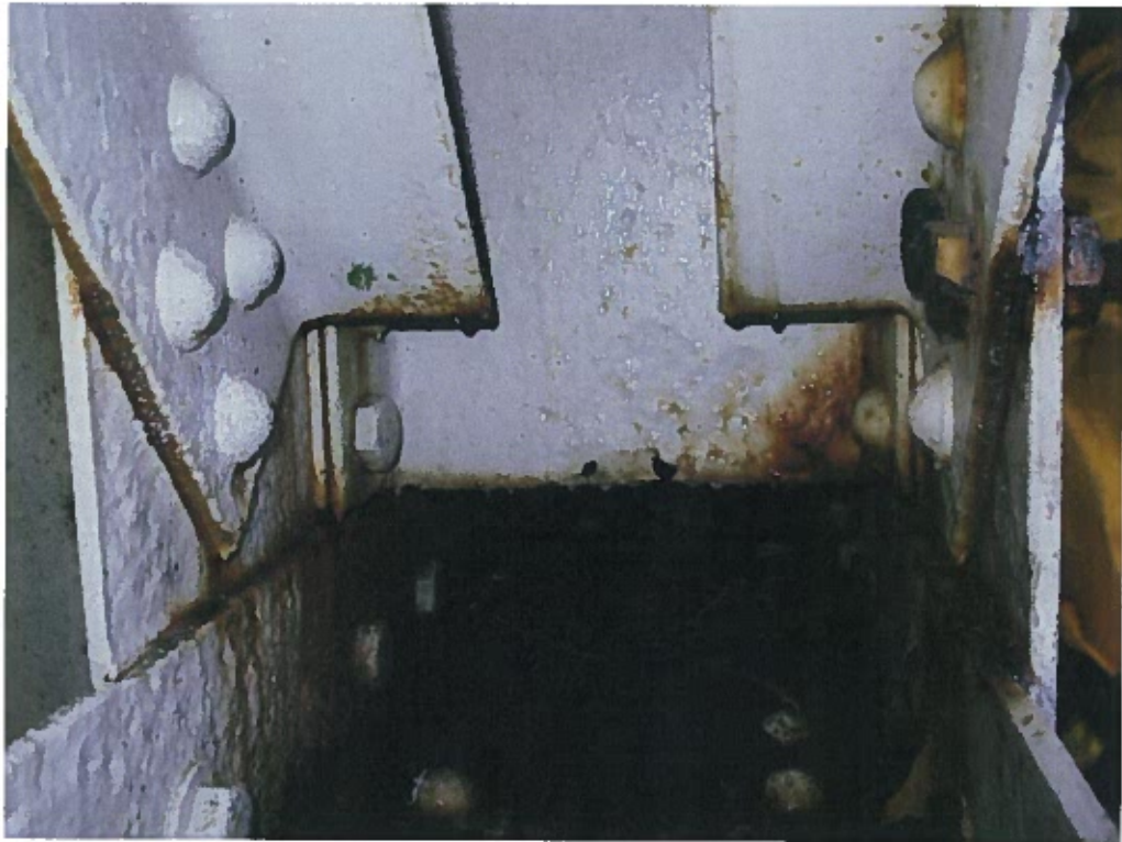
Photograph 23 – Perforation and section loss at vertical member at panel point 4E on south truss.
