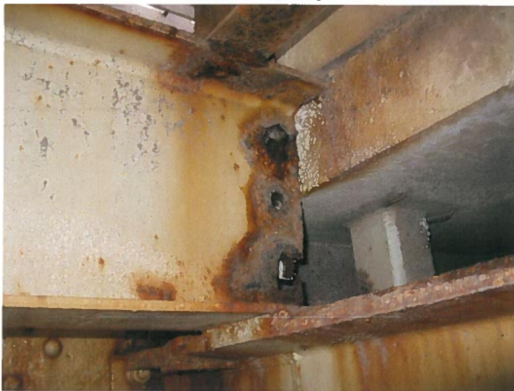
Photograph 28 – Perforation and section loss at stringer S8 between panel points 2W and 3W.
