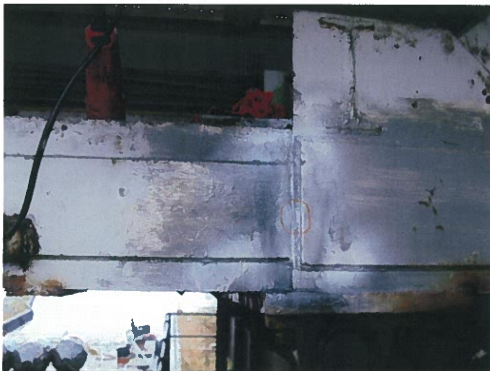
Photograph 43 – Crack in weld at welded reinforcement at panel point 5E south truss bottom chord.
