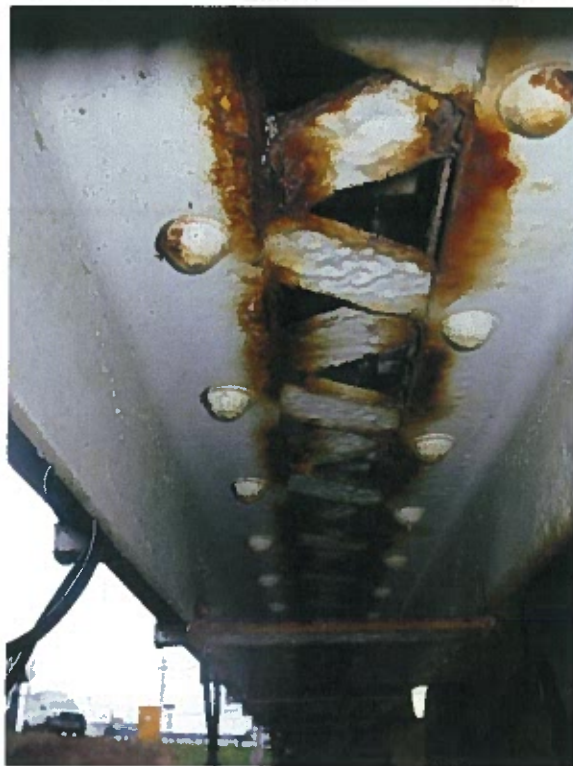
Photograph 22 – Condition of lacing bars along south truss bottom chord between panel points 3E and 5E.
