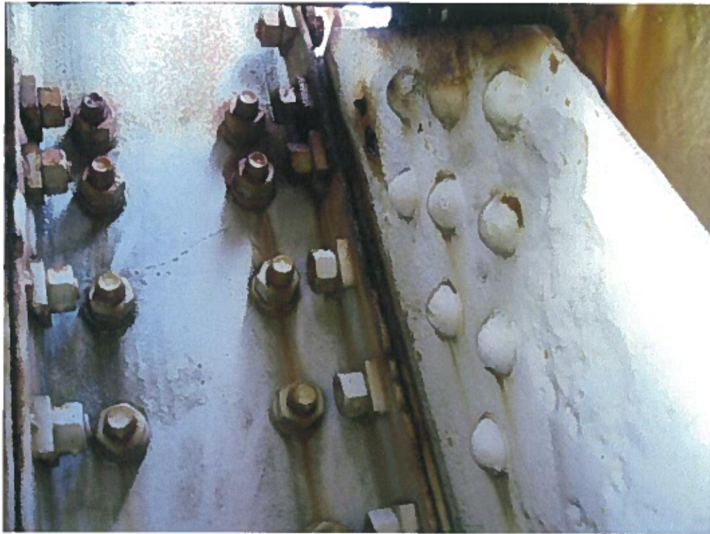
Photograph 25 – Perforation / section loss at gusset plate panel point 0 south truss bottom chord.
