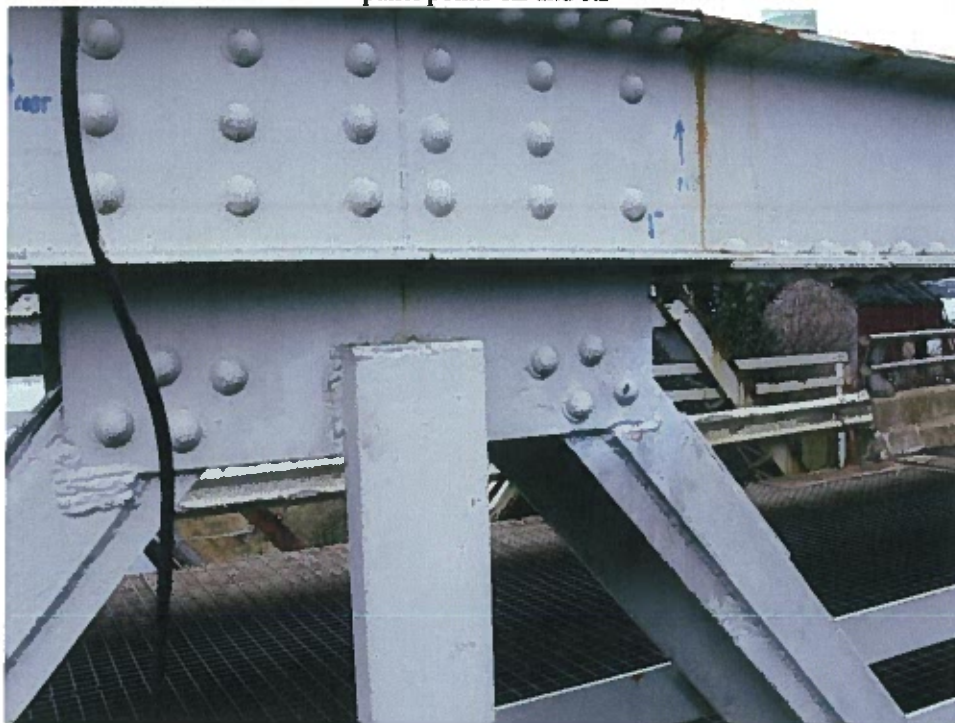
Photograph 42 – Magnetic particle testing of welded connection at the top truss diagonal member.
