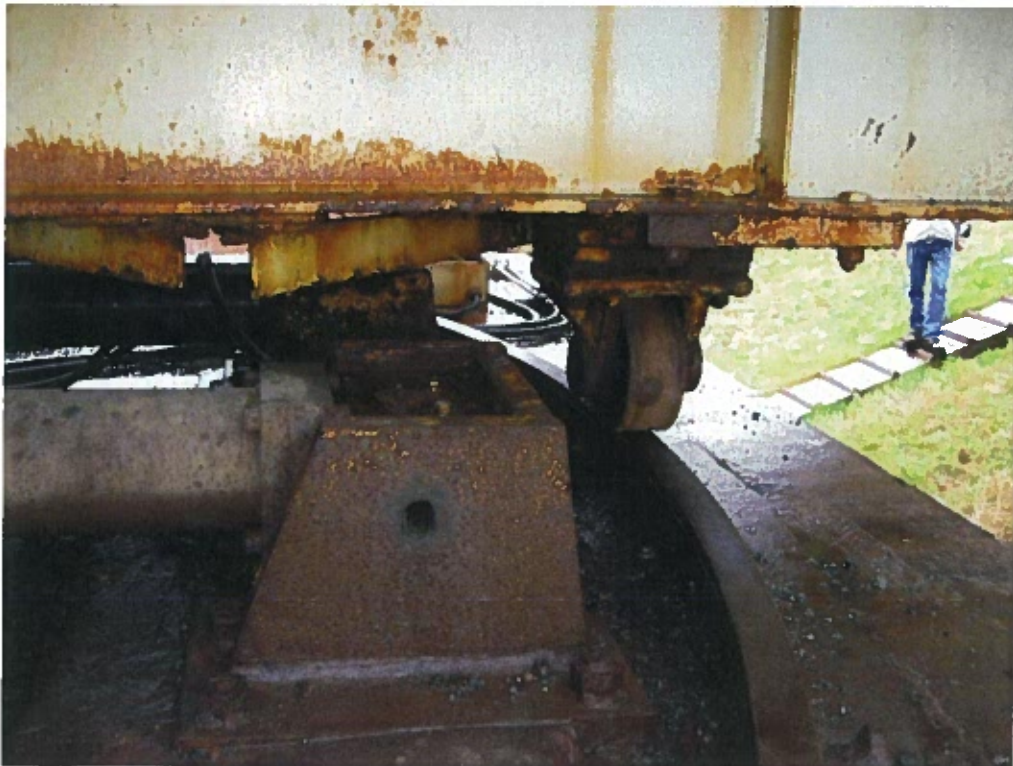
Photograph 12 – East bogey wheel, note number of shims
