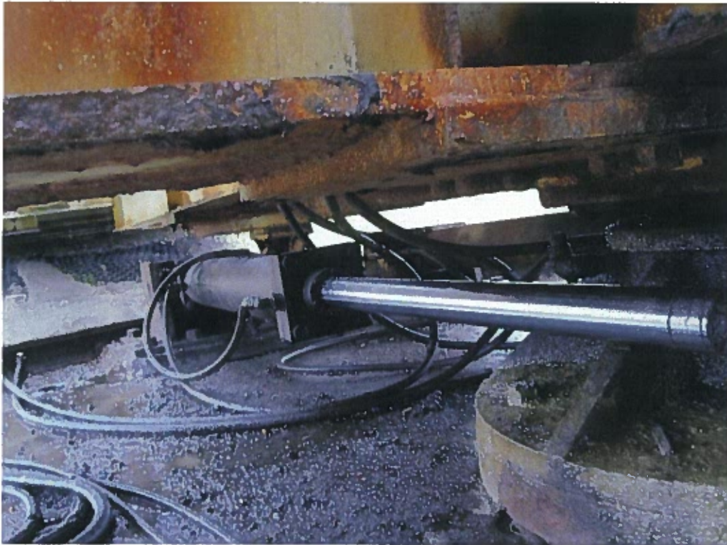
Photograph 5 – North slewing cylinder
