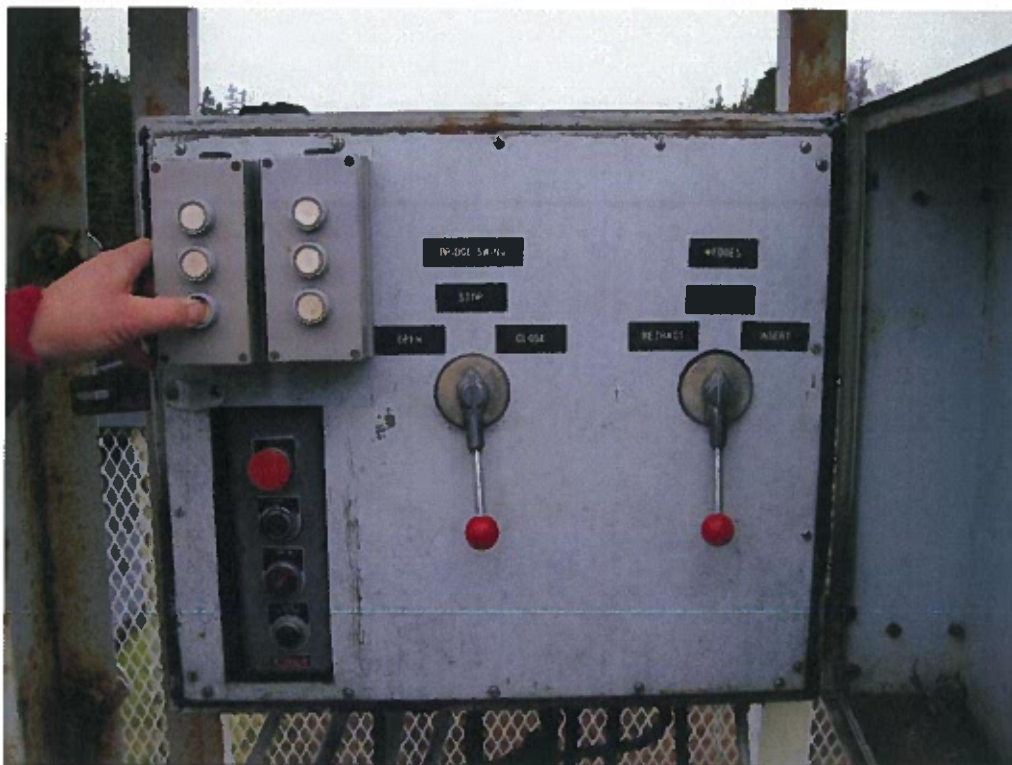
Photograph 20 – Main control panel
