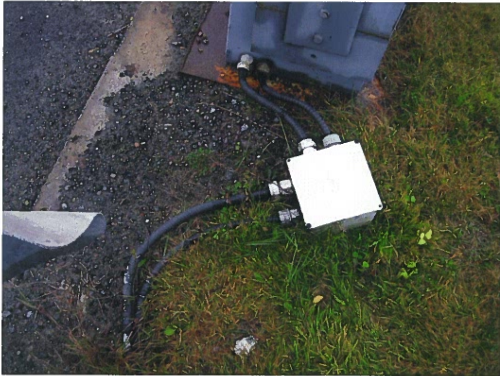
Photograph 21 – Junction box at west traffic gate
