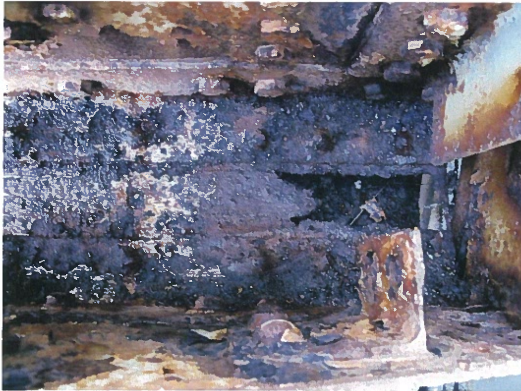
Photograph 11 – Perforation at north truss bottom chord at panel point 3W.
