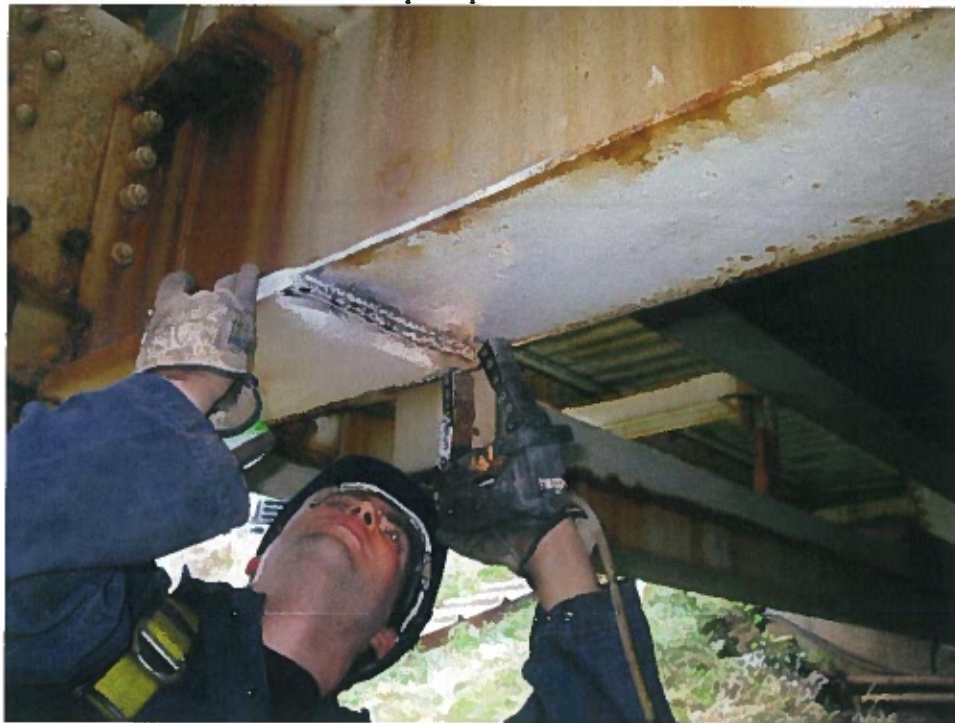
Photograph 46 – Magnetic particle testing of welded reinforcement at bottom flange of floor beam at panel point 2W
