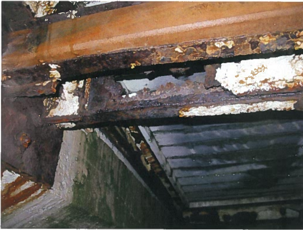
Photograph 39 – Welded reinforcement to existing transverse steel member at east app. sidewalk. Note: perforation and section loss at existing steel member
