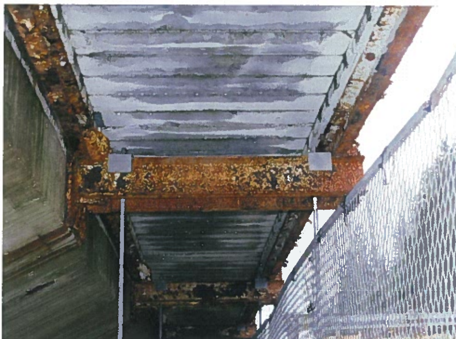
Photograph 36 – Typical condition of structural steel at sidewalk overhang at east approach.
