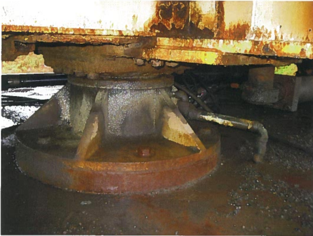
Photograph 7 – Center bearing oil drain line
