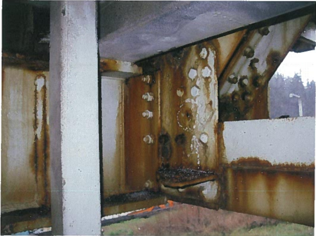
Photograph 24 – Perforation / section loss at gusset plate panel point 2W south truss bottom chord.
