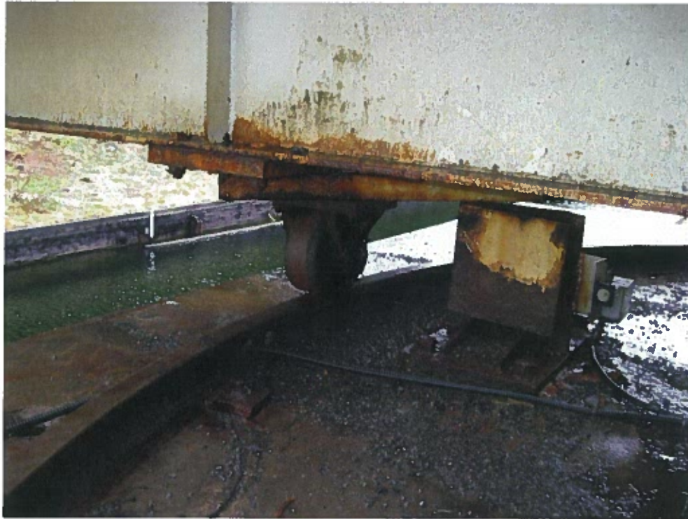
Photograph 13 – Bridge open end stop, note that rubber pad is sandwiched in between steel plates
