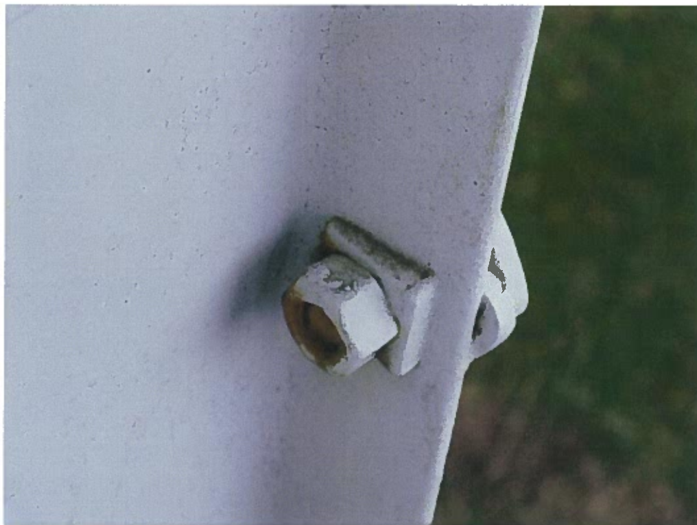
Photograph 7 – Insufficient bolt thread (typical).
