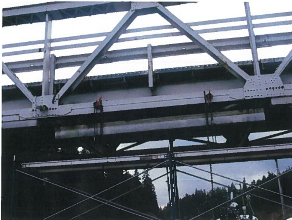
Photograph 18 – Welded reinforcement along north truss bottom chord and at panel point locations.
