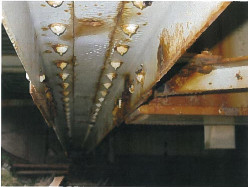
Photograph 21 – Condition of bottom chord along south truss. Note: Medium to severe corrosion.
