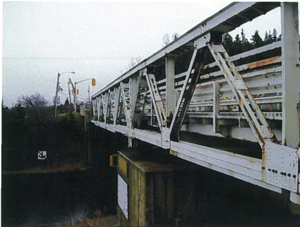
Photograph 16 – Concrete weights attached to bottom chord of north truss
