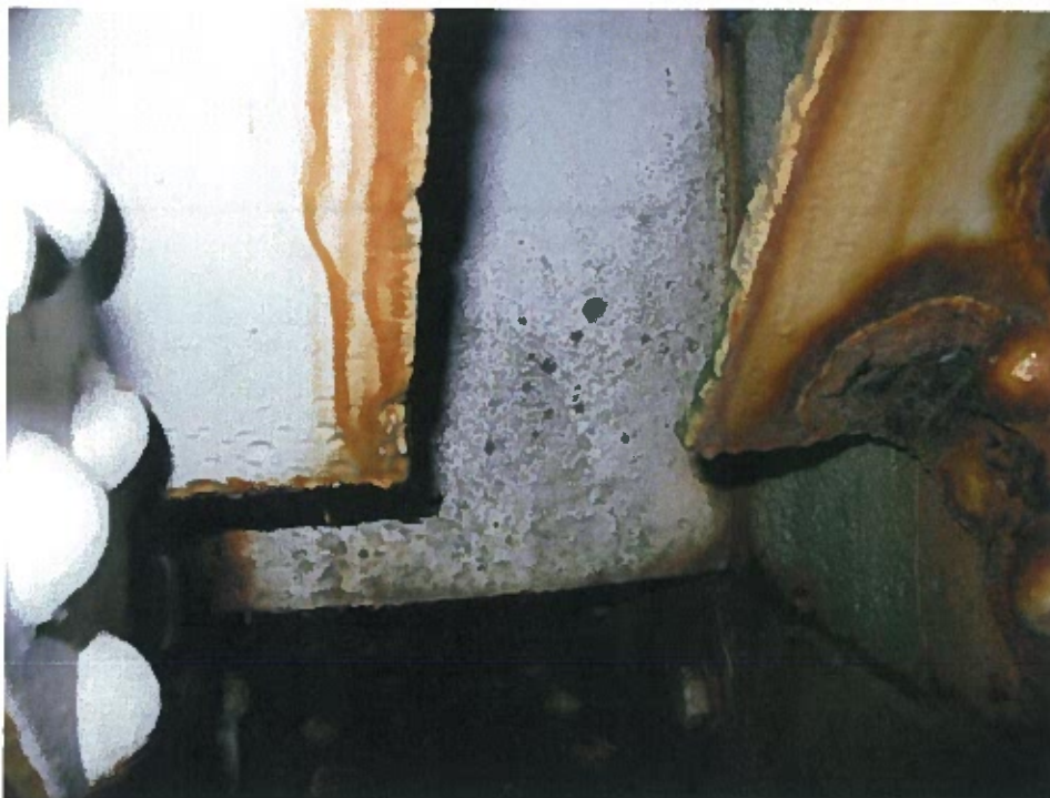
Photograph 14 – Section loss and perforation of the vertical member at panel point location along north truss bottom chord.
