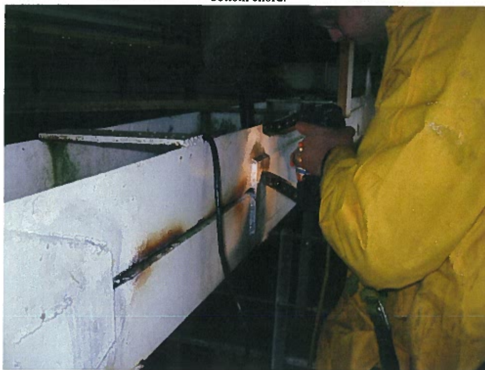
Photograph 50 – Magnetic particle testing of welded reinforcement at south truss bottom chord between panel points 4E and 5E.
