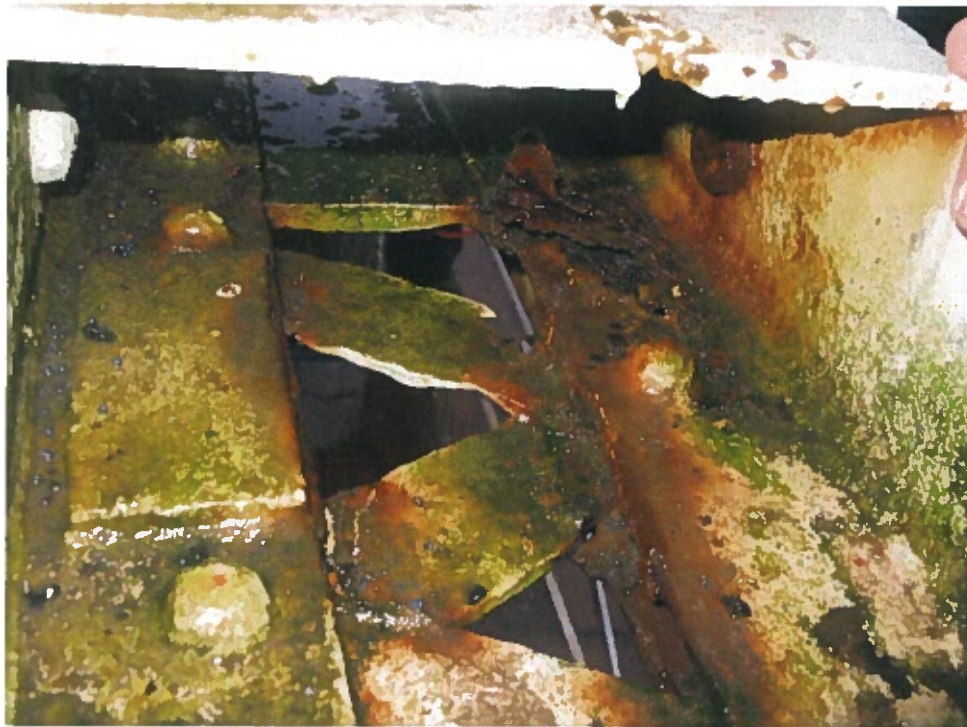
Photograph 13 – Perforation / section loss and corrosion at lacing bars at north truss bottom chord.
