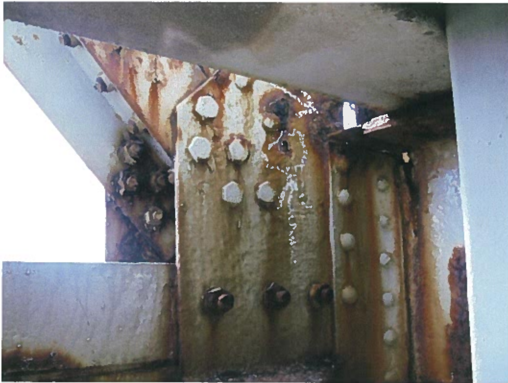
Photograph 15 – Section loss and perforation at gusset plate location at north truss panel point 2W.
