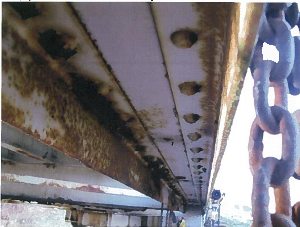
Photograph 10 - Condition of bottom chord along north truss. Note: Medium to severe corrosion.
