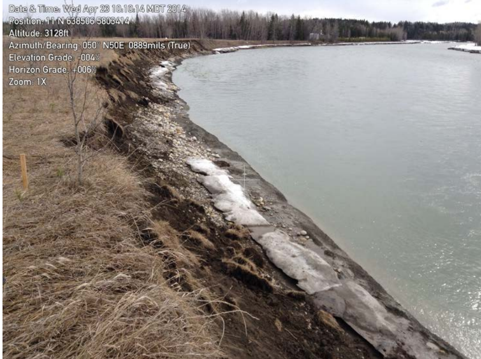
Photo 3: Downstream view of downstream extent of works location, from top of bank. This illustrates an eroding bank that is not suitable for potted plants or trees. This area should be planted with live stakes or wattles. Areas with bank nests are to be planted only with a single row of live stakes.
