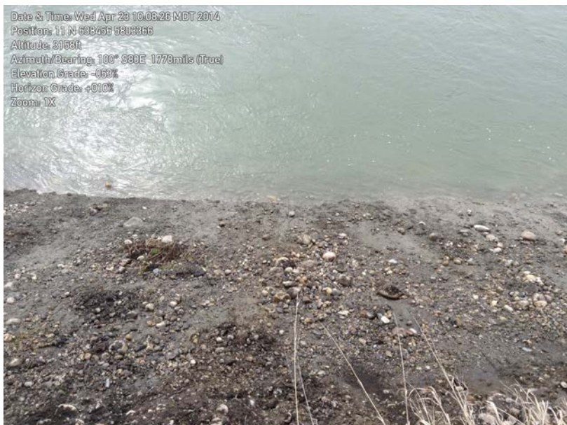
Photo 2: Clay and gravel substrate at midpoint of works. This is an example where significant groundwater outflow exists. The margin above the clay would be suitable for staking or willow wattle placement.
