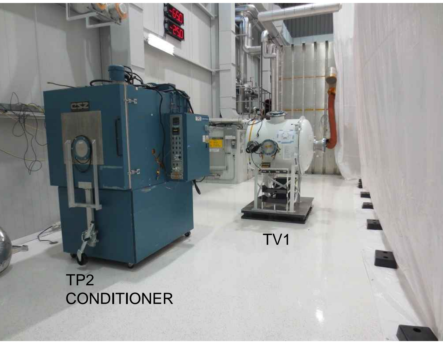
OVERALL VIEW OF TV1 & TP2 CONDITIONER UNITS IN SWING SPACE AREA (NOT POSITIONED IN PLACE) VIEW 2 A1
