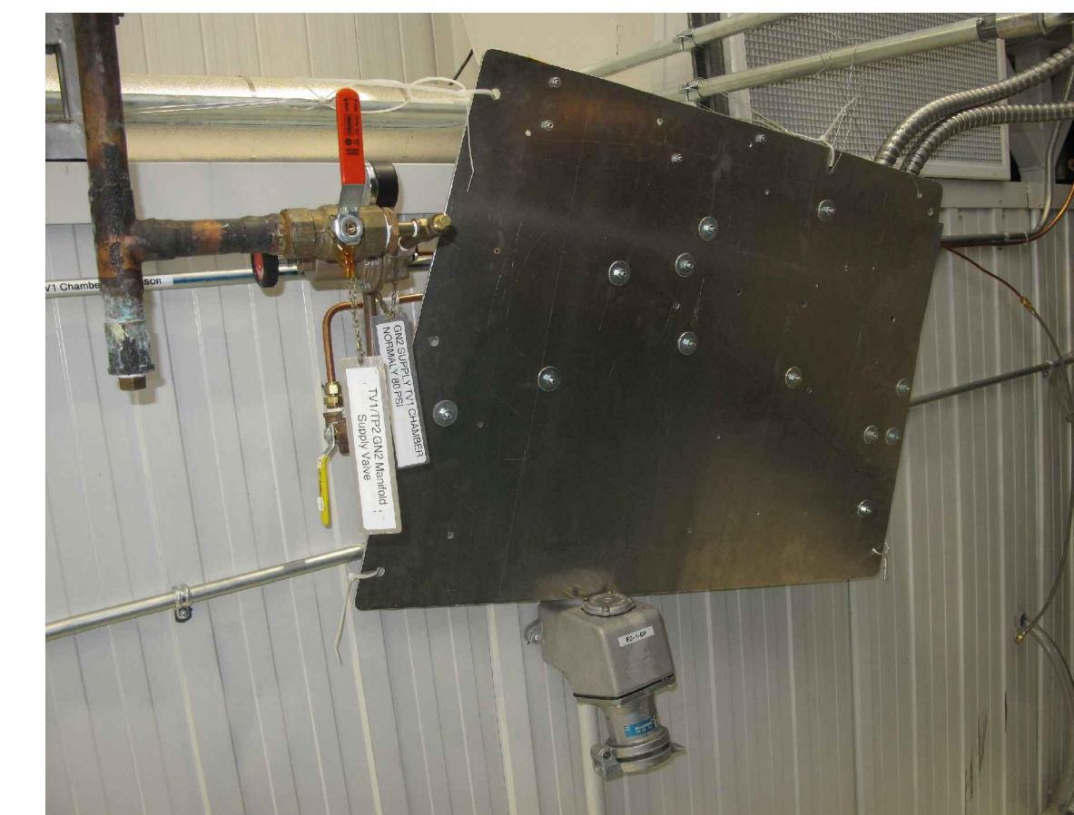
TV1 OLD ELECTRICAL PANEL
