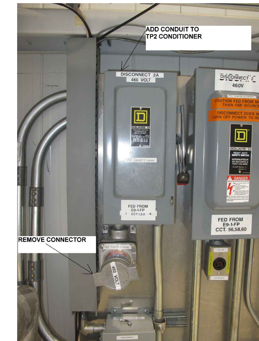
TP2 CONDITIONER DISCONNECT
