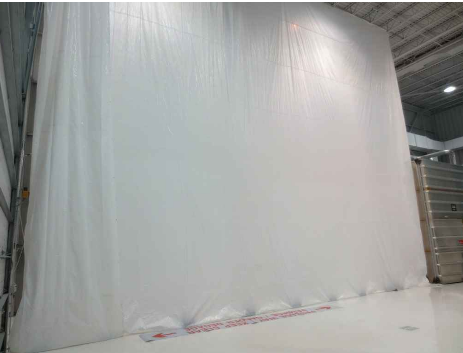
TEMPORARY TARP INSTALLED AT PROJECT AREA IN SWING SPACE, CONTRACTOR TO MODIFY & SEAL IT AS REQUIRED PRIOR TO CONSTRUCTION. VIEW 1 A1
