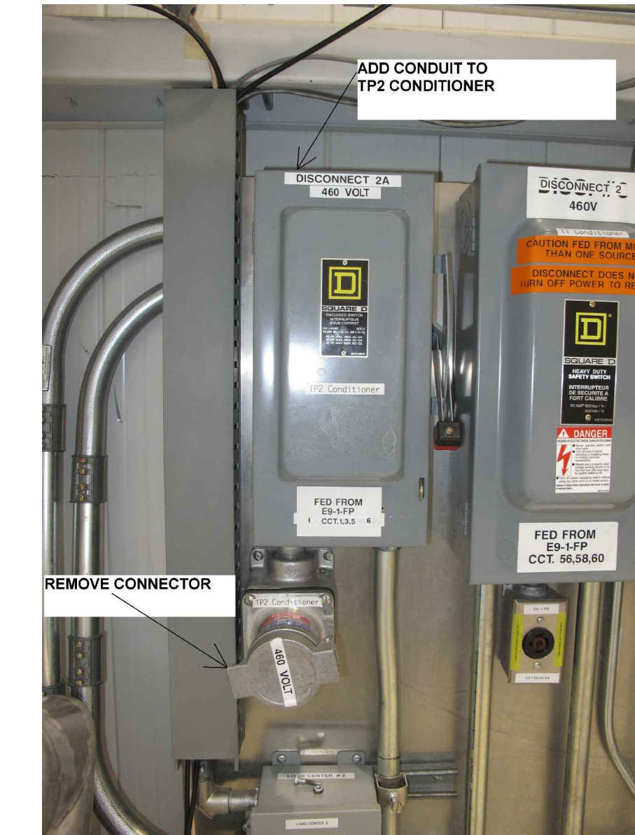
TP2 CONDITIONER DISCONNECT
