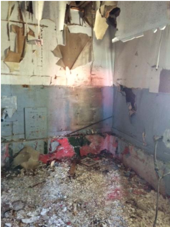
Interior of equipment building
