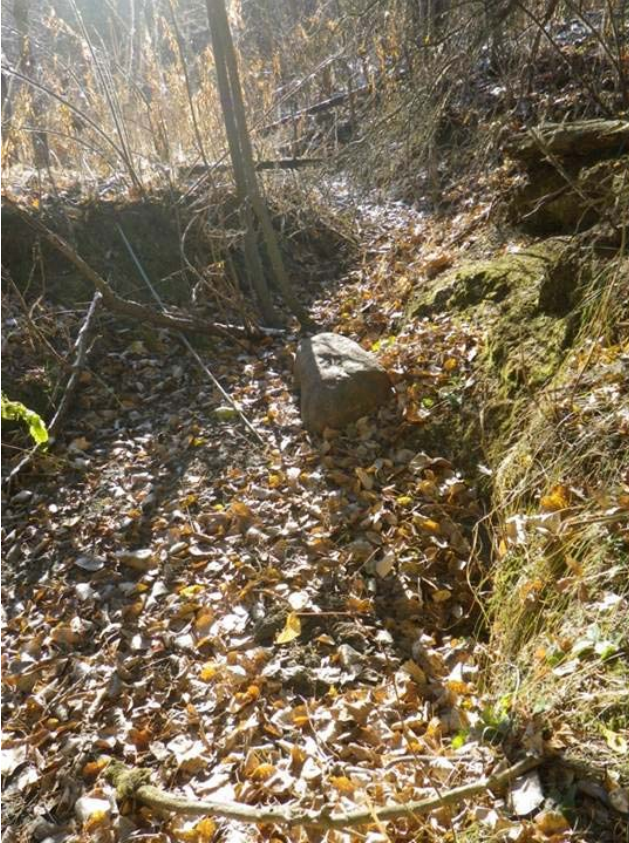
Photograph 3: Outlet pipe from Astotin Lake Recreation Area Sewage Lagoon. Photo taken facing south. Astotin Lake Recreation Area Sewage Lagoon is beyond right-hand edge of photo.
