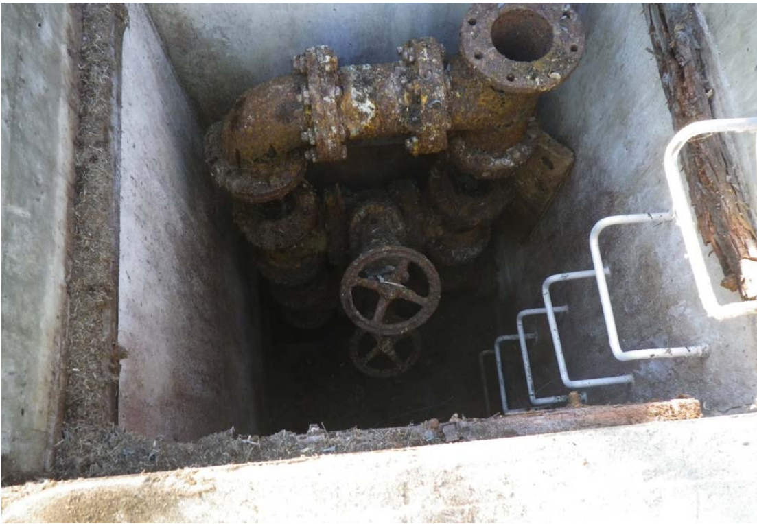
Photograph 2: Close-up of outlet structure on east side of Astotin Lake Recreation Area Sewage Lagoon.
