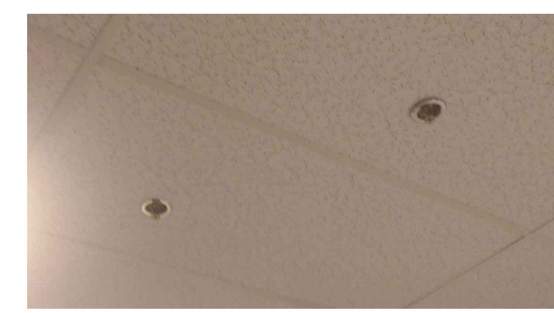
SPRINKLERS ARE LESS THAN 6 FEET APART AND DO NOT MEET NFPA 13 REQUIREMENTS.
