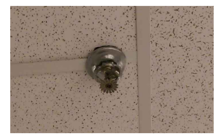
OLD STYLE SPRINKLER SHOULD BE REPLACED TO MATCH NEWER SPRINKLERS.
