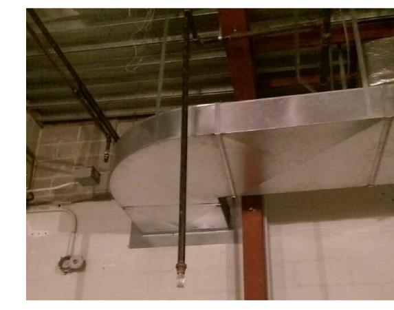
EXISTING HEAD NO LONGER REQUIRED. SHOULD BE REMOVED TO PREVENT ACCIDENTAL DISCHARGE.
