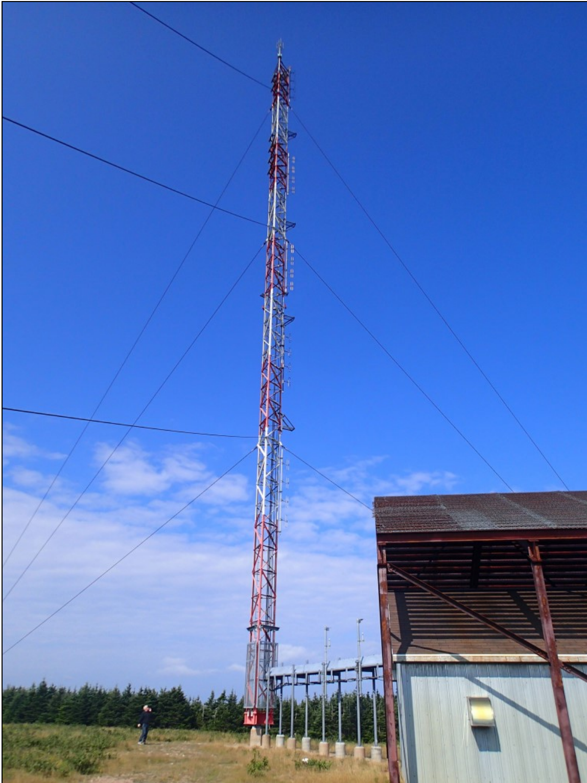
CCG VHF tower, waveguide bridge, ice shelter and equipment building.
