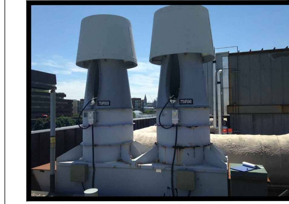
6 PICTURE - HVAC UNIT AT SUSSEX CAMPUS SCALE = N/A
