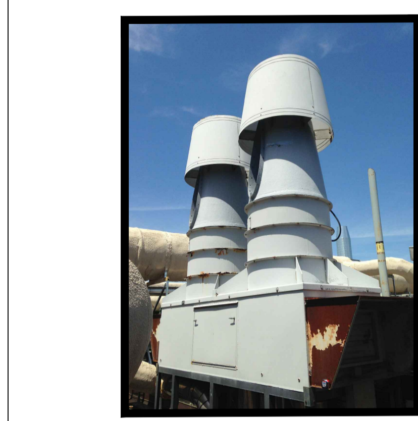
4 PICTURE - HVAC UNIT AT SUSSEX CAMPUS SCALE = N/A
