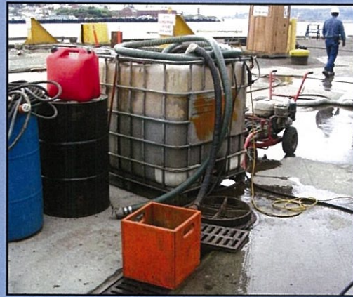
The trench drain is blocked and a sump pump is installed to collect wash water into a tote.
