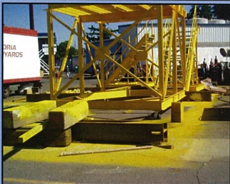
Ensure tarps are in place to prevent overspray impacting the surrounding work area.
