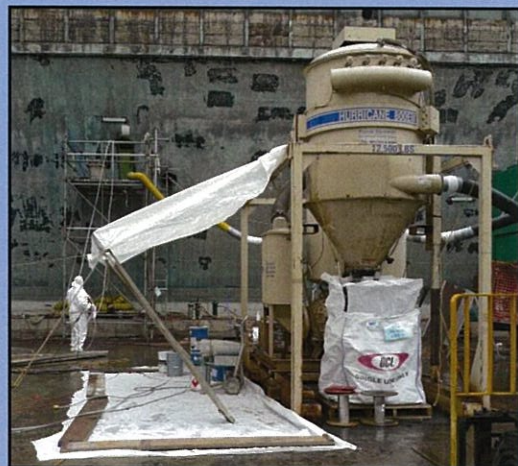
All hazardous materials must be stored in appropriate containment and away from tunnel drain system.
