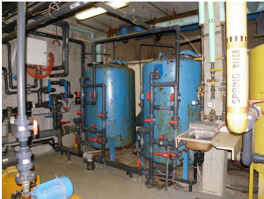
Image showing existing rapid sand filter system.
