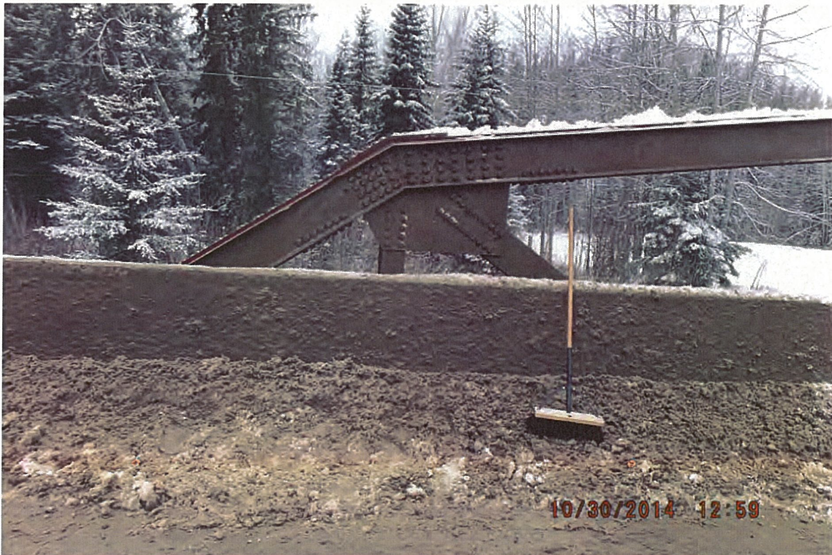
P26 - West Truss - Top Chord - Minor Collision Damage to L0-U1
