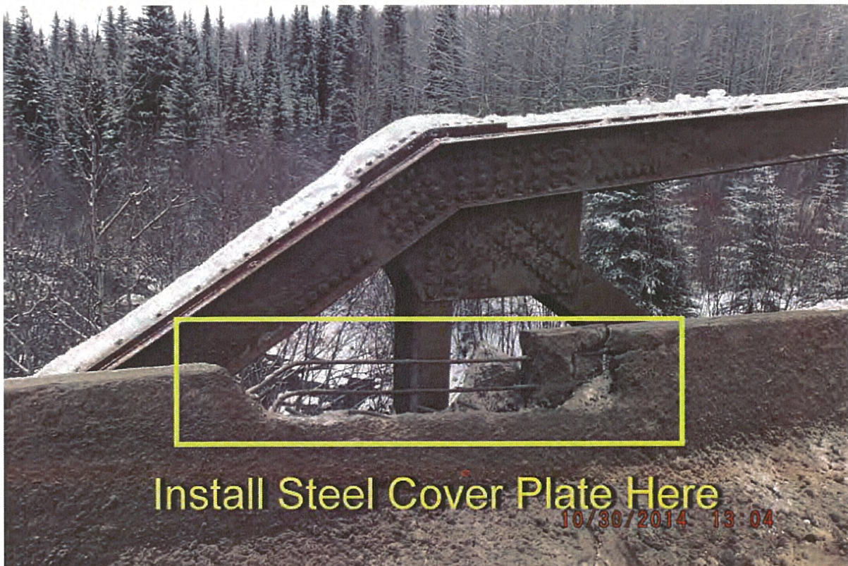
P20 - East Truss - Collision Damage to Bridge Barrier at NE Corner - No Collision Damage to Truss
