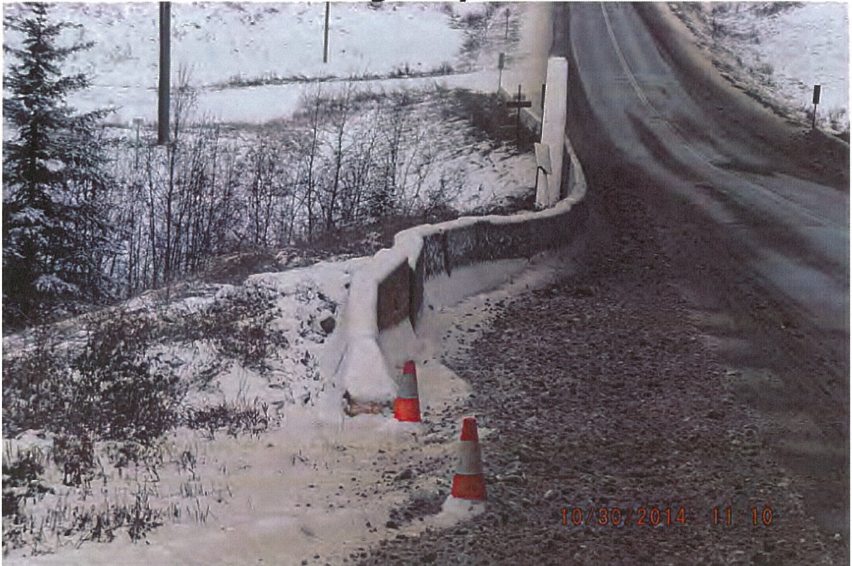
P03 - SW Approach Barrier - Shifted After Collision
