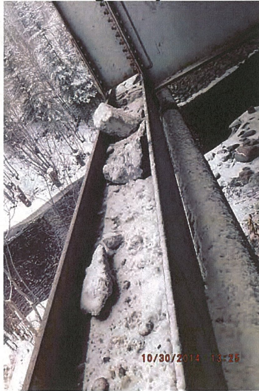
P23 - East Truss - Spalled Barrier Concrete below Spall
