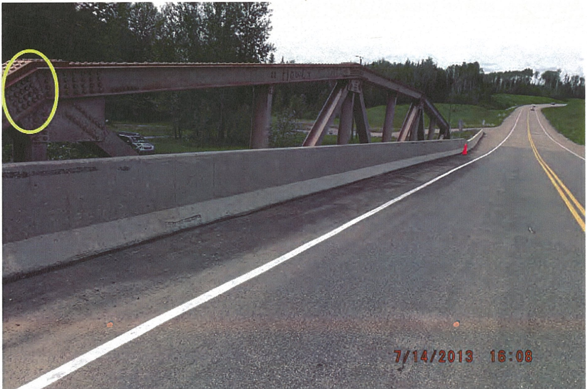
P40 - Previous July 2013 Inspection - West Truss - Looking North - Before Current Collision Damage
