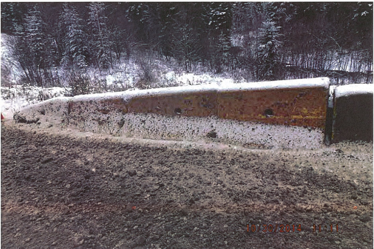
P04 - SW Approach Barrier - Broken Hook at End of Yellow Section
