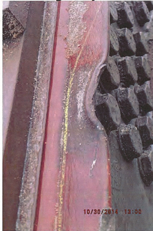
P35 - West Truss - Top Chord - Minor Collision Damage to L0-U1 - 6 Notches in Inside Channel - Notch 5 - 100 mm x 25 mm
