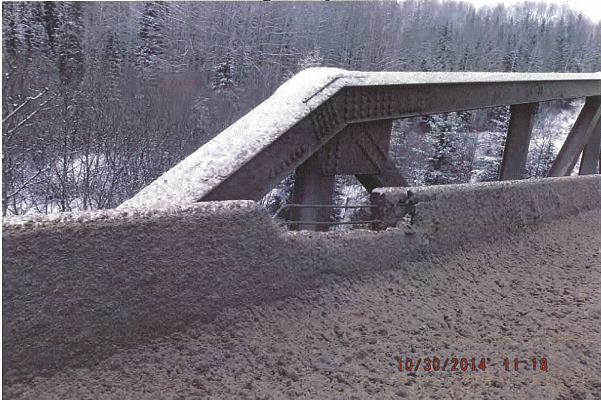
P19 - East Barriers - Collision Spall in Bridge Barrier - 2.6m x 0.35m - Exposed Rebar
