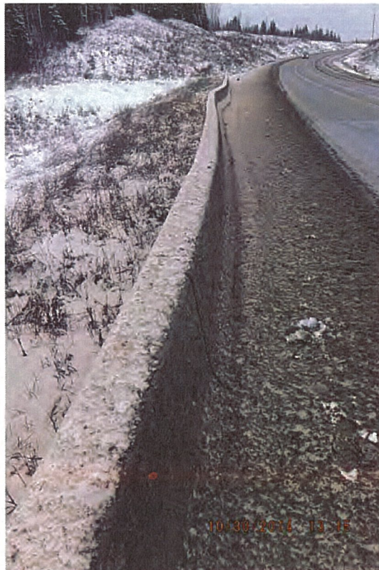
P12 - SE Approach Barrier - Kink in Barrier Alignment due to Collision
