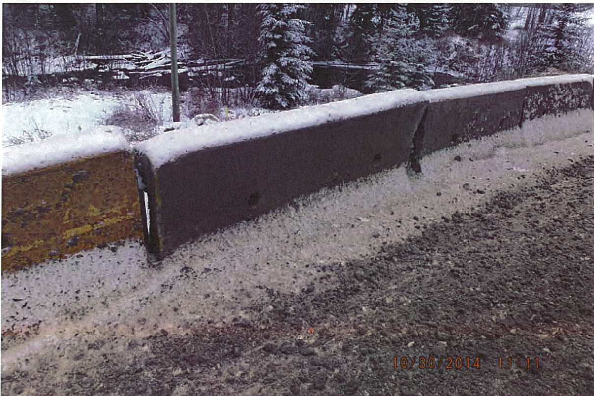
P06 - SW Approach Barriers - 2 Spalled Barrier Joints
