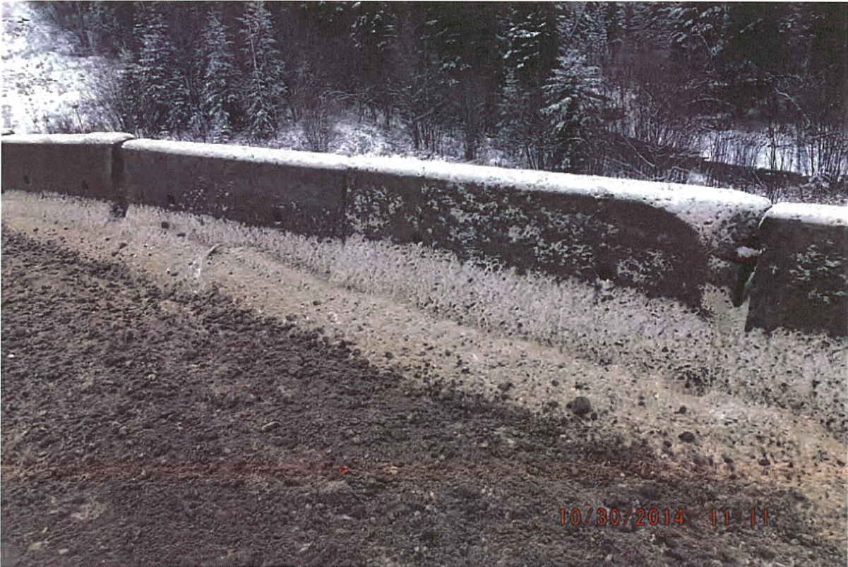
P08 - SW Approach Barriers - 2 Spalled Barrier Joints
