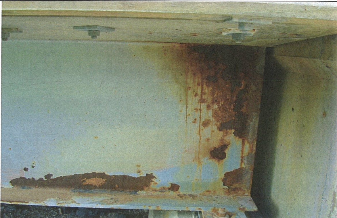
Corroded Web & Bottom Flange
