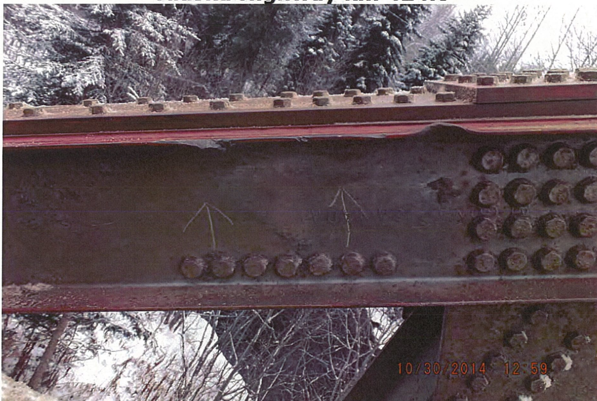
P29 - West Truss - Top Chord - Minor Collision Damage to L0-U1 - 6 Notches in Inside Channel - 5 Notches in Top Flange and 1 Notch in Bottom Flange
