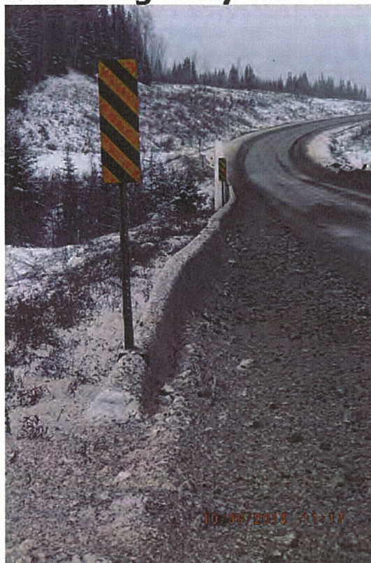
P15 - NE Approach Barrier - Slight Kink in Alignment
