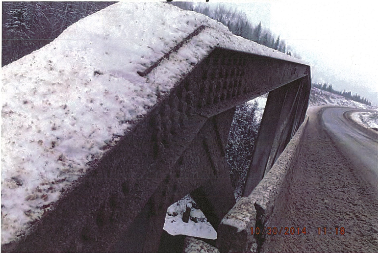
P45 - East Barrier - Top Chord - Looking South at Vertical 7 - No Impact Damage
