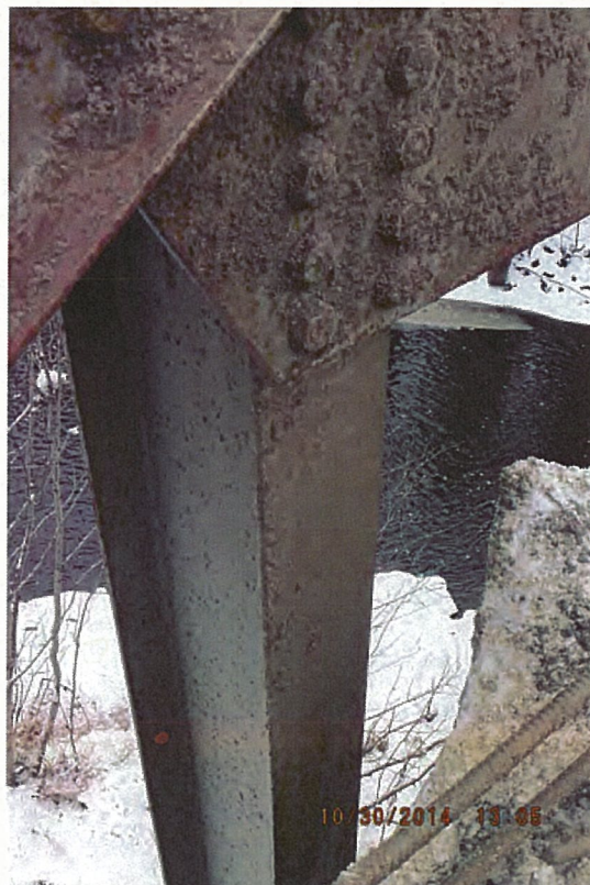
P46 - East Truss - Vertical 7 - No Collision Damage
