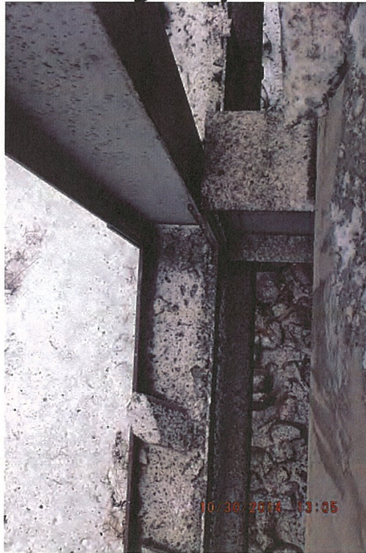
P47 - East Truss - Bottom Chord - No Collision Damage - Spalled Barrier Concrete in Bottom Chord
