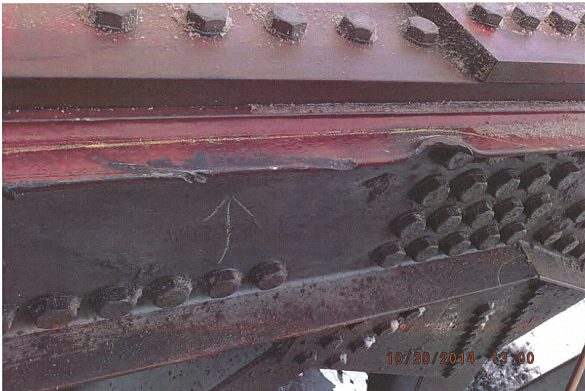
P32 - West Truss - Top Chord - Minor Collision Damage to L0-U1 - 6 Notches in Inside Channel - Notches 2, 3 and 4 - 3 mm Deep
