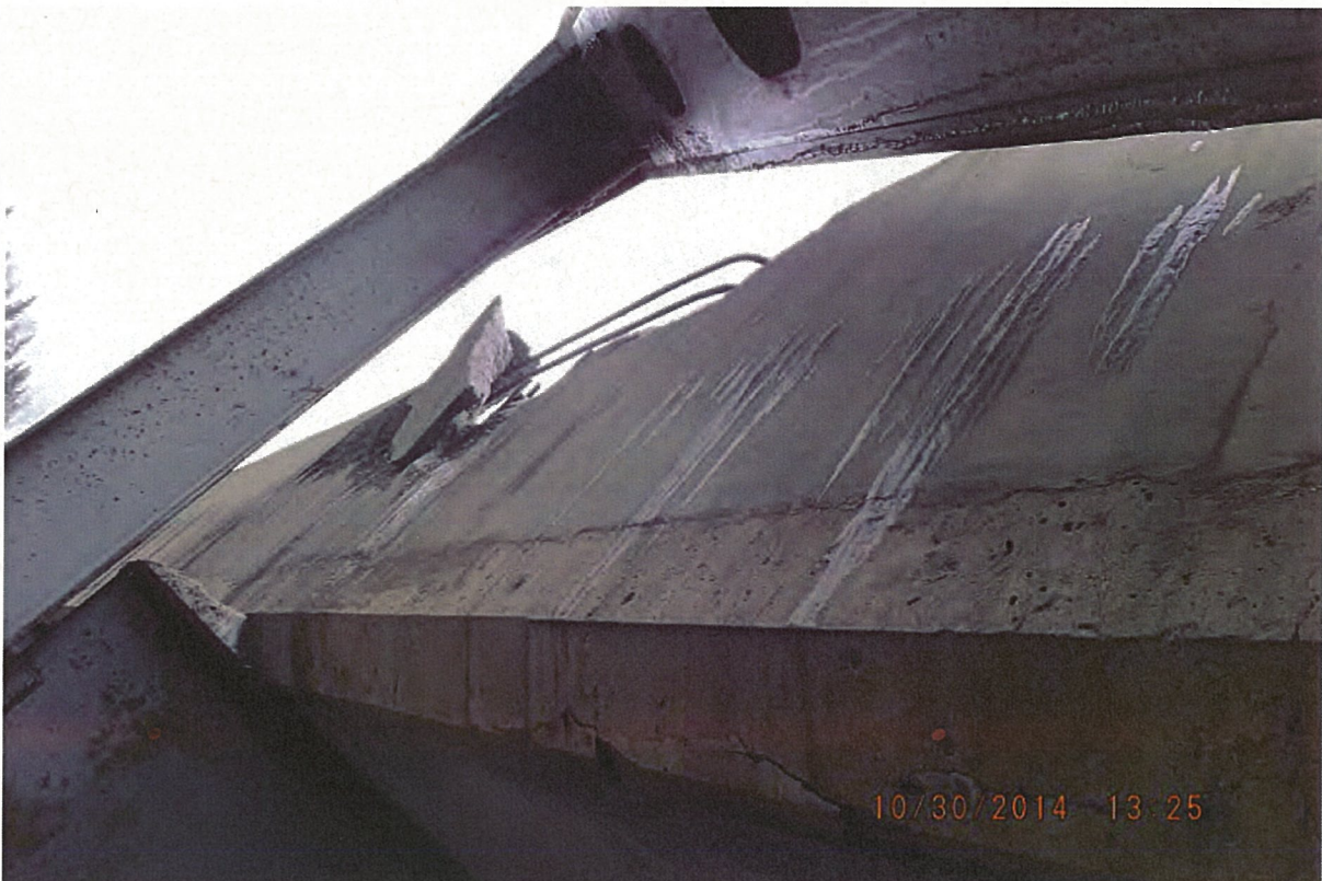
P22 - East Bridge Barrier Spall
