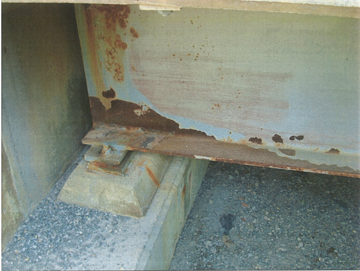
Corroded Girder & Bearing
