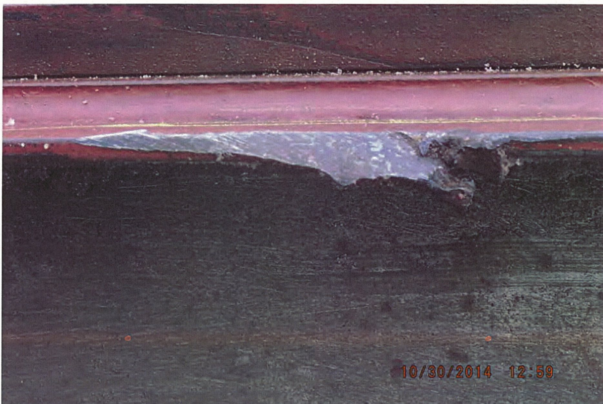
P30 - West Truss - Top Chord - Minor Collision Damage to L0-U1 - 6 Notches in Inside Channel - Notch 1 -110 mm x 12 mm Tear
