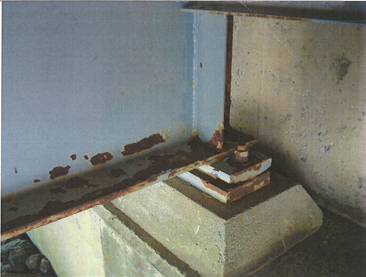
Corroded Girder & Bearing
