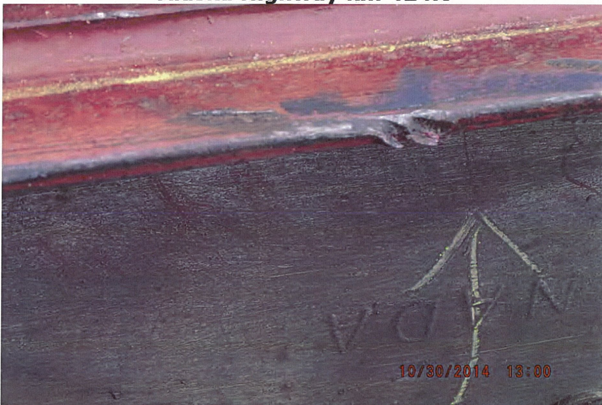
P33 - West Truss - Top Chord - Minor Collision Damage to L0-U1 - 6 Notches in Inside Channel - Notches 2, 3 and 4 - 3 mm Deep
