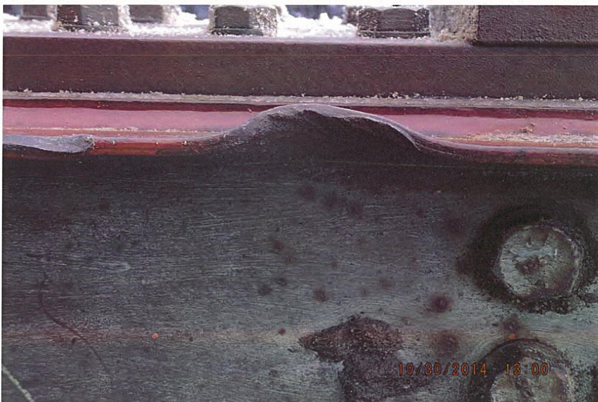
P34 - West Truss - Top Chord - Minor Collision Damage to L0-U1 - 6 Notches in Inside Channel - Notch 5 - 100 mm x 25 mm
