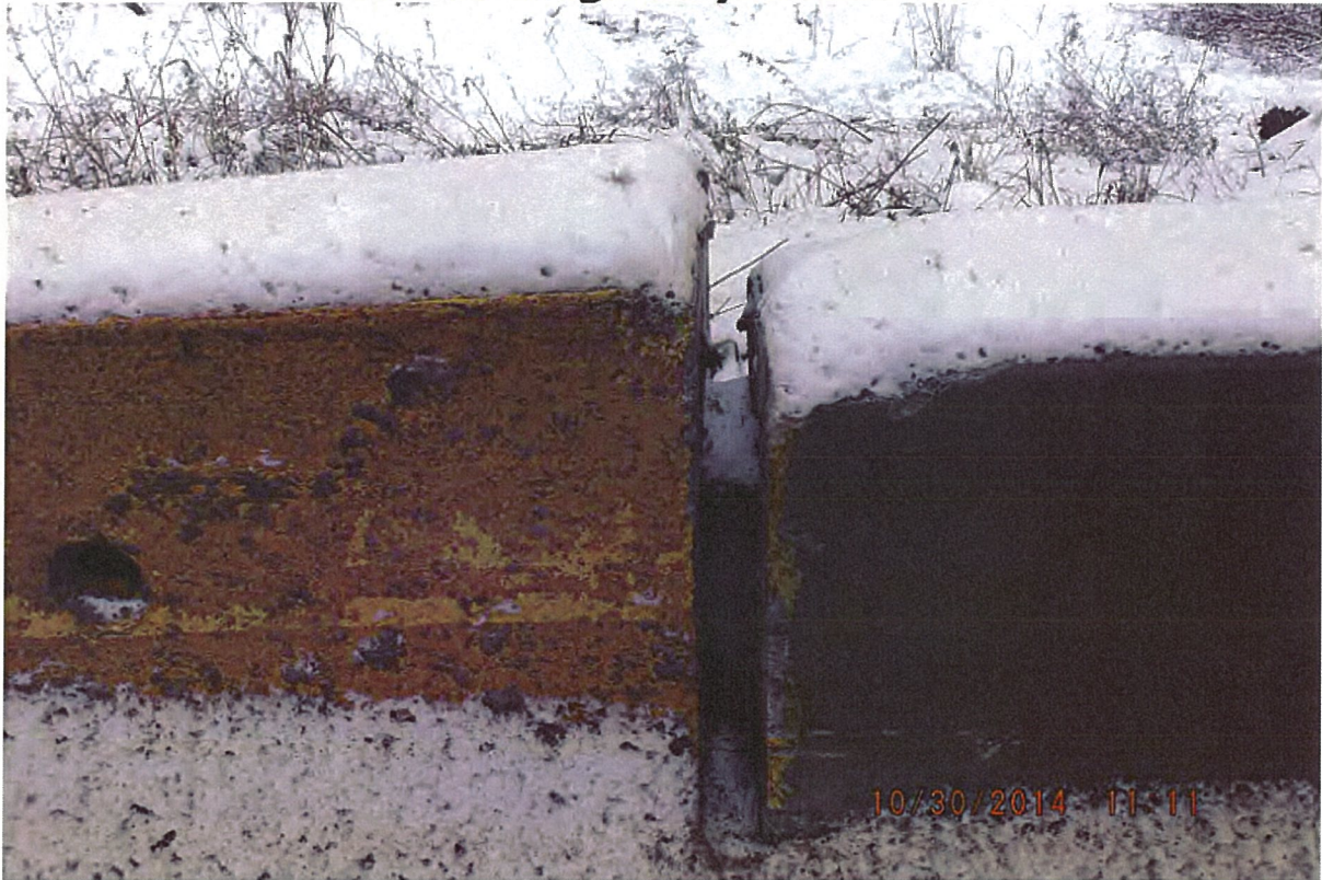
P05 - SW Approach Barrier - Broken Hook at End of Yellow Section
