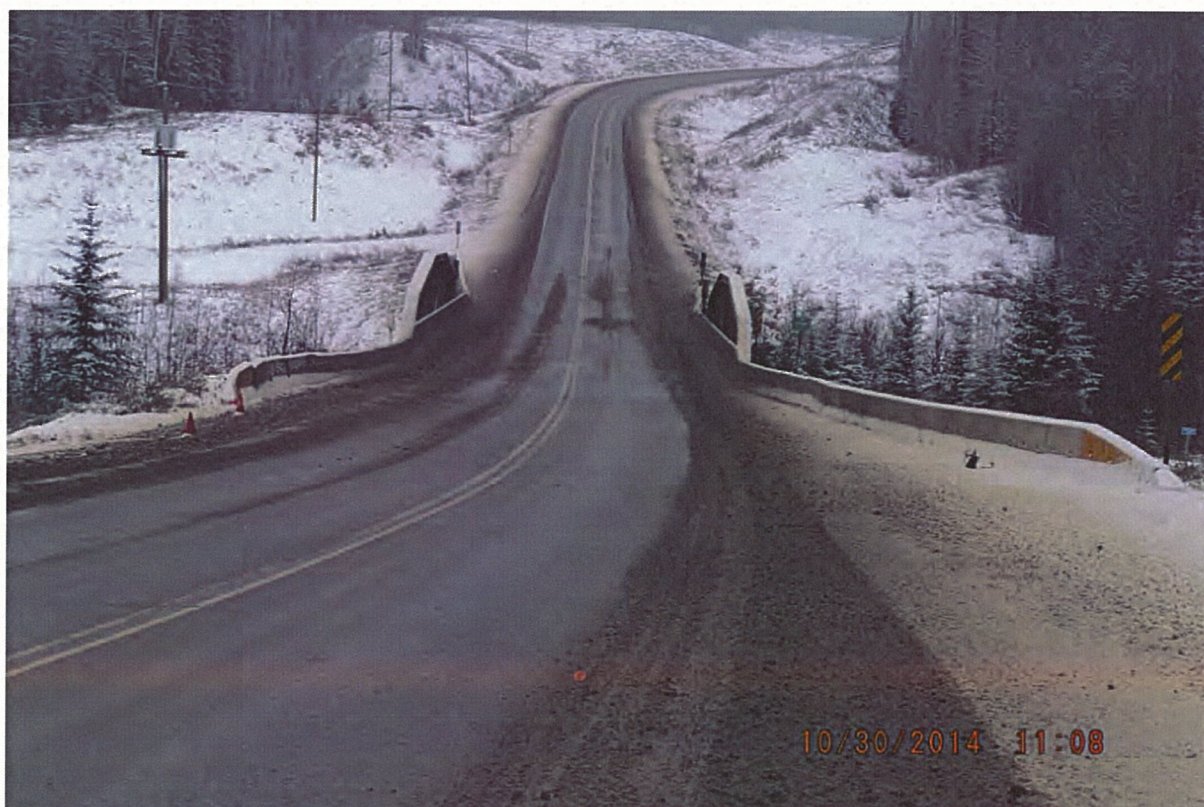
P02 - South Approach - Looking North - Both Approach Barriers Shifted after Collision
