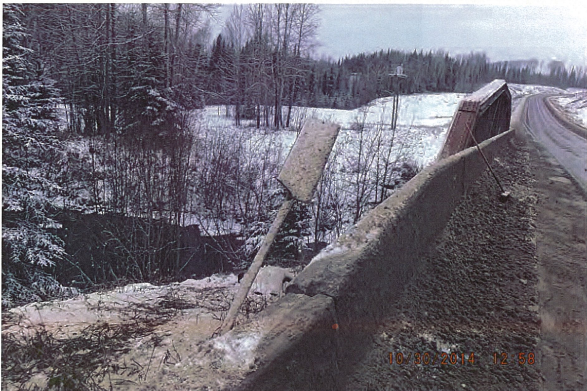
P10 - SW Delineator Sign Pushed Over
