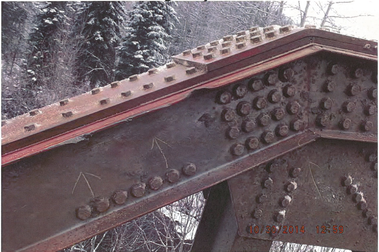
P27 - West Truss - Top Chord - Minor Collision Damage to L0-U1 - 6 Notches in Inside Channel - 5 Notches in Top Flange and 1 Notch in Bottom Flange
