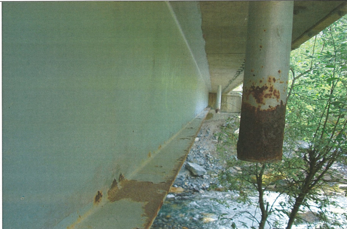
Corroded Bottom Flange & Drain Pipe
