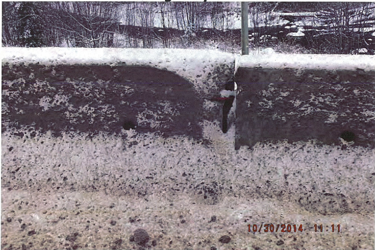
P09 - SW Approach Barriers - 2 Spalled Barrier Joints
