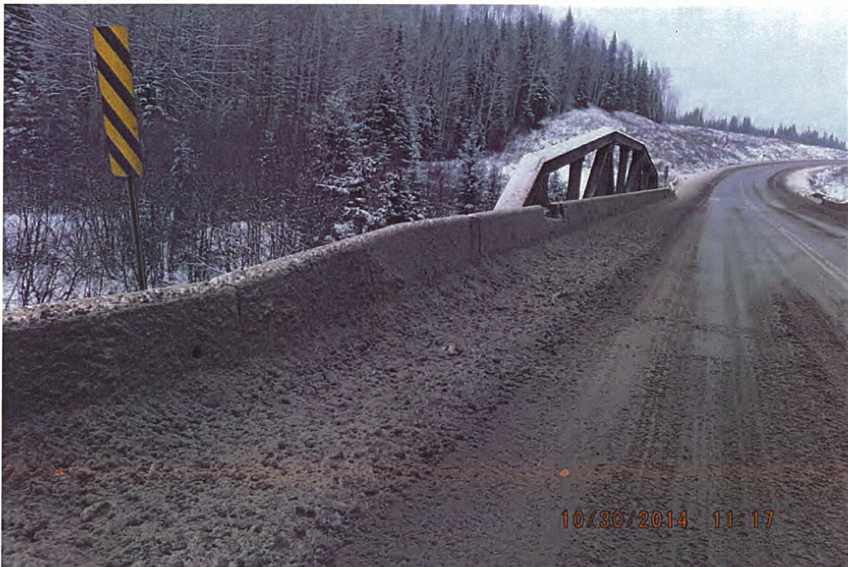
P18 - East Barriers - Collision Spall in Bridge Barrier
