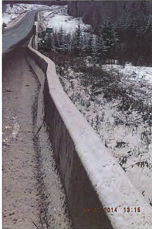
P11 - SE Approach Barrier - Kink in Barrier Alignment due to Collision
