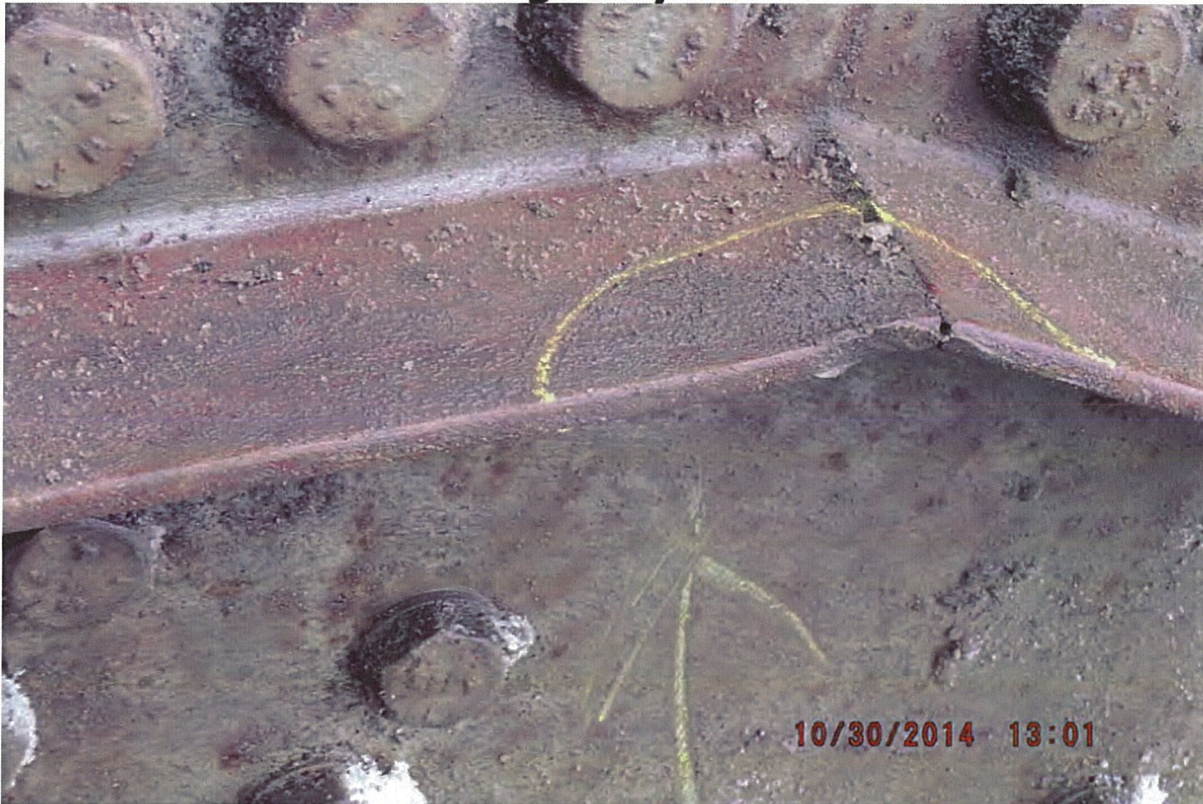
P37 - West Truss - Top Chord - Minor Collision Damage to L0-U1 - 6 Notches in Inside Channel - Notch 6 - 30 mm x 3 mm Deep
