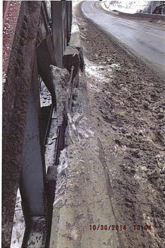
P21 - East Truss - Collision Damage to Bridge Barrier at NE Corner - No Collision Damage to Truss
