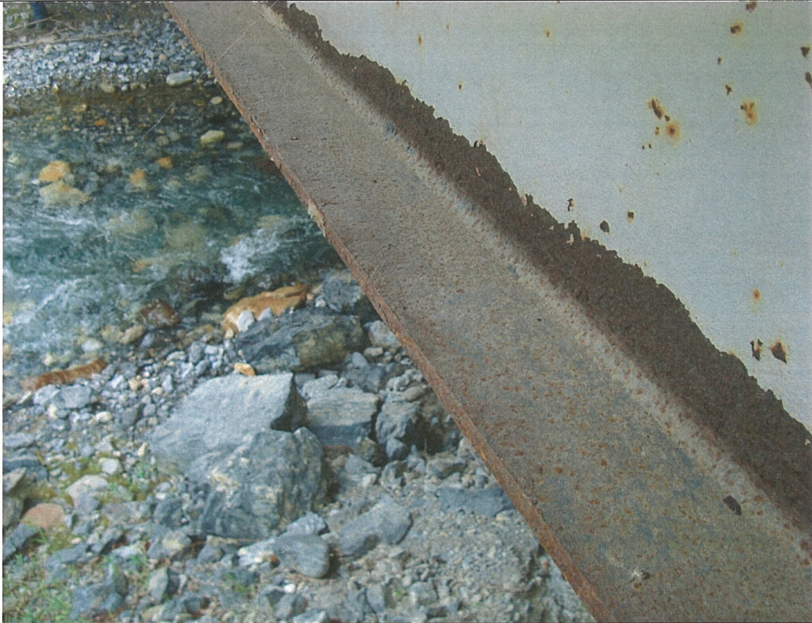
Corroded Bottom Flange
