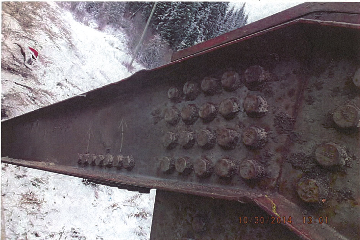
P38 - West Truss - Top Chord - Minor Collision Damage to L0-U1 - 6 Notches in Inside Channel
