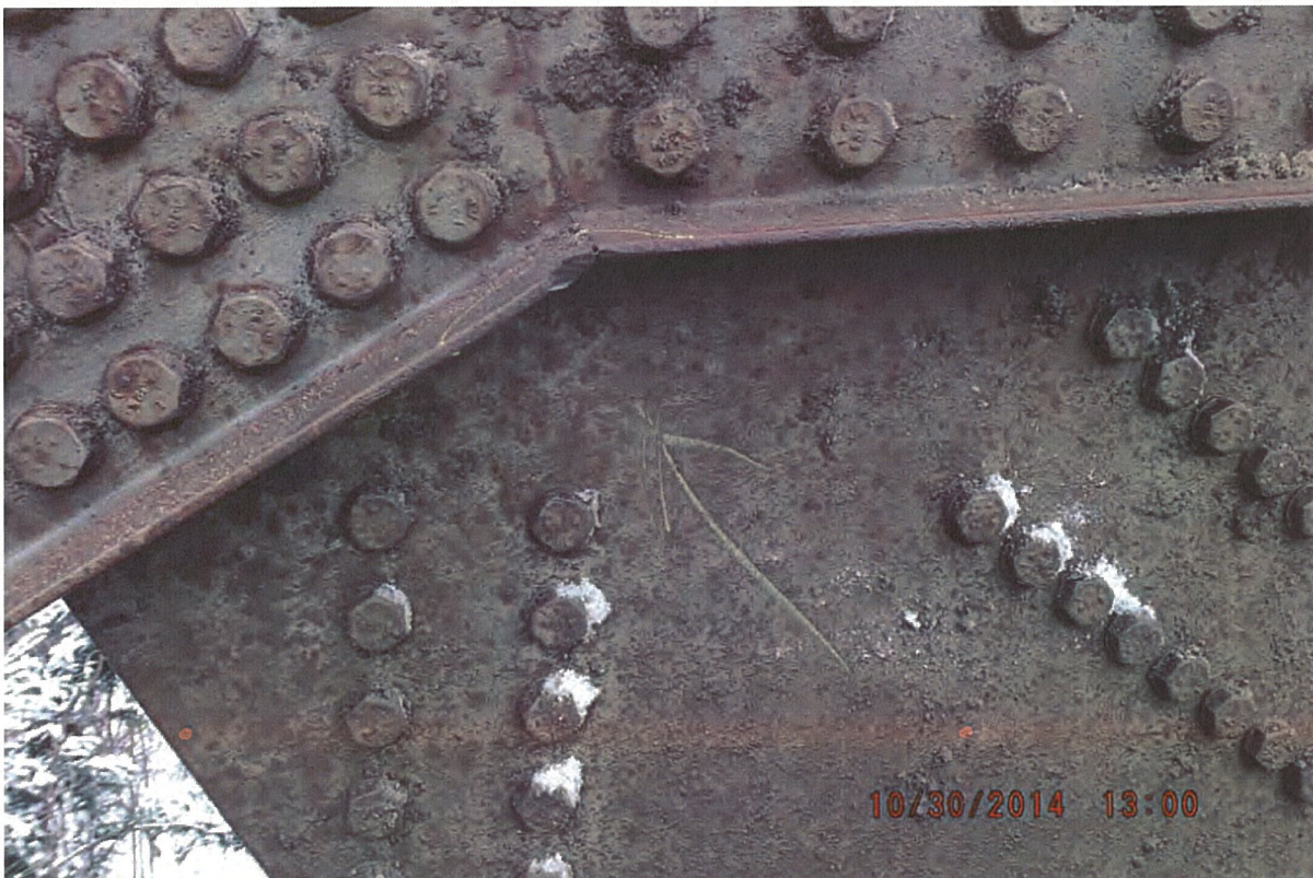
P36 - West Truss - Top Chord - Minor Collision Damage to L0-U1 - 6 Notches in Inside Channel - Notch 6 - 30 mm x 3 mm Deep
