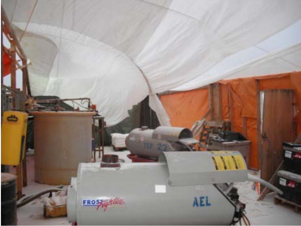
Figure 11: Plant Winterizing Phase – Frost Fighter
