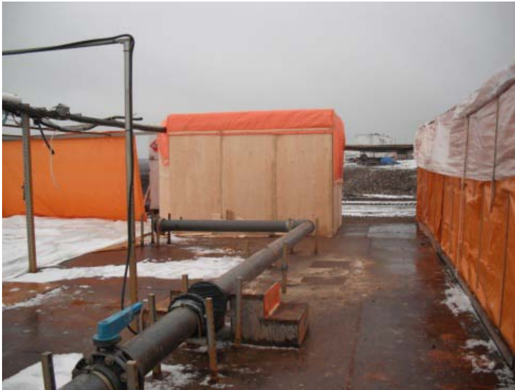
Figure 24: Electrical Control Panel Plywood Enclosure (Platform)
