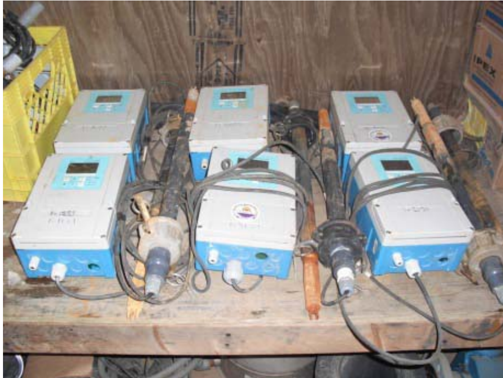
Figure 21: Transmitter and pH Sensor Storage (Storage Room)
