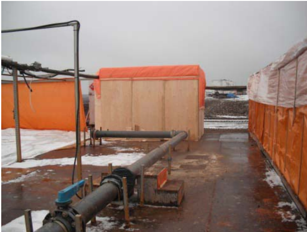
Figure 24: Electrical Control Panel Plywood Enclosure (Platform)
