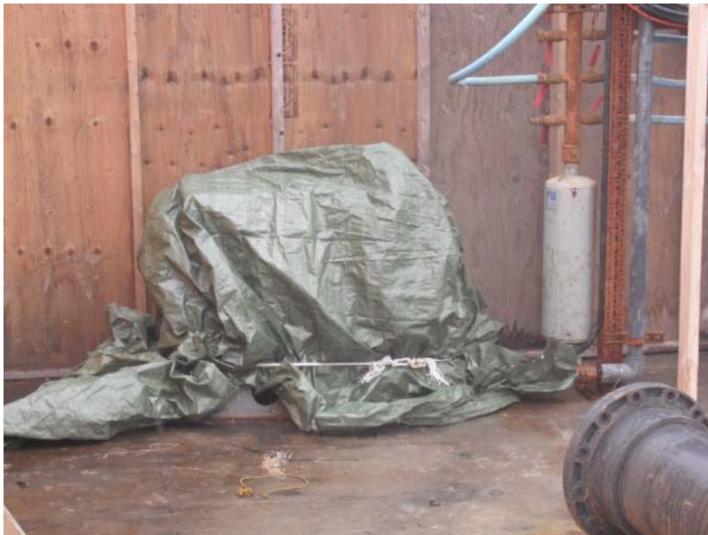
Figure 18: Chemical Makeup Blower Storage (Platform)
