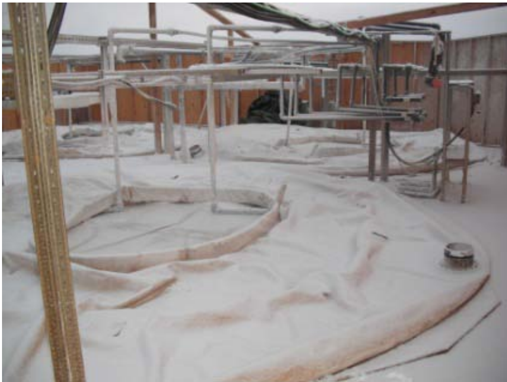
Figure 16: Lime Onion Tank Storage (Platform)
