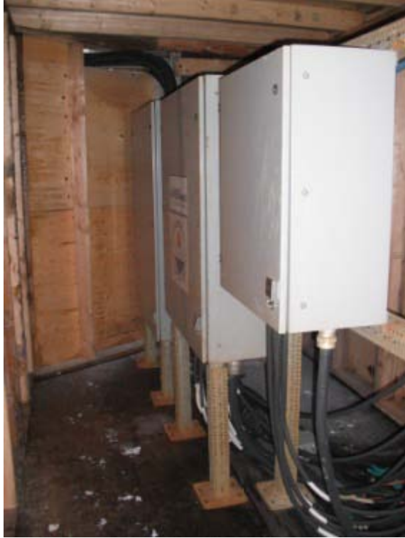
Figure 23: Electrical Control Panel Storage (Platform)
