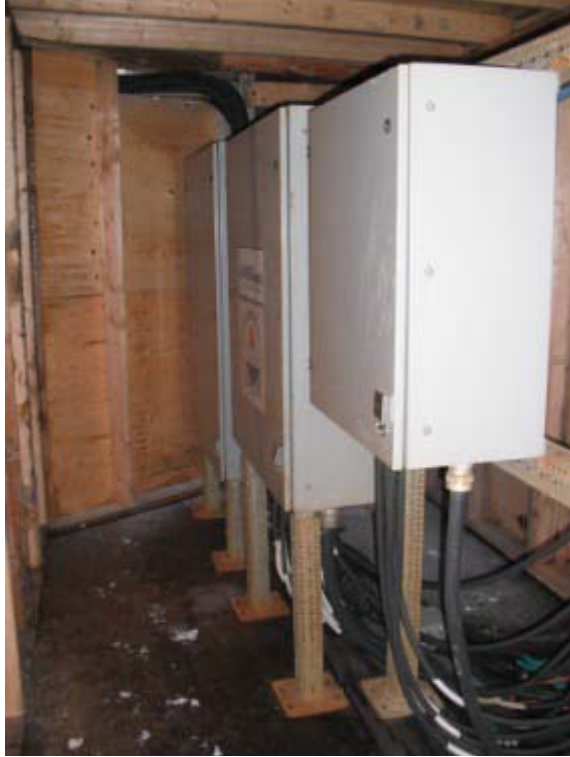
Figure 23: Electrical Control Panel Storage (Platform)
