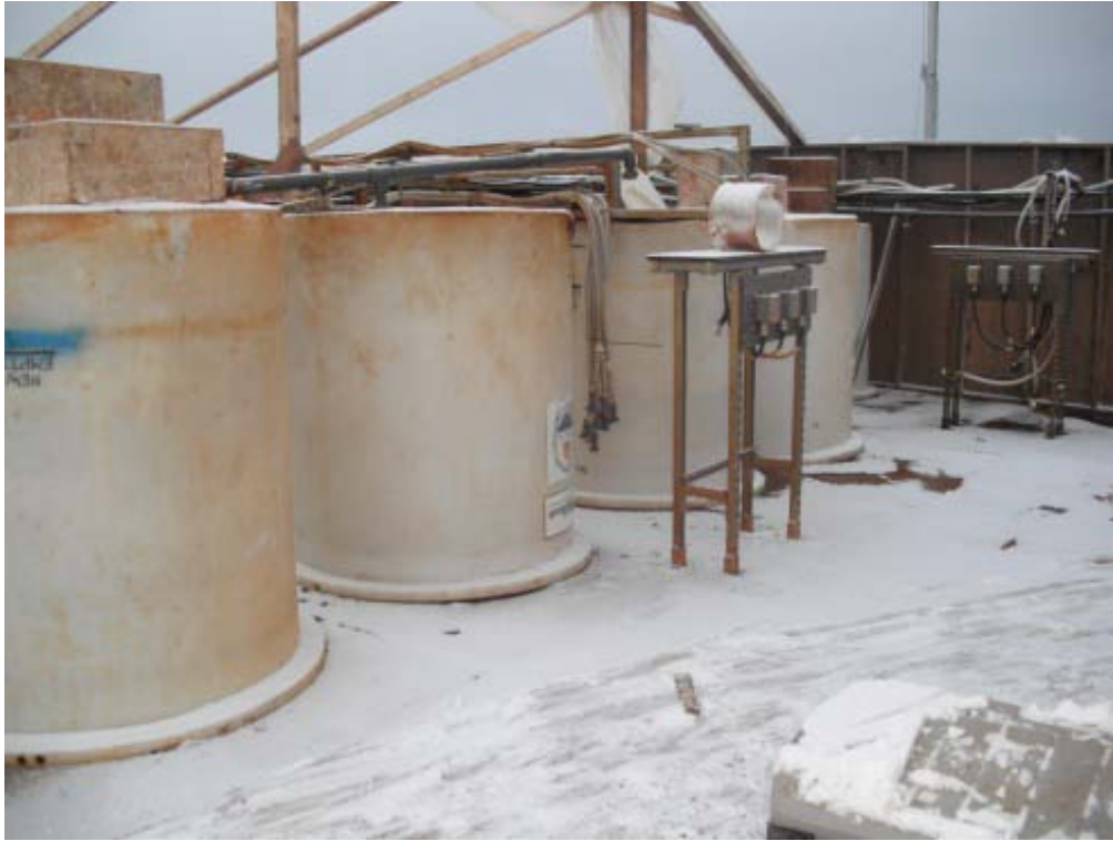
Figure 17: Polymer and Sodium Metabisulfite Tank Storage (Platform)
