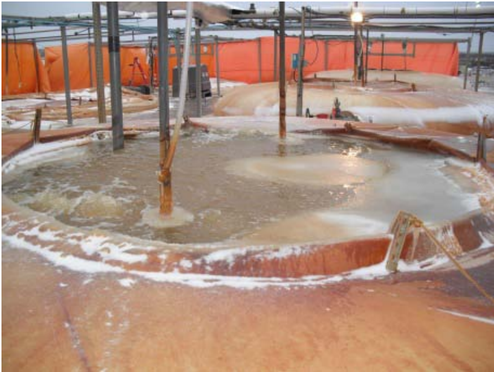
Figure 12: Plant Winterizing Phase – Tanks Freezing
