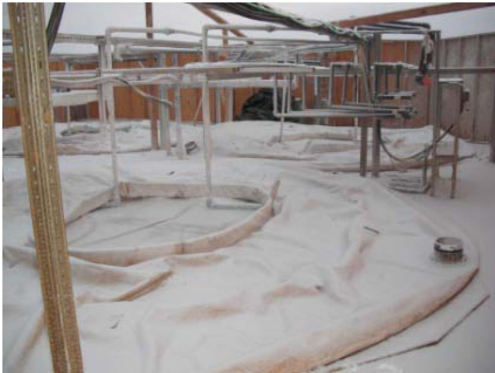
Figure 16: Lime Onion Tank Storage (Platform)
