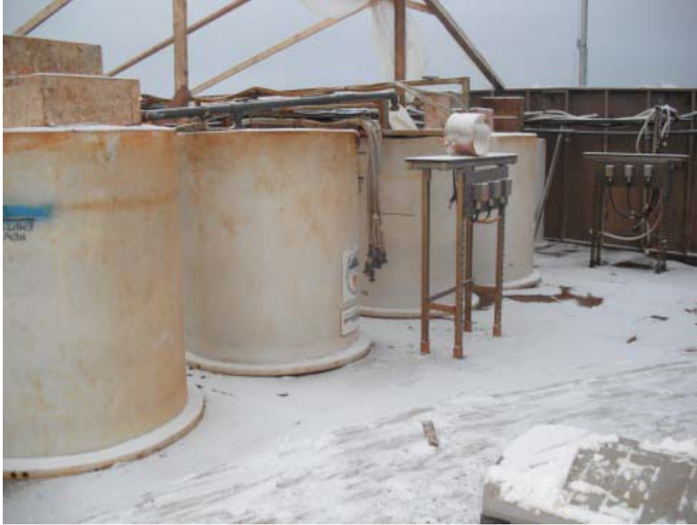
Figure 17: Polymer and Sodium Metabisulfite Tank Storage (Platform)
