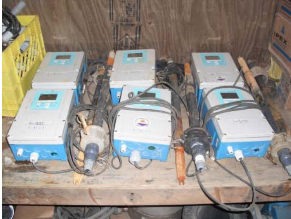
Figure 21: Transmitter and pH Sensor Storage (Storage Room)
