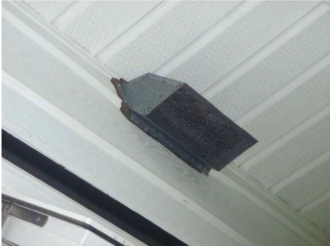
Customs Office - 11 - Asbestos-containing grey putty (A6) surrounding exterior vent on north side of building.
