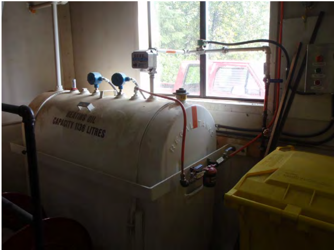
Secondary Examination Shelter - 7 - Heating oil tank in northeast corner of building.
