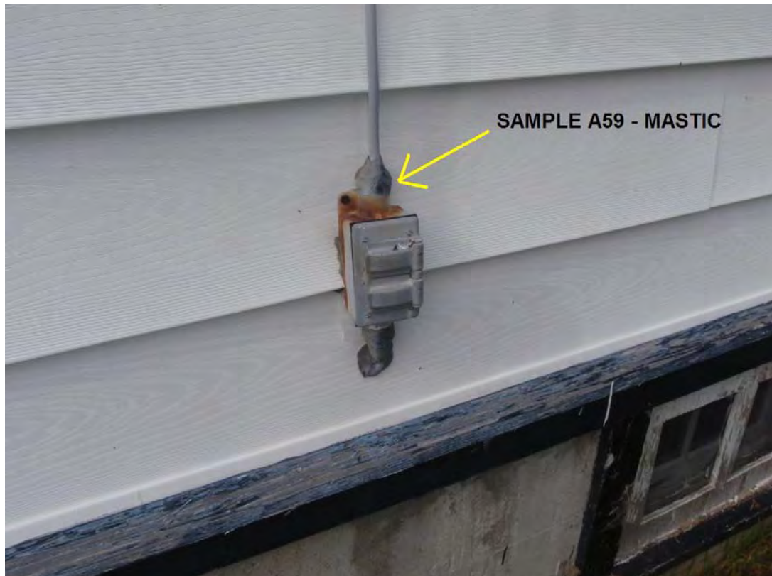
House #9 - 19 - Asbestos-containing mastic (A59) surrounding electrical boxes.
