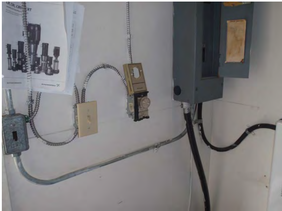
Pump House - 3 - Non-mercury containing thermostat on south wall.
