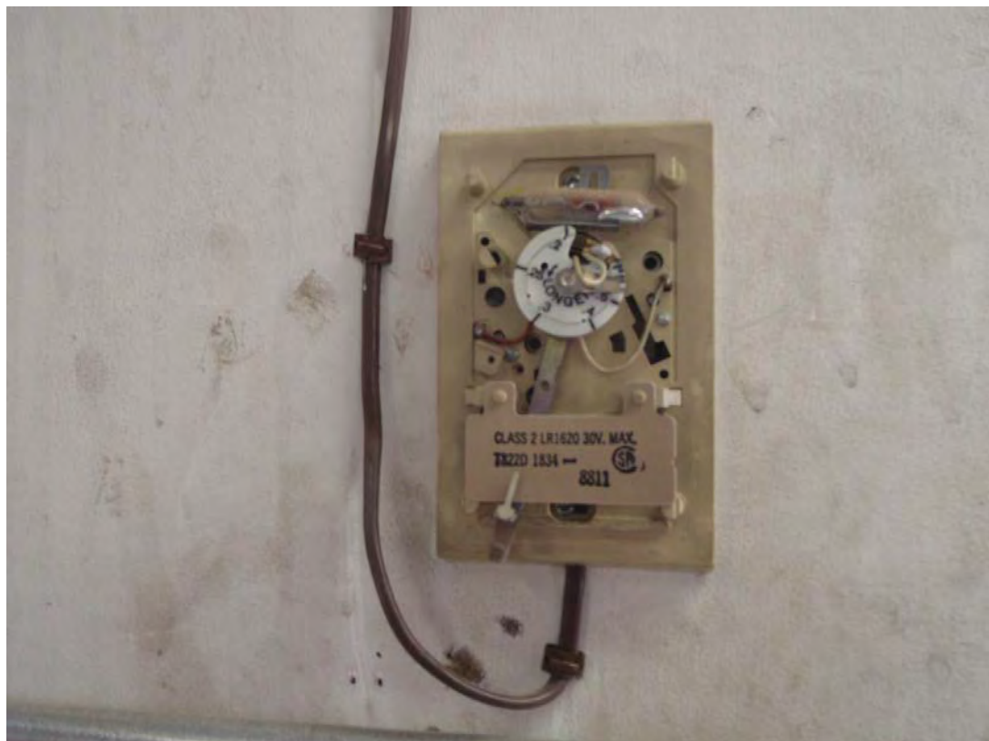
Secondary Examination Shelter - 10 - Thermostat (2 of 2) on east wall.
