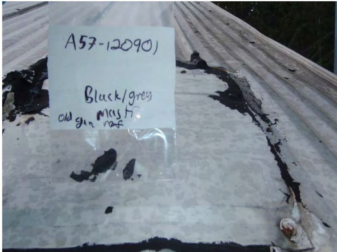
Generator Building - 15 - Asbestos-containing mastic (A57) on older area of metal roof.
