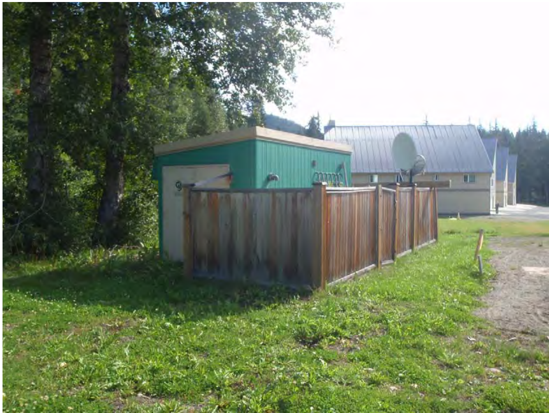
Remedial System Enclosure - 1 - Facing northeast.
