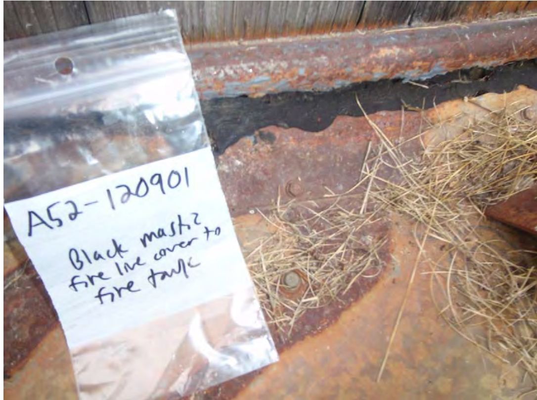
Water Storage Tank - 4 - Asbestos-containing mastic (A52) joining metal pipe covering to Water Storage Tank.
