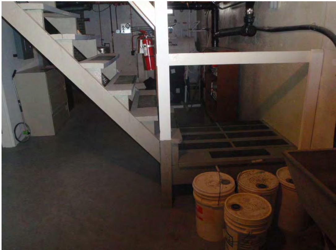
Customs Office - 8 - Various floor sealers and cleaners in basement electrical room.
