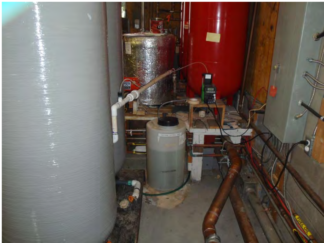
Generator Building - 6 - Chlorine tank and dosing pump for water treatment system.
