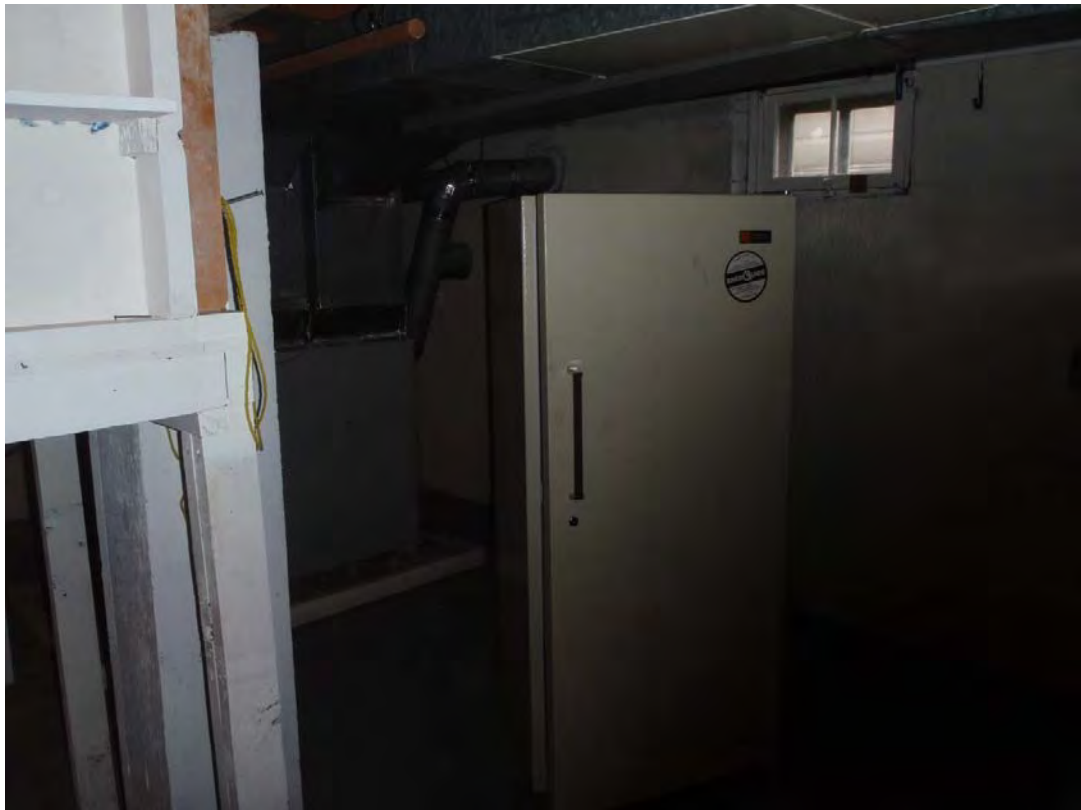
House #9 - 13 - Stand-up freezer in basement.
