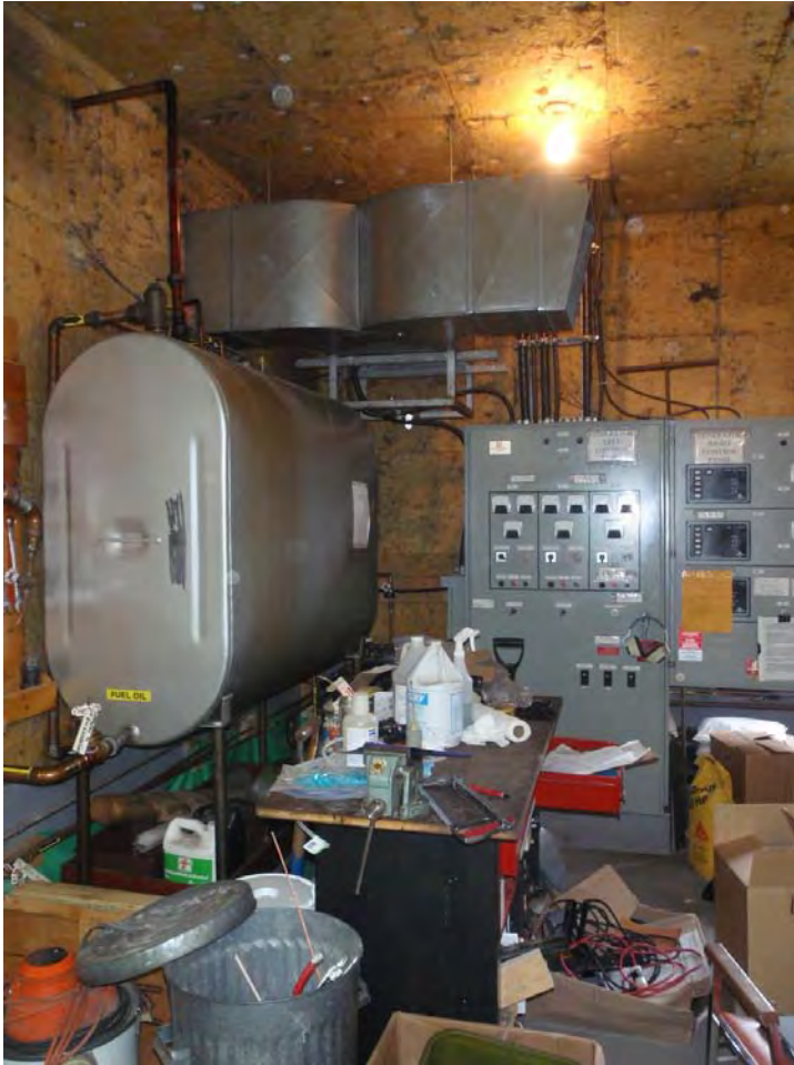
Generator Building - 7 - Diesel AST in southeast corner of building.
