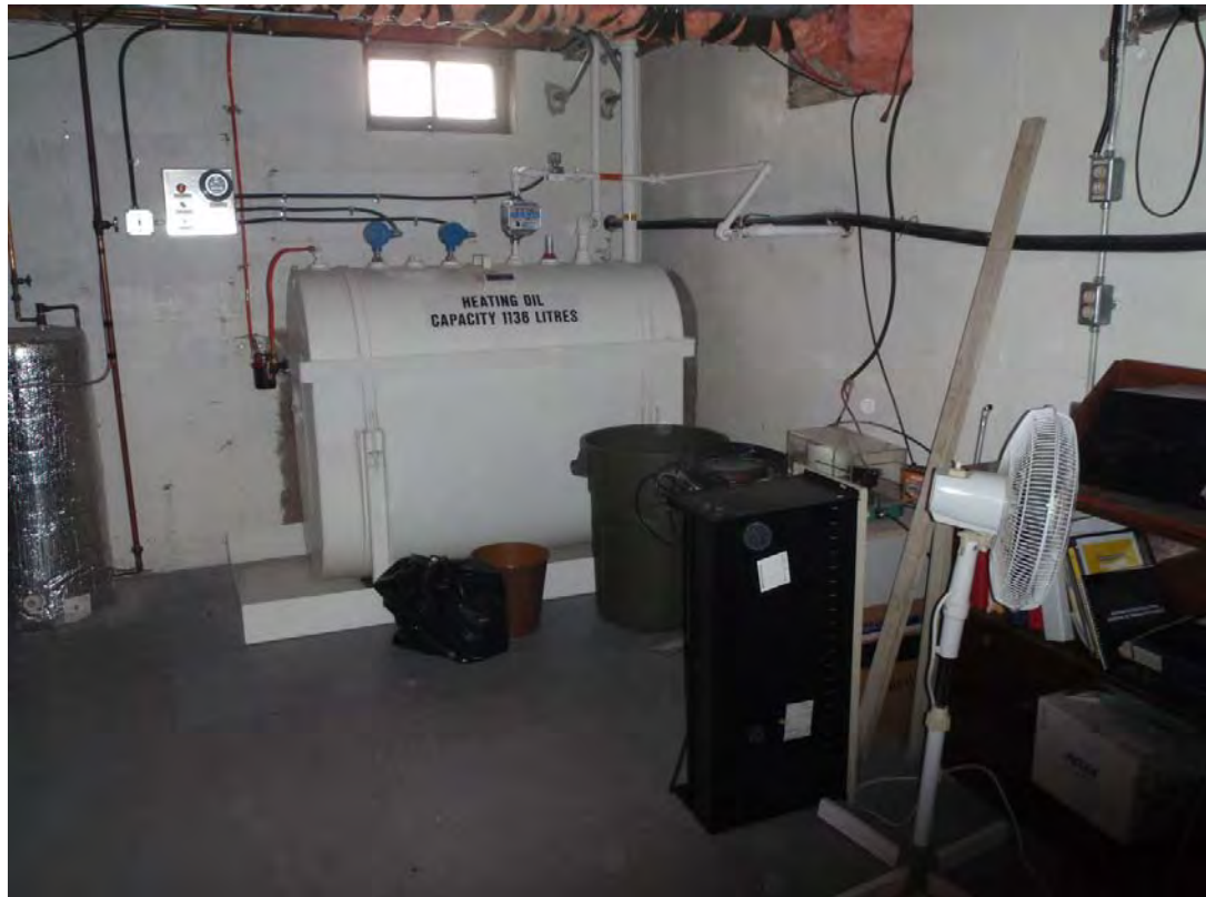
Customs Office - 6 - Heating oil tank in basement (northwest corner).
