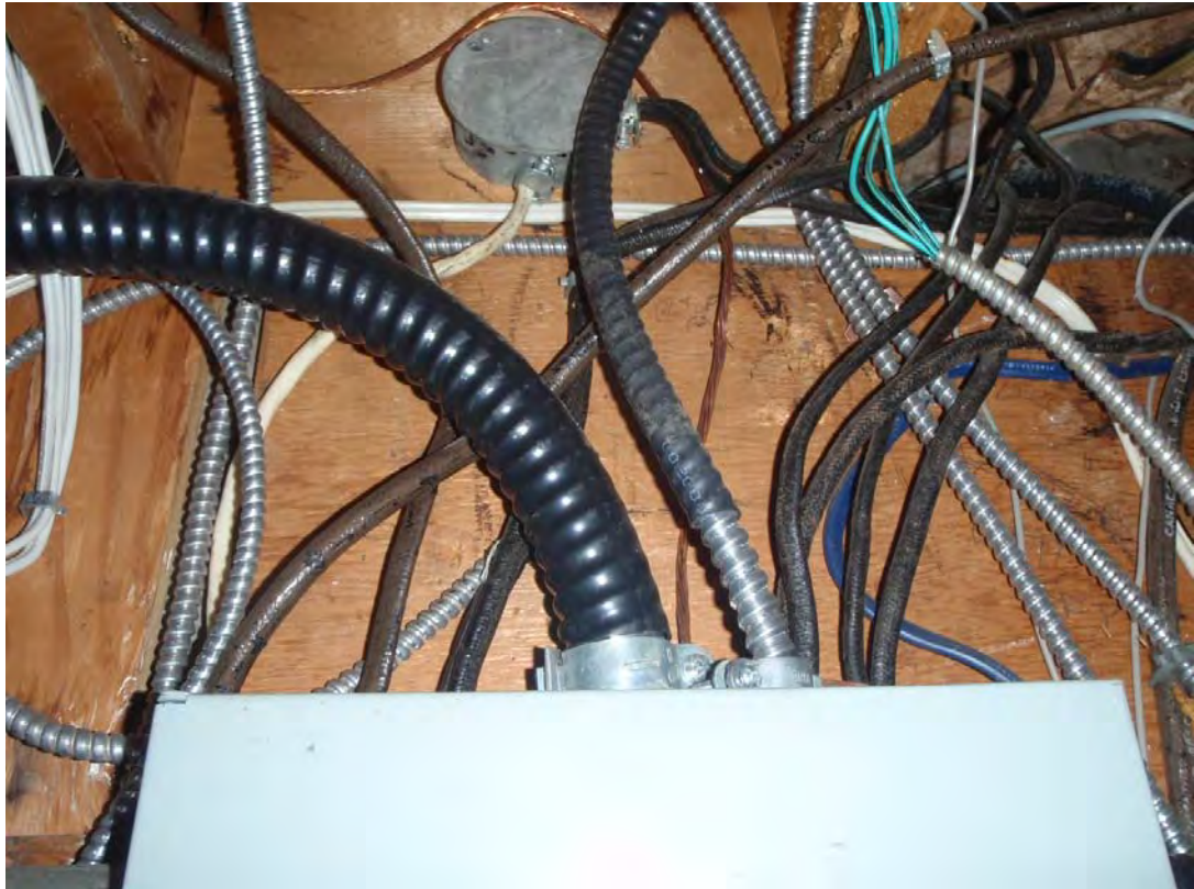
Customs Office - 7 - Old wiring in the basement electrical room.
