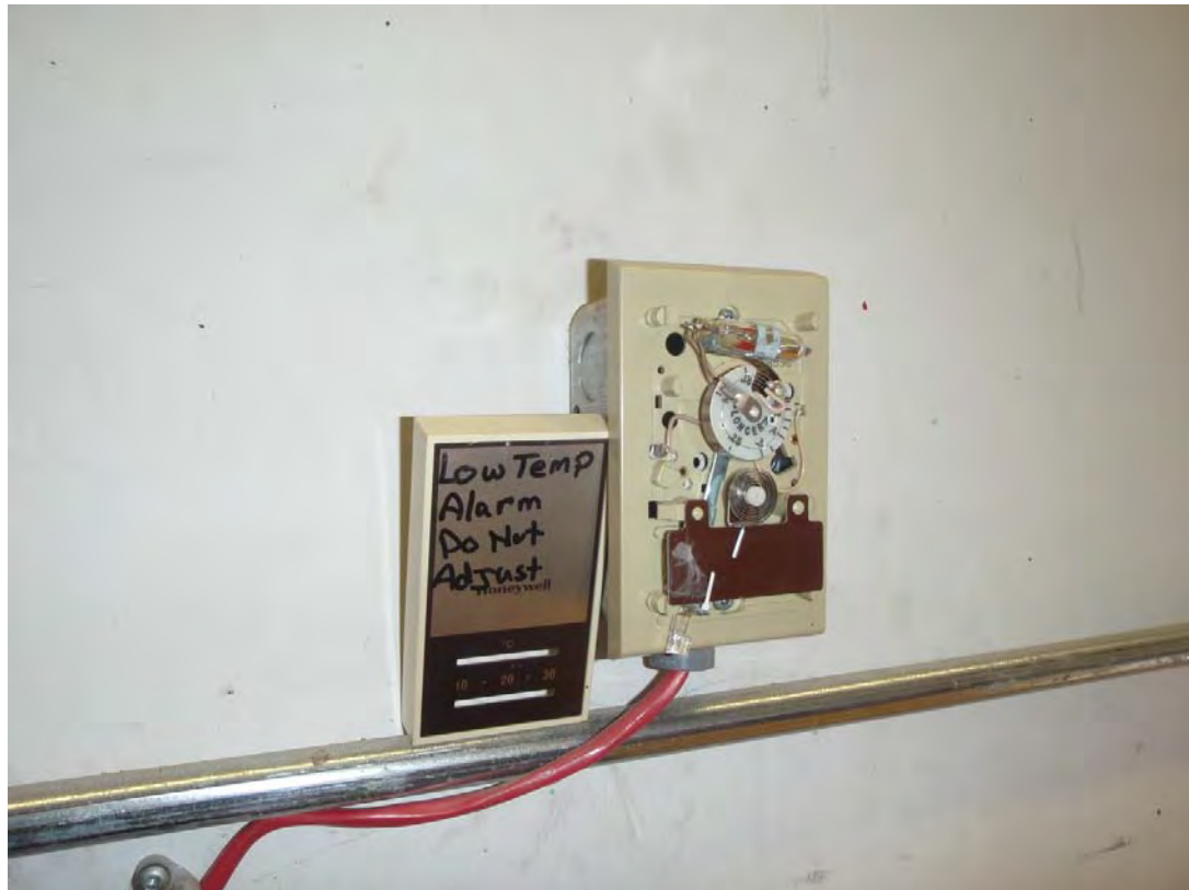
Secondary Examination Shelter - 9 - Thermostat (1 of 2) on east wall.
