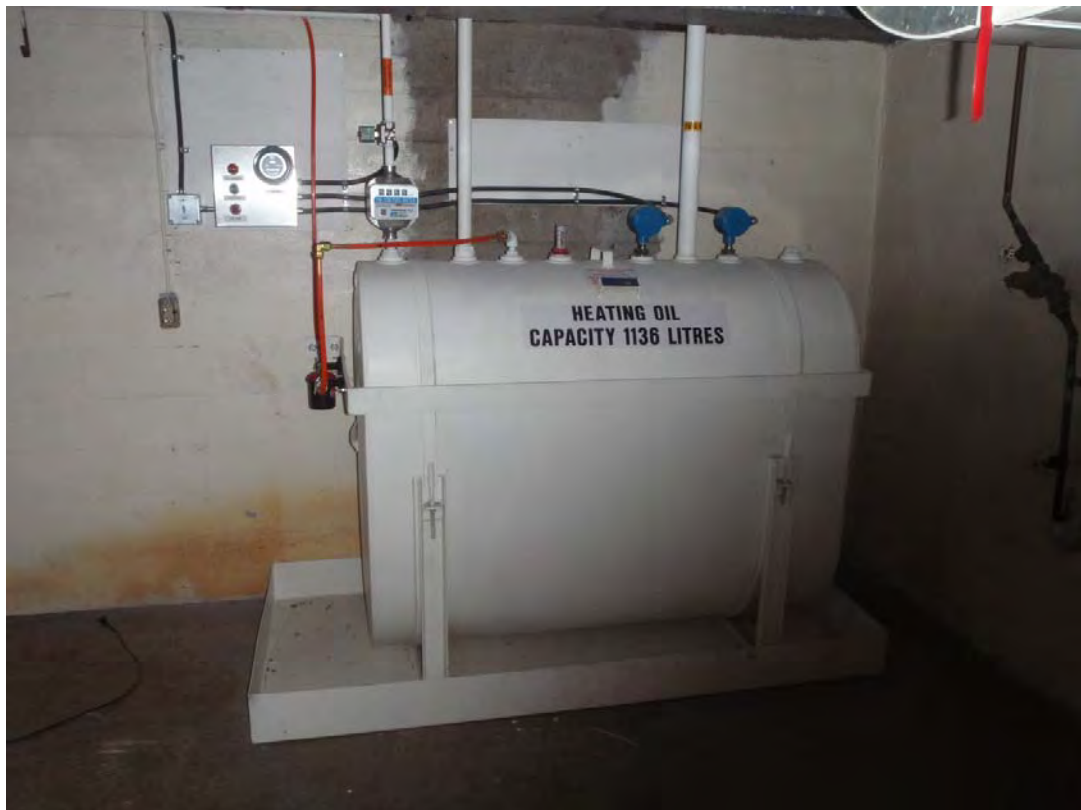
House #9 - 11 - Heating oil tank in southeast corner of basement.
