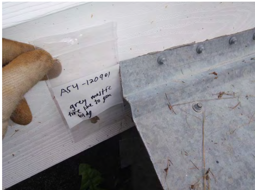
Water Storage Tank - 5 - Asbestos-containing mastic (A54) joining metal pipe cover to Generator Building.
