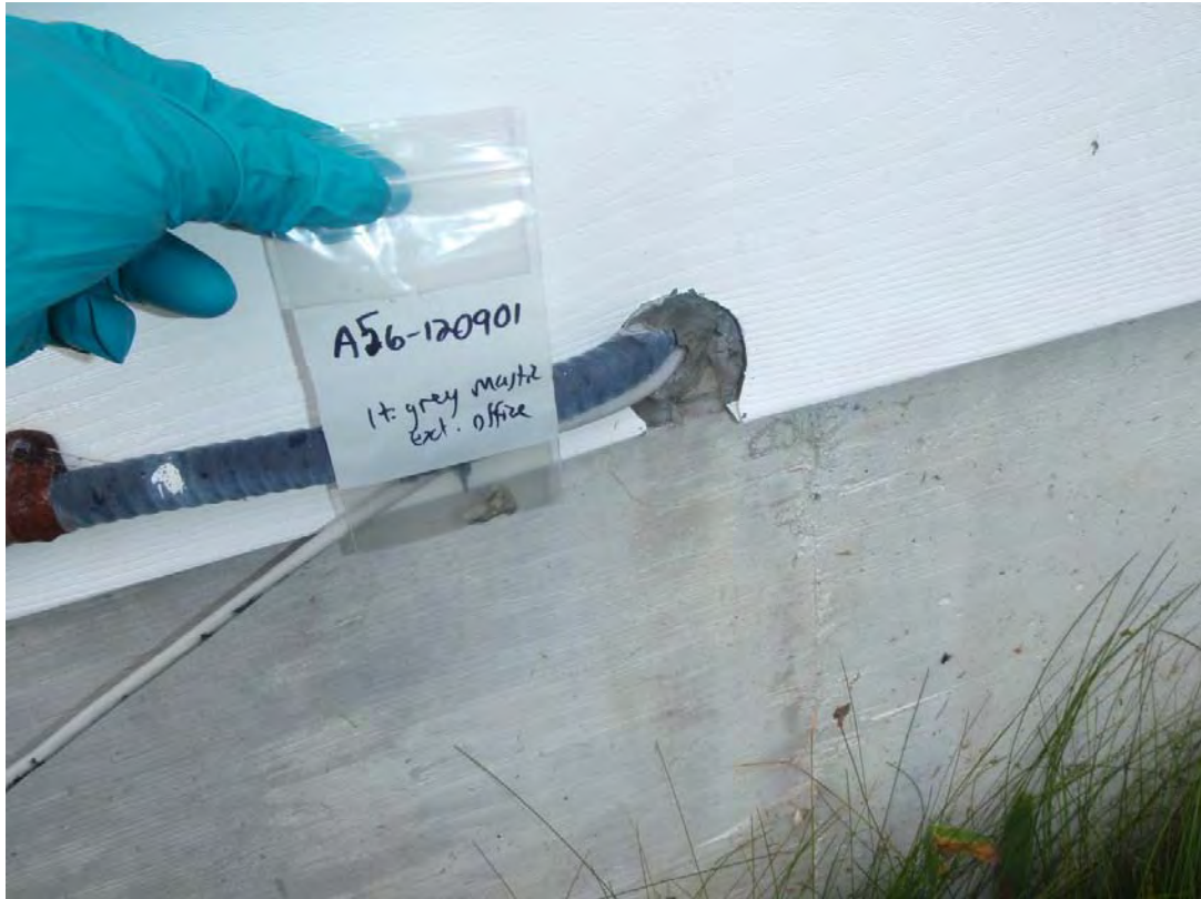
Customs Office - 15 - Asbestos-containing mastic (A56) surrounding conduit entering the building.
