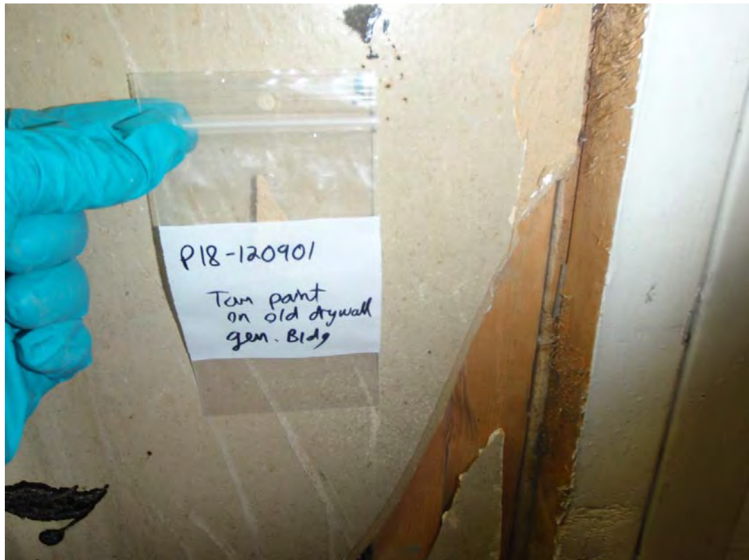
Generator Building - 16 - Lead-based paint on older area drywall.
