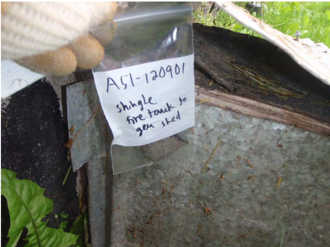
Water Storage Tank - 3 - Asbestos-containing shingle (A51) beneath metal cladding on ground piping.
