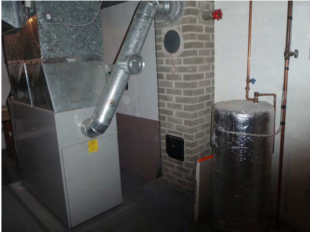
Customs Office - 5 - Furnace, chimney and hot water tank in basement.
