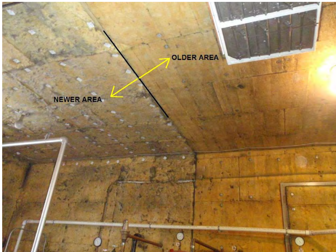
Generator Building - 3 - Separation between newer and older sections.
