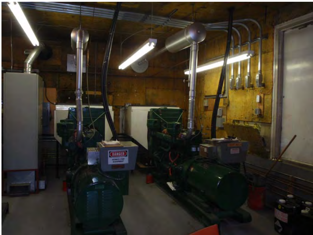
Generator Building - 8 - Back-up generators.
