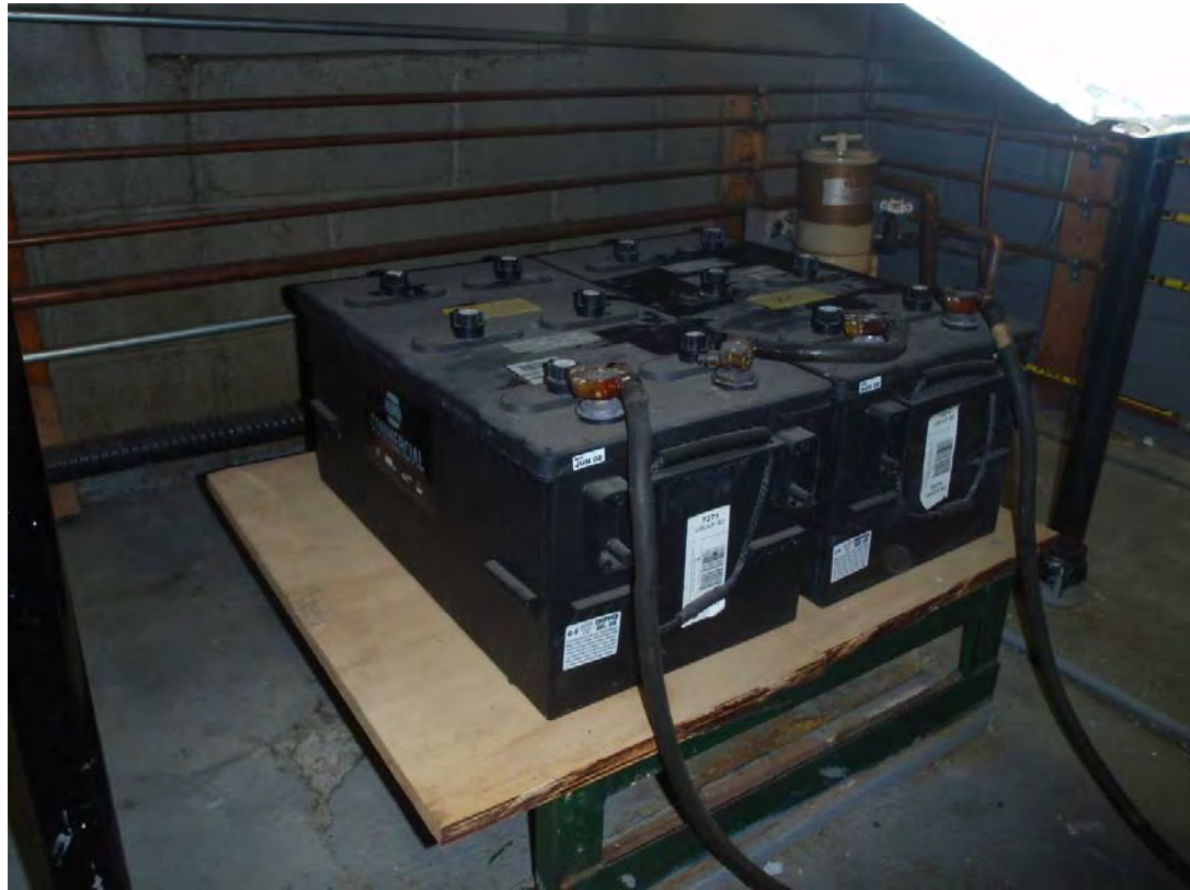
Generator Building - 9 - Lead batteries for back-up generators (2 for each generator).
