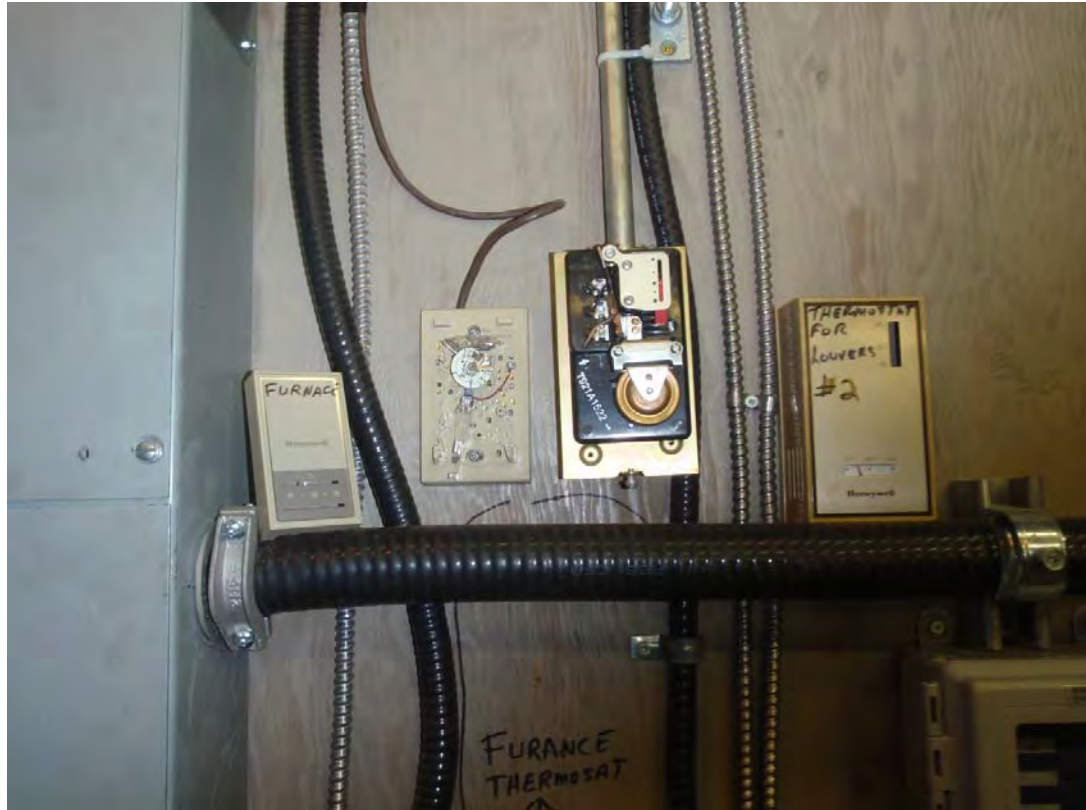
Generator Building - 11 - Mercury containing thermostat on west wall.
