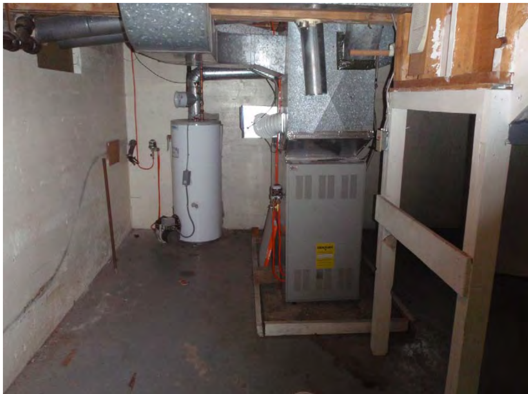
House #9 - 7 - Furnace and hot water tank in basement.
