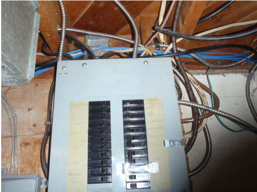
House #9 - 12 - Older wiring in basement.
