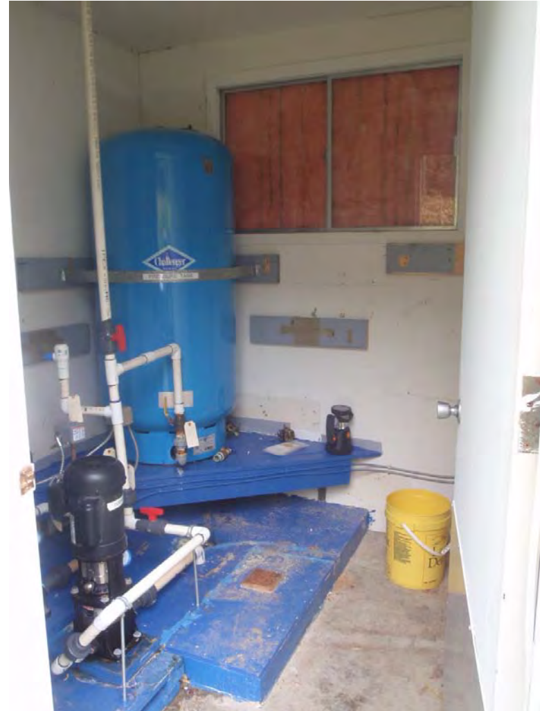
Pump House - 2 - Interior of pump house.
