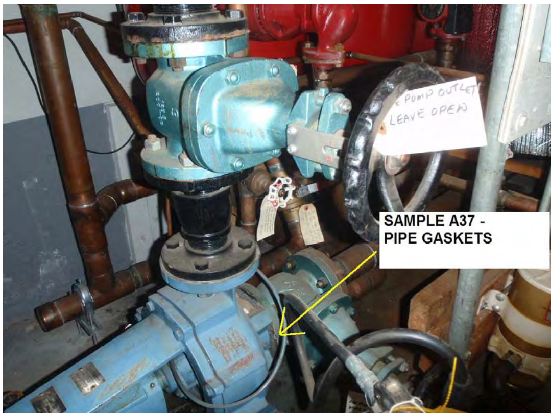
Generator Building - 12 - Asbestos-containing pipe gaskets (A37) in fire suppression system piping.
