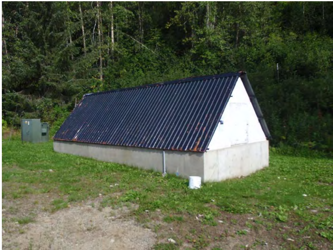
Main Fuel Storage Tank Enclosure - 1 - Facing northwest.
