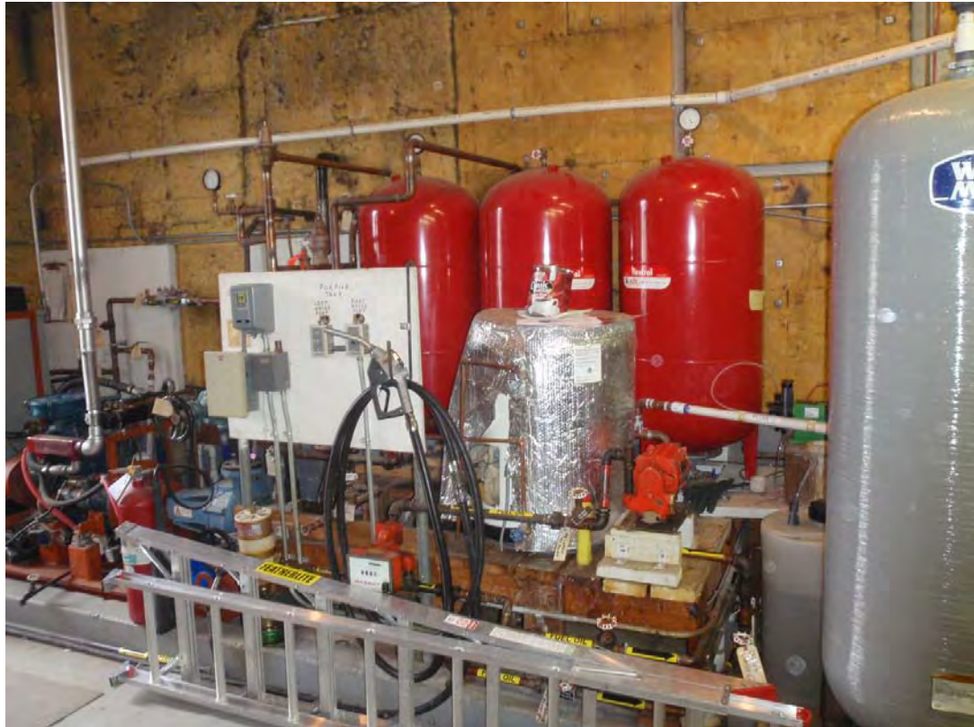
Generator Building - 5 - Water treatment and fire suppression system.
