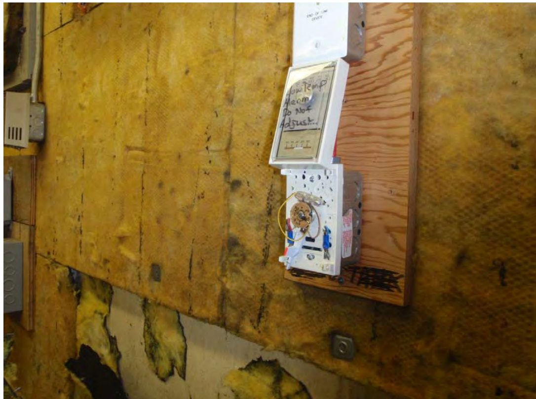
Generator Building - 10 - Mercury containing thermostat on east wall.
