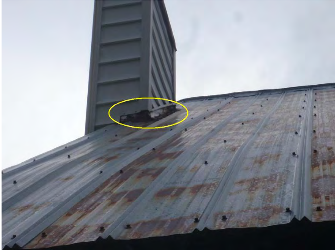
House #9 - 20 - Potentially asbestos-containing mastic (similar to A59) around chimney flashing.
