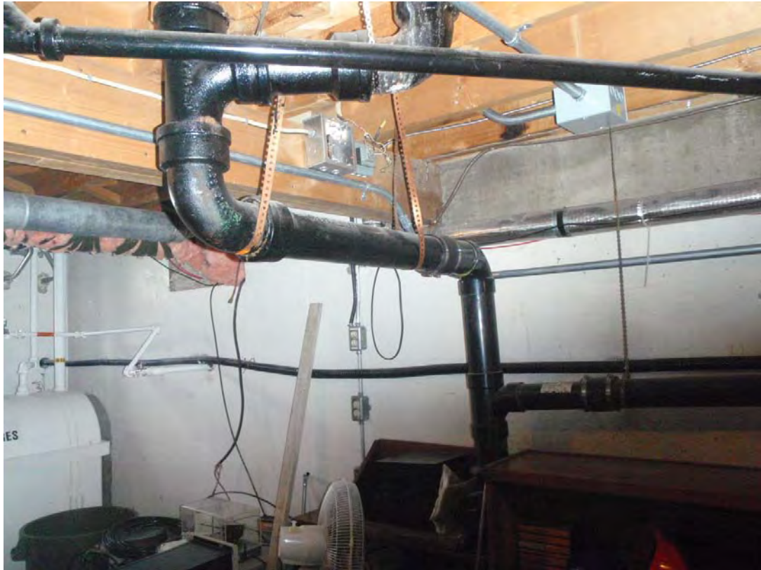
Customs Office - 9 - Cast iron piping in basement.
