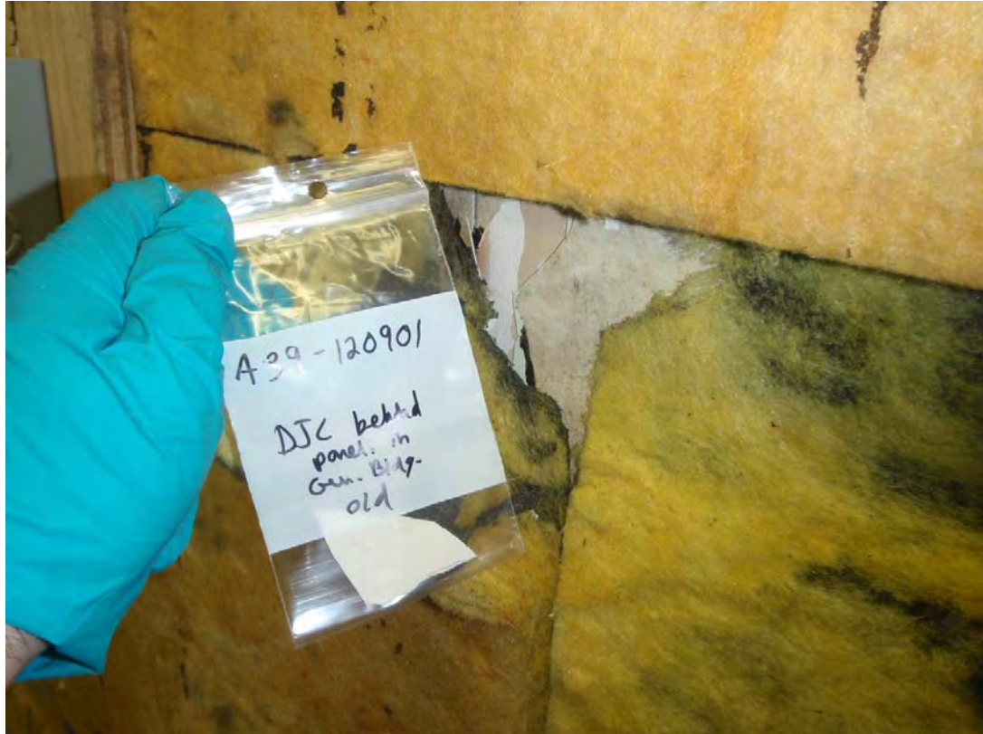
Generator Building - 13 - Asbestos-containing drywall joint compound (A39) on older area drywall.
