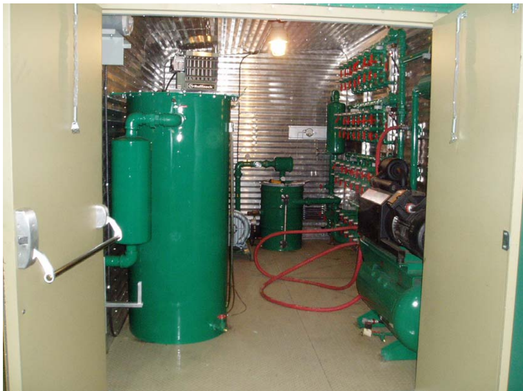
Photograph 20: Air sparge and SVE equipment inside enclosure.
