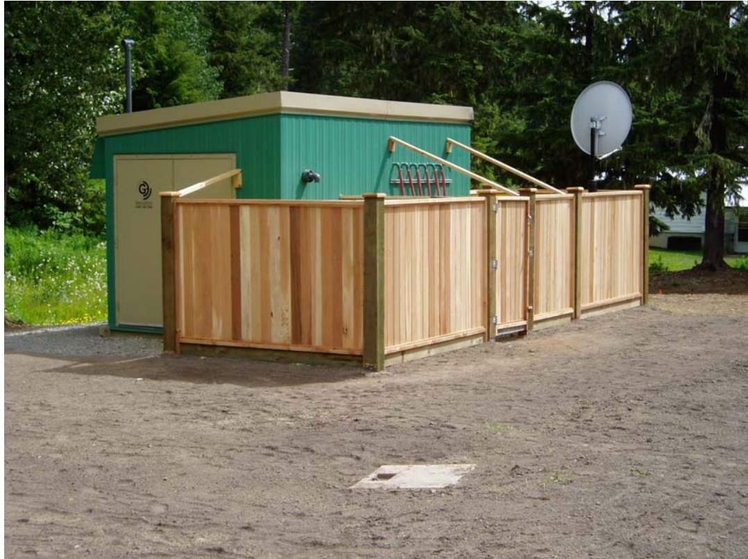
Photograph 19: Remediation equipment enclosure.
