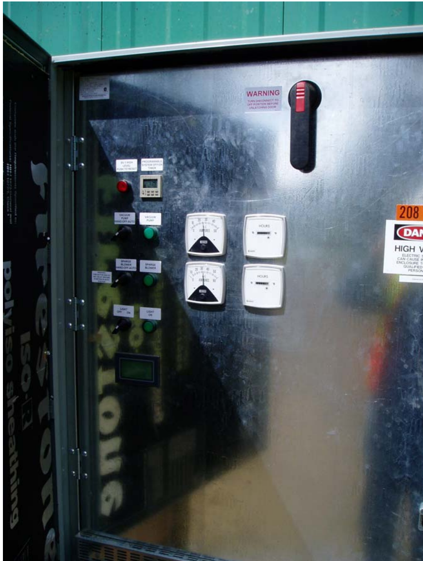
Photograph 26: Equipment control panel.
