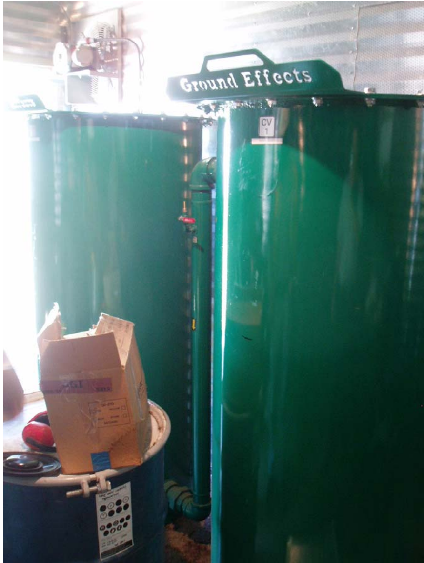
Photograph 25: Air phase carbon vessels.
