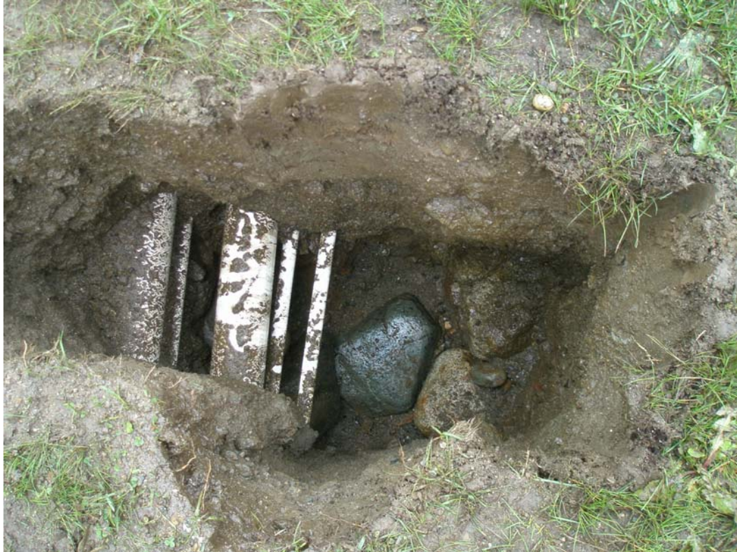
Photograph 11: Exposed remediation system piping in BH09-12.
