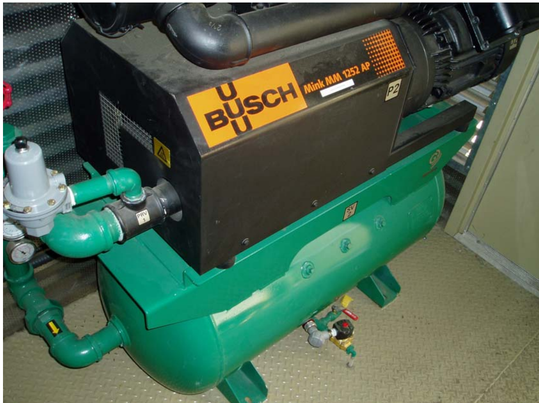
Photograph 22: Air sparge blower.
