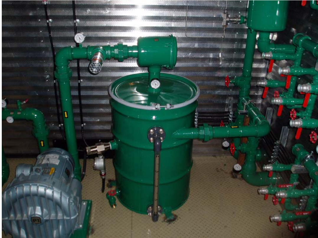
Photograph 21: SVE blower and inlet knockout.
