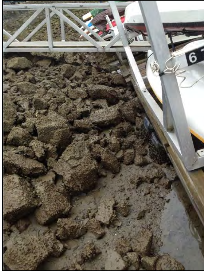
Photo 12 View of the Rock Slope and a Gangway Leading to a Stranded Floating Dock at Low Tide adjacent to the Maritime Market Boardwalk (Photo Courtesy of Parsons)
