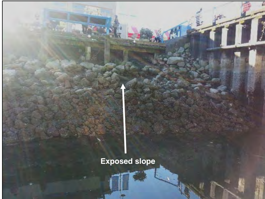
Photo 10 Rock Slope Protection to be Repaired along the Public Market Boardwalk
