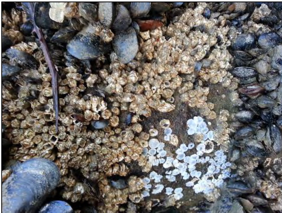
Photo 7 Close-up View of a Wooden Pile Encrusted with Marine Life, Predominantly Barnacles and Mussels
