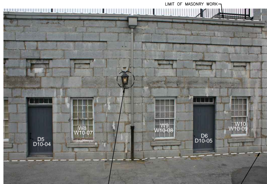
CAREFULLY DISMANTLE, TURN OVER TO OWNER FOR REPAIRS TO BE COMPLETED (BY OTHERS) AND RE-INSTALL AFTER MASONRY REPAIRS ARE COMPLETE
