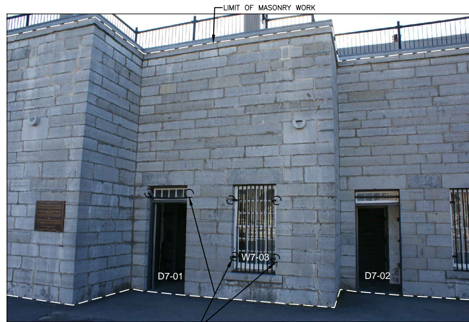
BAR GRILL ANCHORAGES TO BE REVIEWED BY DEPARTMENTAL REPRESENTATIVE ON SITE. IF ARE CORRODING, REMOVE ANCHORS, REPAIR MASONRY AND RE-INSTALL BAR GRILLS WITH NEW STAINLESS ANCHORAGES
