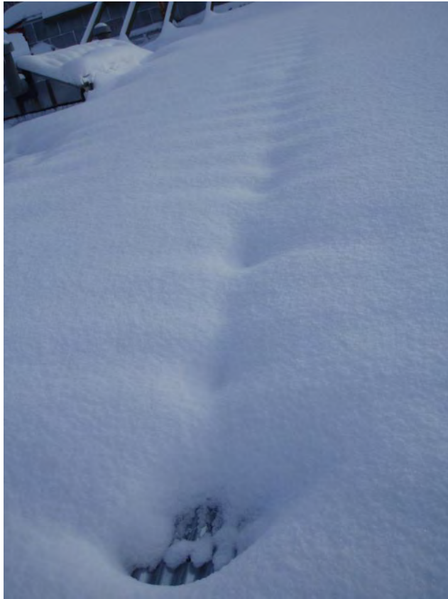
Figure 5: Roof Heat Loss (Feb. 2013)
