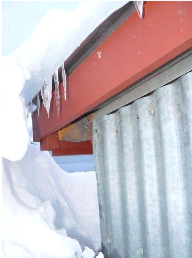
Figure 9: Ice damming at rear of roof
