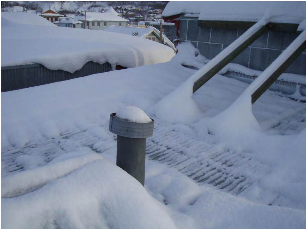
Figure 6: Roof Heat Loss (Feb. 2013)
