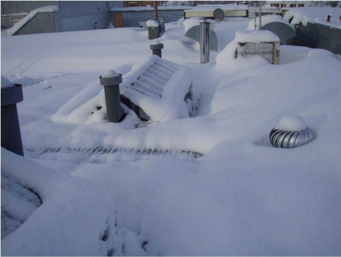
Figure 7: Roof Heat Loss (Feb. 2013)
