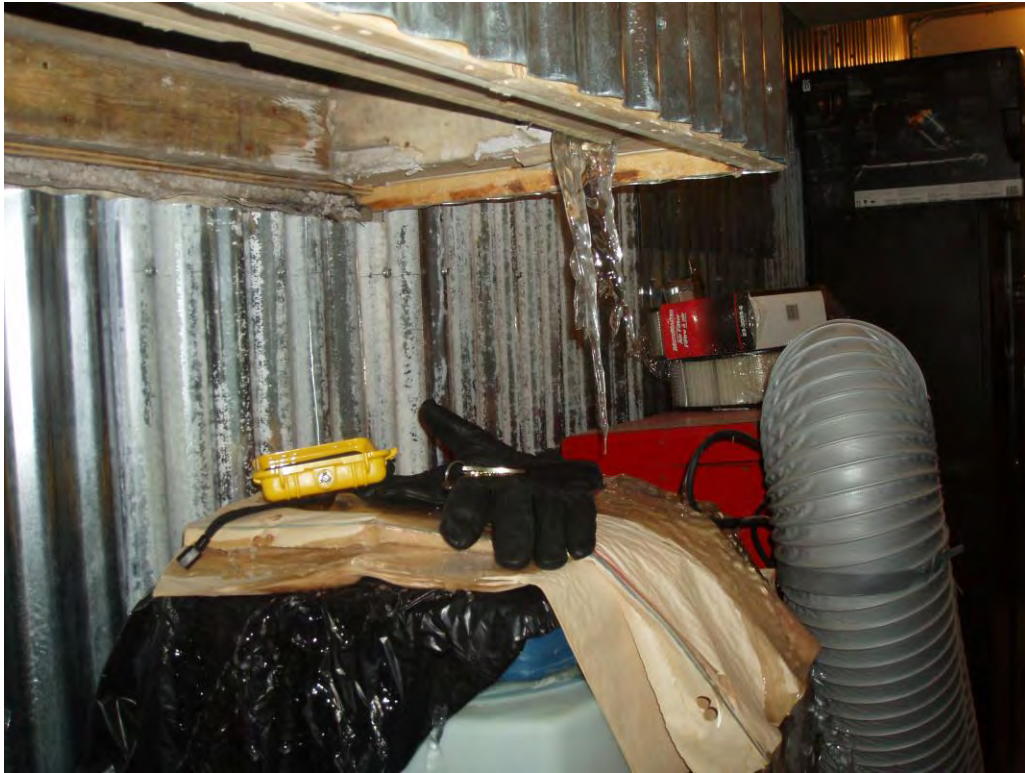
Figure 11: Leakage in mechanical room, transition way to Annex
