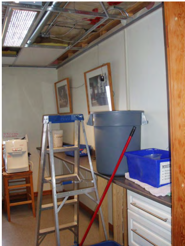
Figure 10: Leakage in kitchen, rear of roof
