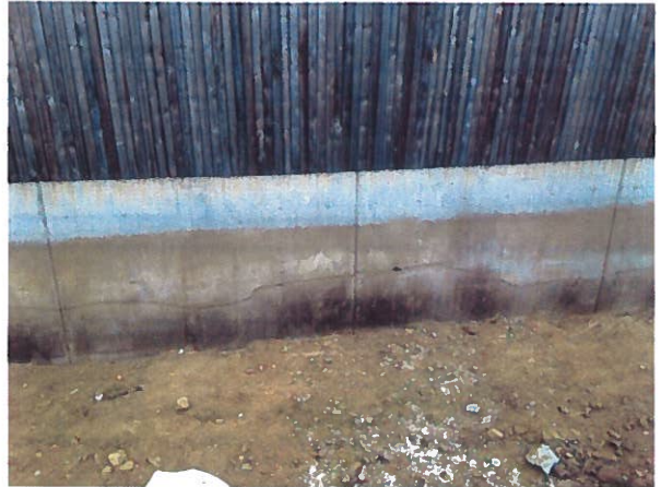
Fissure horizontale au centre du mur Horizontal crack at the middle of the wall
