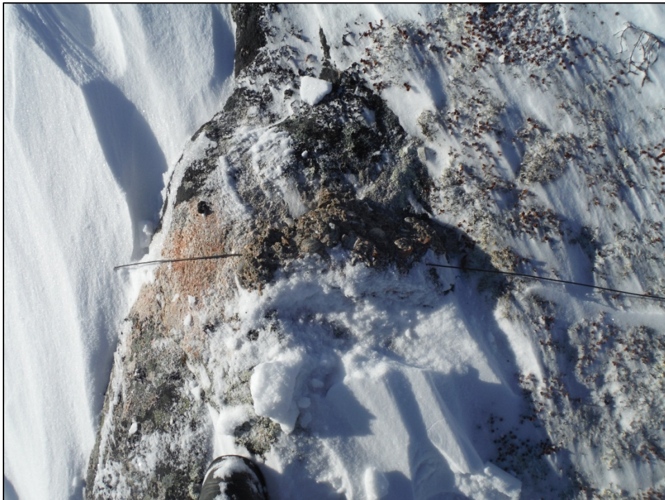
Photograph 14 – Grounding wire encapsulated in cement
