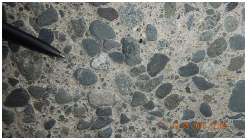
Figure 3 - Typical concrete Raceway Surface Condition 3/3
