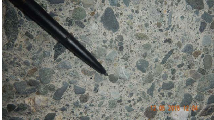
Figure 1 - Typical Concrete Raceway Surface Condition 1/3
