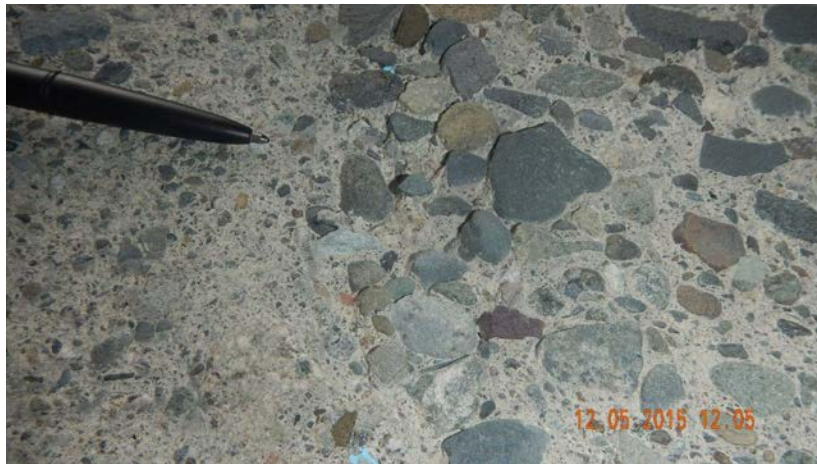
Figure 2 - Typical Concrete Raceway Surface Condition 2/3
