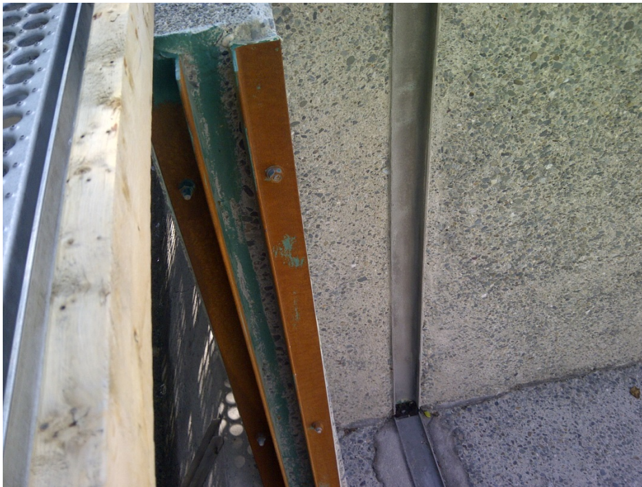
Figure 7 - Additional embedded metal within the channel
