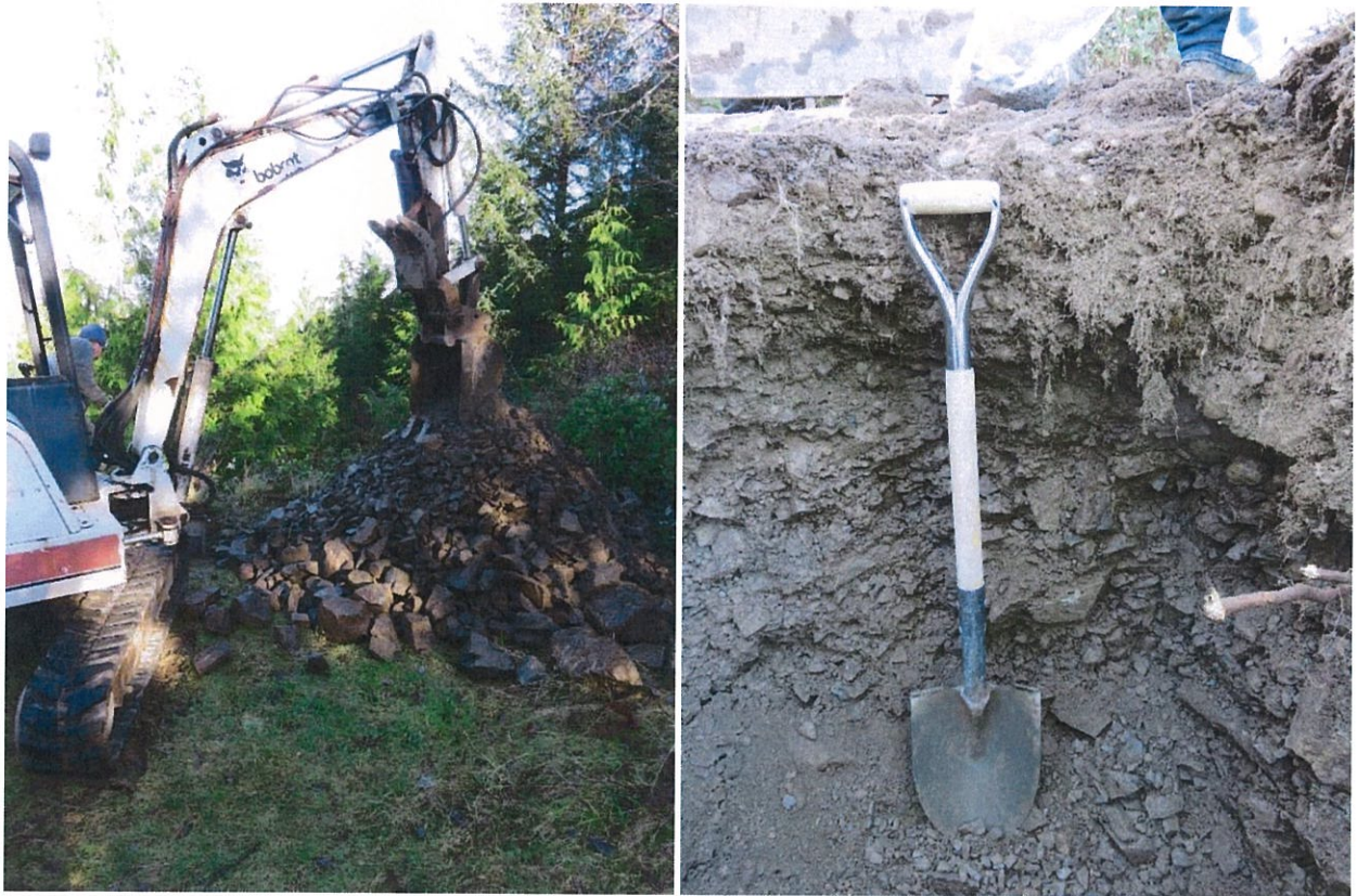
Photo 6 and 7 – Excavator with material removed from test pit and exposed rock fill within the top 1.2 m.
