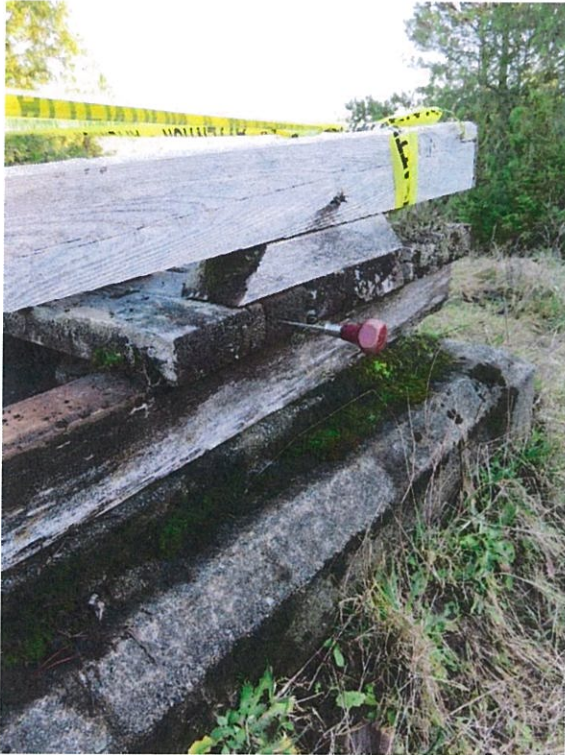
Photo 10 – Decay of decking boards ranged from 10 to 100 mm.
