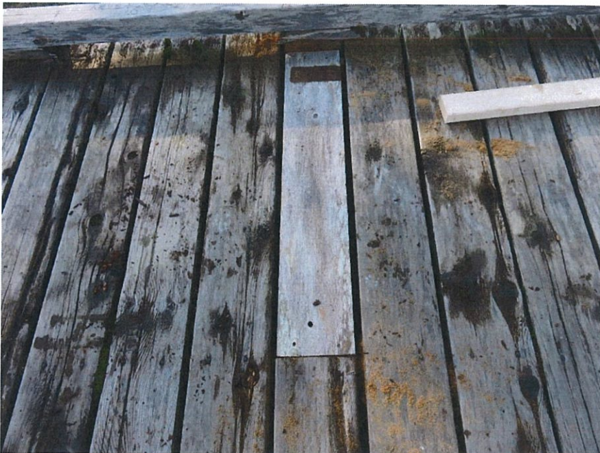
Photo 9 – Trip hazard in top south platform southwest corner removed after replacement of board.
