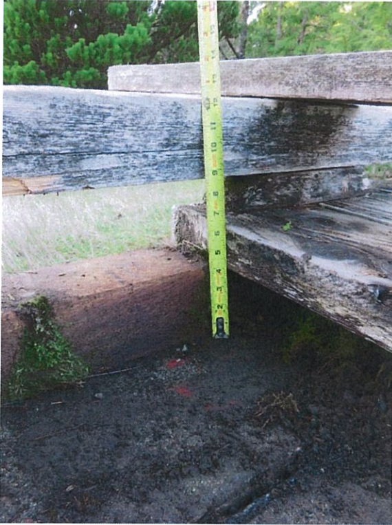
Photo 3 – Typical platform construction with sleeper in direct contact with footing / slab on grade.
