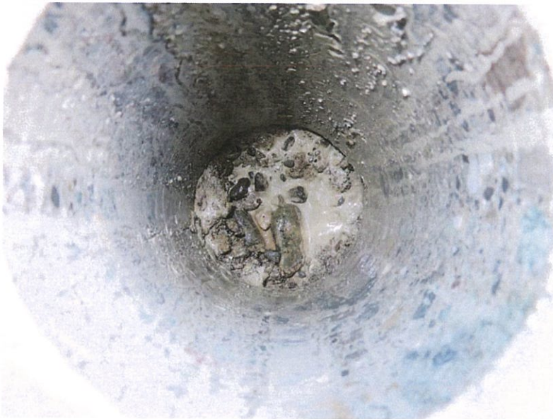
Photo 13 – Material below core hole in slab on grade.
