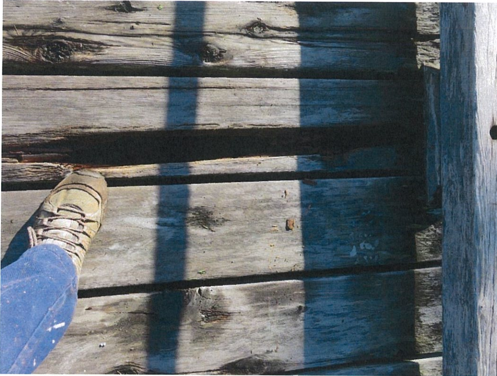
Photo 8 – Trip hazard in top south platform southwest corner.
