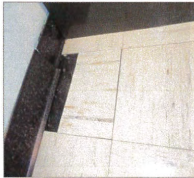
Photo 3. Asbestos-containing 9"x 9" vinyl floor tile. Mastic does not contain asbestos. (sample 0007A-C)
