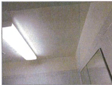
Photo 1, B-100, plaster containing chrysotile asbestos in plaster base coat(sample 0003A-B)
