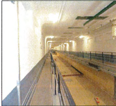
Photo 4 – Cementitious parge on walls and ceiling, containing chrysotile asbestos, room 120, building M-22, (LAB ID 1507733 Sample 0001A-C)
