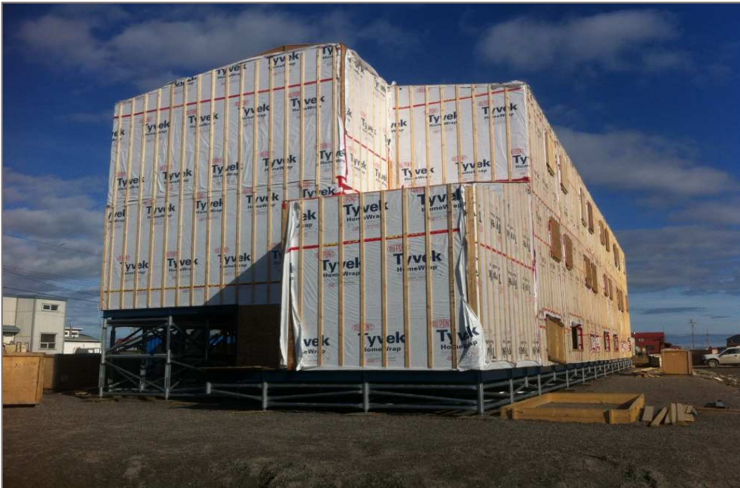
Photo 12: This 5-plex housing unit in Arviat is being constructed using a tridetic multipoint foundation system.
