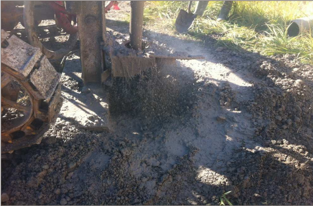
Photo 9: Water can be seen being blown from Probehole 2 during drilling. Water was observed at a depth of 2.0 m within the probehole.
