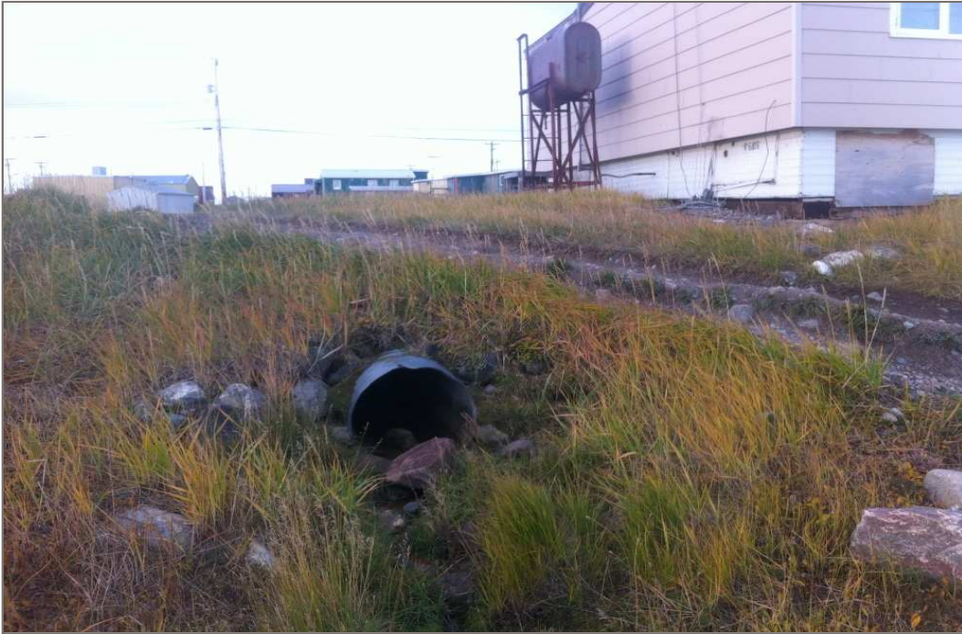
Photo 5: Looking south through the project site at the culvert outlet and fuel tank.
