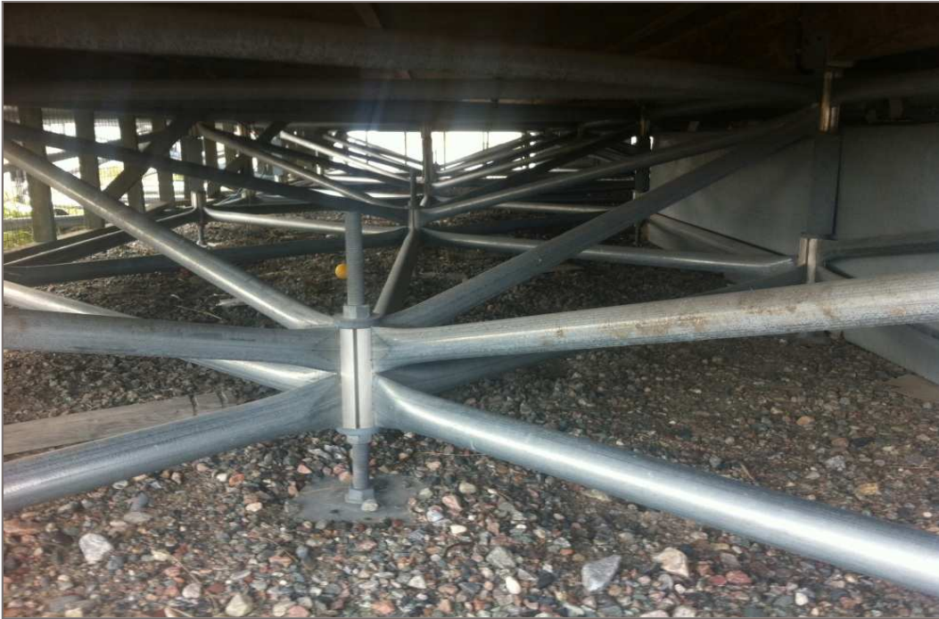
Photo 13: Close up of the multipoint connector system utilized by the triodetic foundation type.
