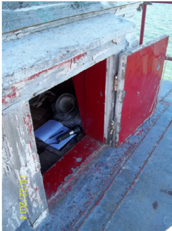
Photo 17: View from upper exterior walkway looking back to hatch door on east side. Door closes but does not seal off opening fully.
