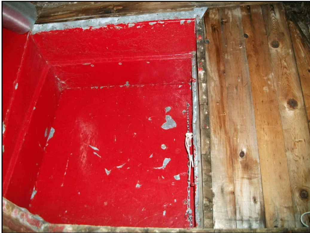
Photograph 8: Red lead-based paint (fair condition) on interior metal surface on 3rd floor of Old Light Tower.
