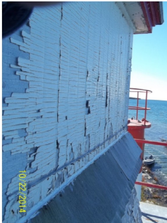
Photo 22: North wall face at level above exterior walkway, paint in poor condition.
