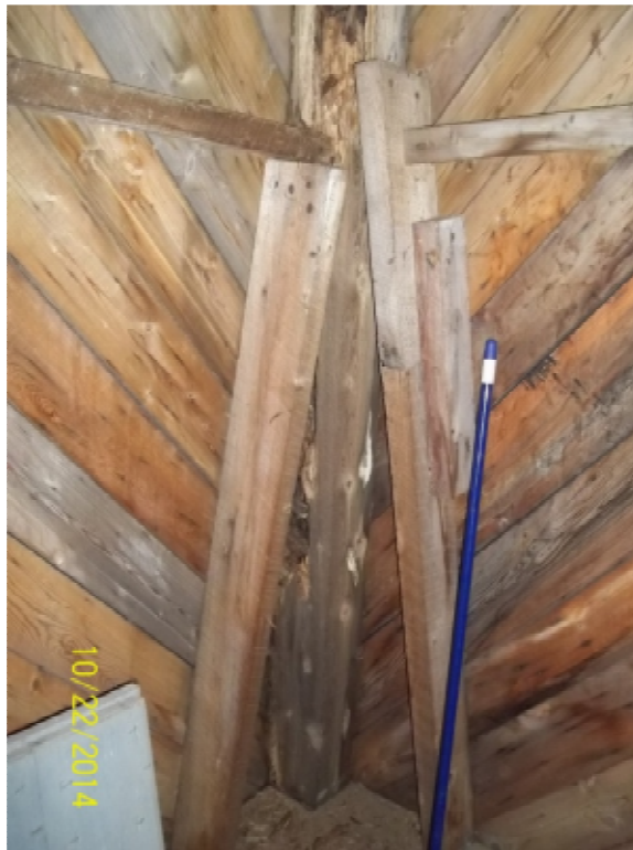
Photo 28: View of southeast corner post which is rotting.
