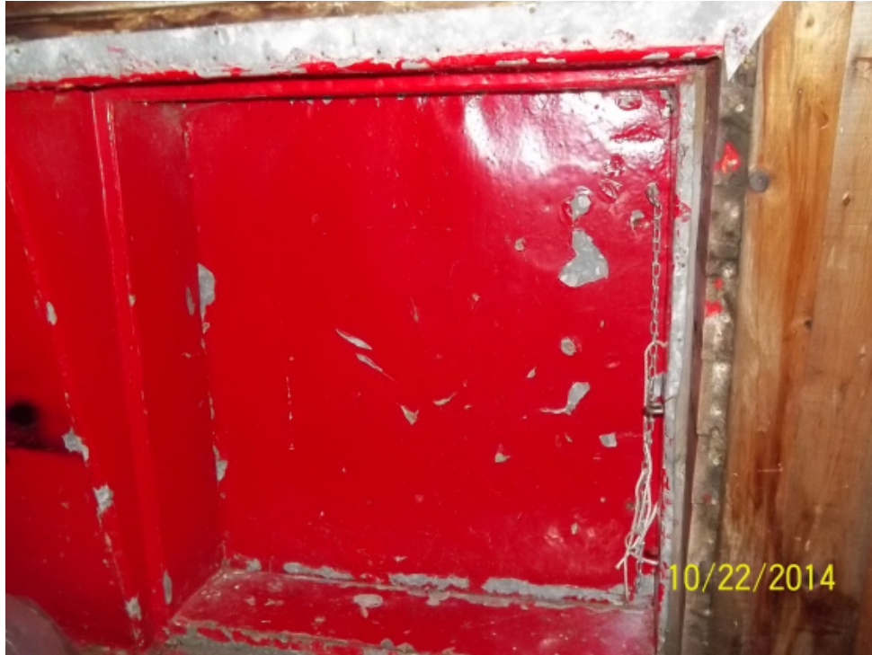
Photo 37: Interior view of side wall access door which goes from the high level floor out to the exterior perimeter walkway.
