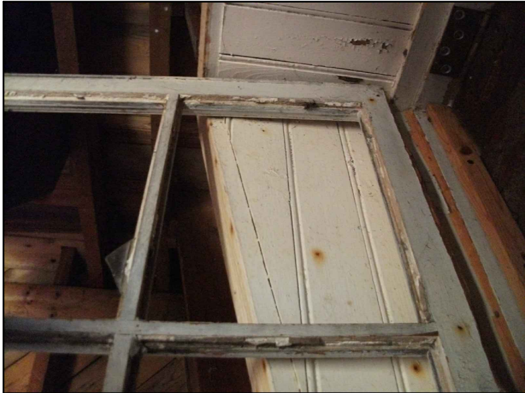
Photograph 14: White caulking (non-ACM) on 1st and 2nd floor windows of Old Light Tower.
