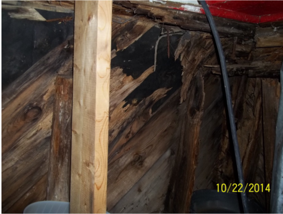
Photo 35: Upper level, missing exterior sheathing due to wood rot.
