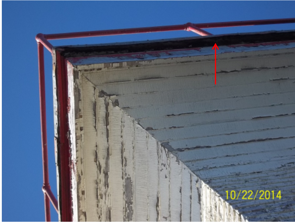
Photo 15: Looking up at underside of lighthouse soffit, decayed wood along edge, under metal roofing.
