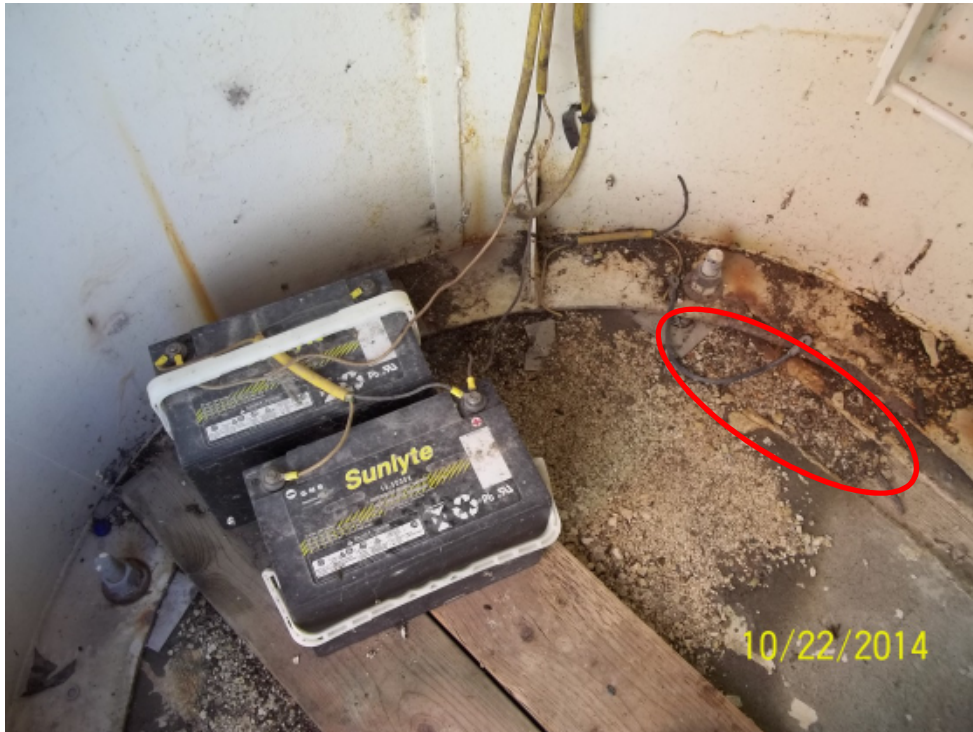
Photo 44: Base of steel tower with storage batteries for solar system. Note drainage channel in concrete base (circled 1 of 2).
