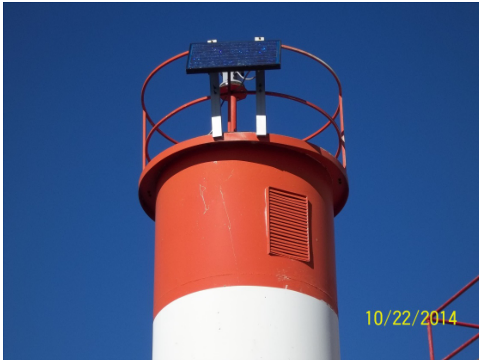
Photo 42: Top of steel tower showing solar panel on south side.
