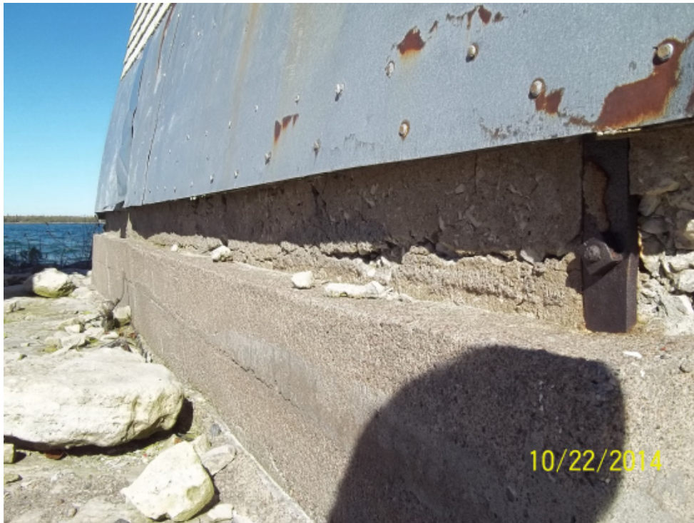
Photo 8: Lighthouse southwest corner of foundation, with steel anchorage in foreground and deteriorated concrete foundation wall, with secondary pour on outside showing top ledge. Steel sheet covering wood shake cladding.
