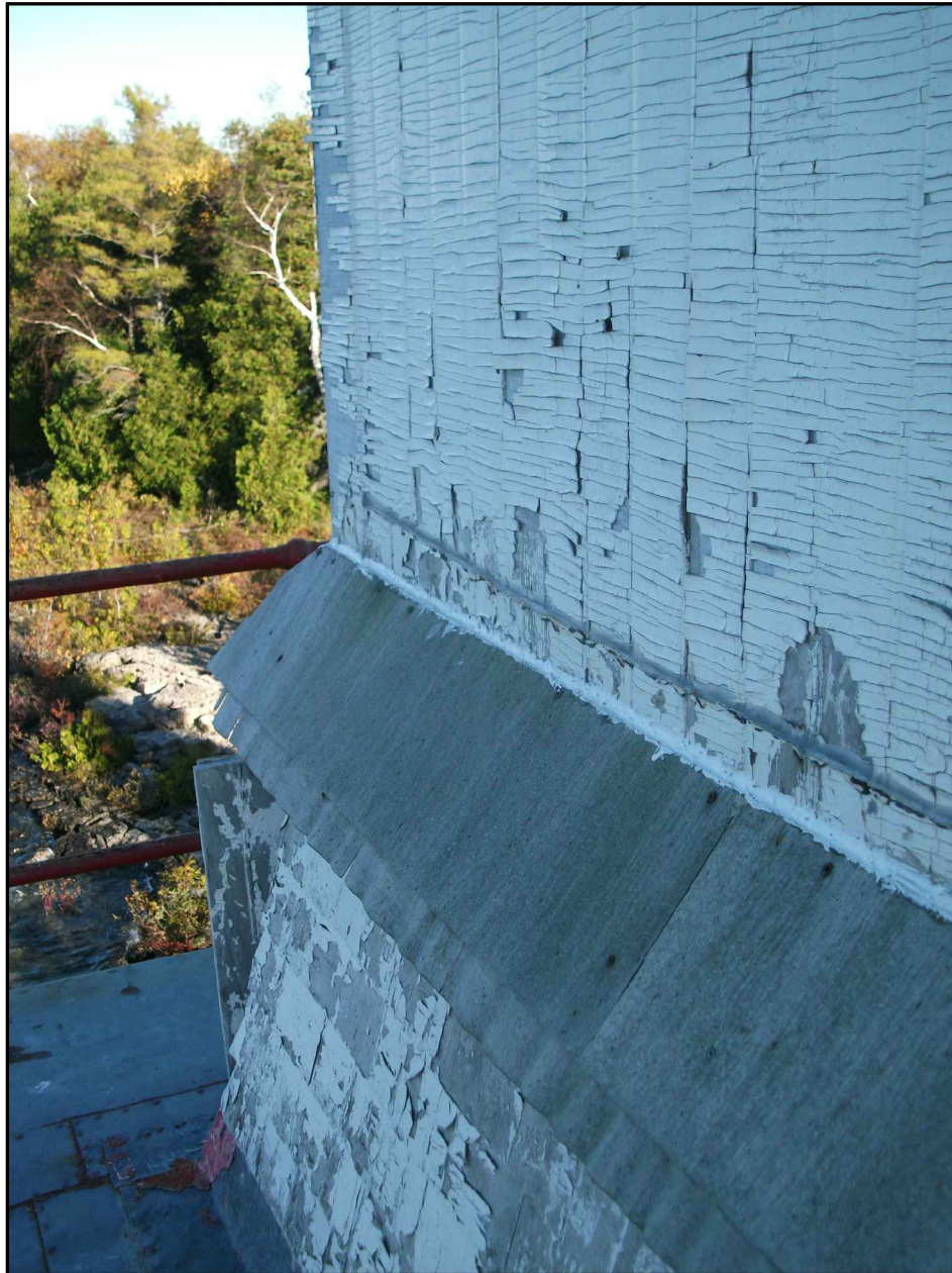
Photograph 9: White lead-based paint on exterior wood surface on 3rd floor of Old Light Tower.
