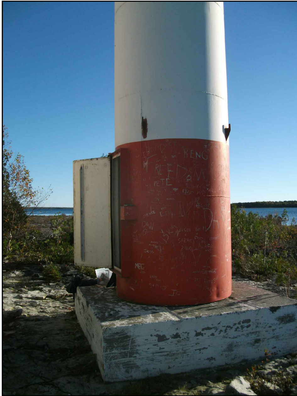
Photograph 13: Red lead-based paint (good condition) on exterior metal surface of New Light Tower (looking south).
