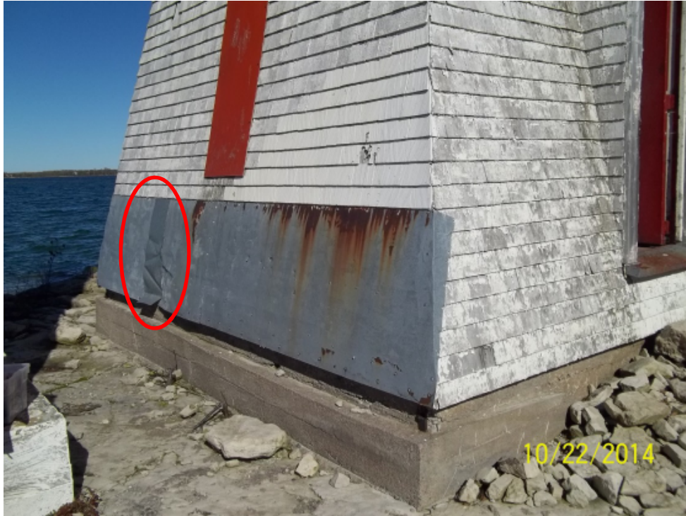
Photo 7: West side of entrance with sheet steel siding, notice impacted area, and rusting along top edge. Repainted/replaced wood shingles.
