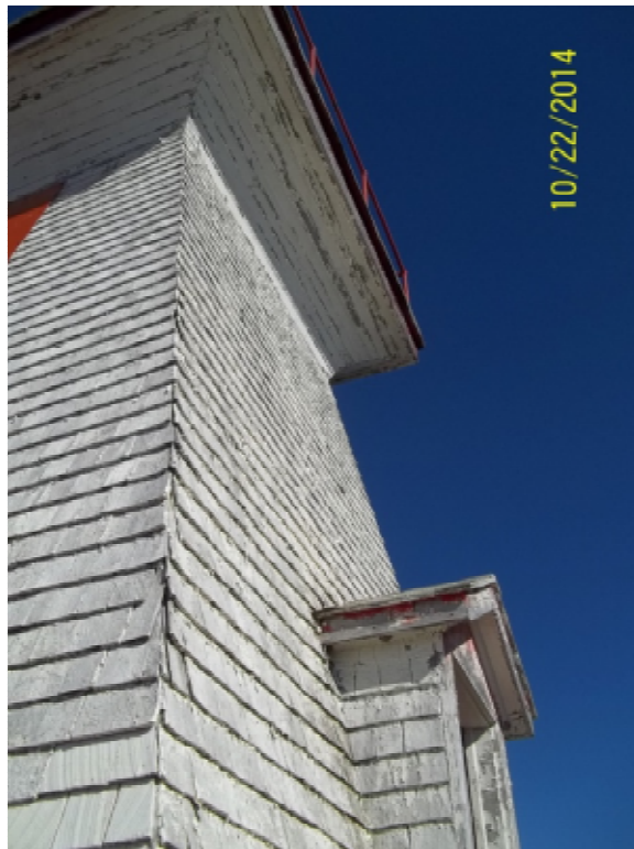
Photo 13: East elevation of lighthouse exterior wall, generally poor paint condition.
