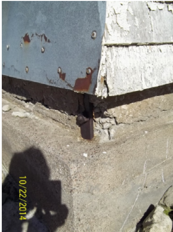
Photo 9: Deteriorating foundation wall at southwest corner.
