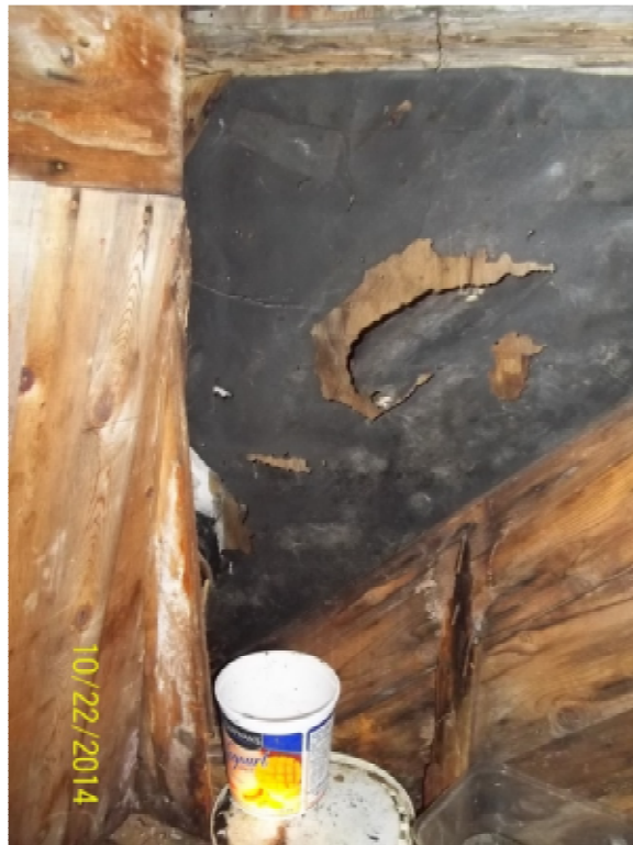
Photo 34: High level southeast corner, some exterior sheathing missing or rotten. Back side of exterior black building paper evident.
