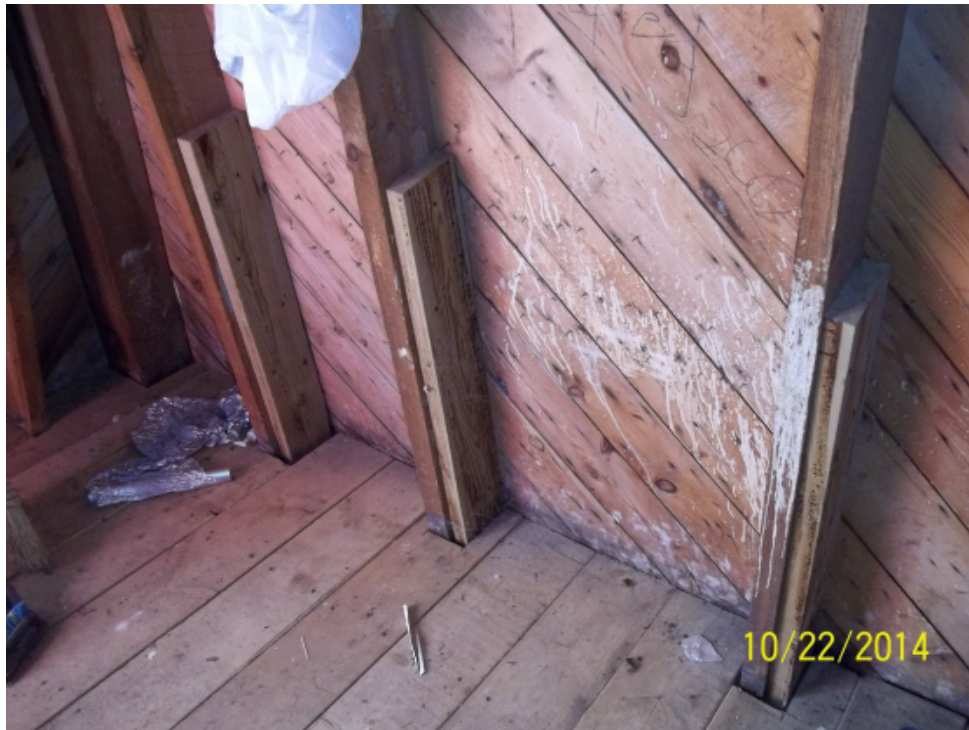
Photo 24: View of interior wall framing at ground level, with base floor in very good condition and pressure treated spliced studs along wall.
