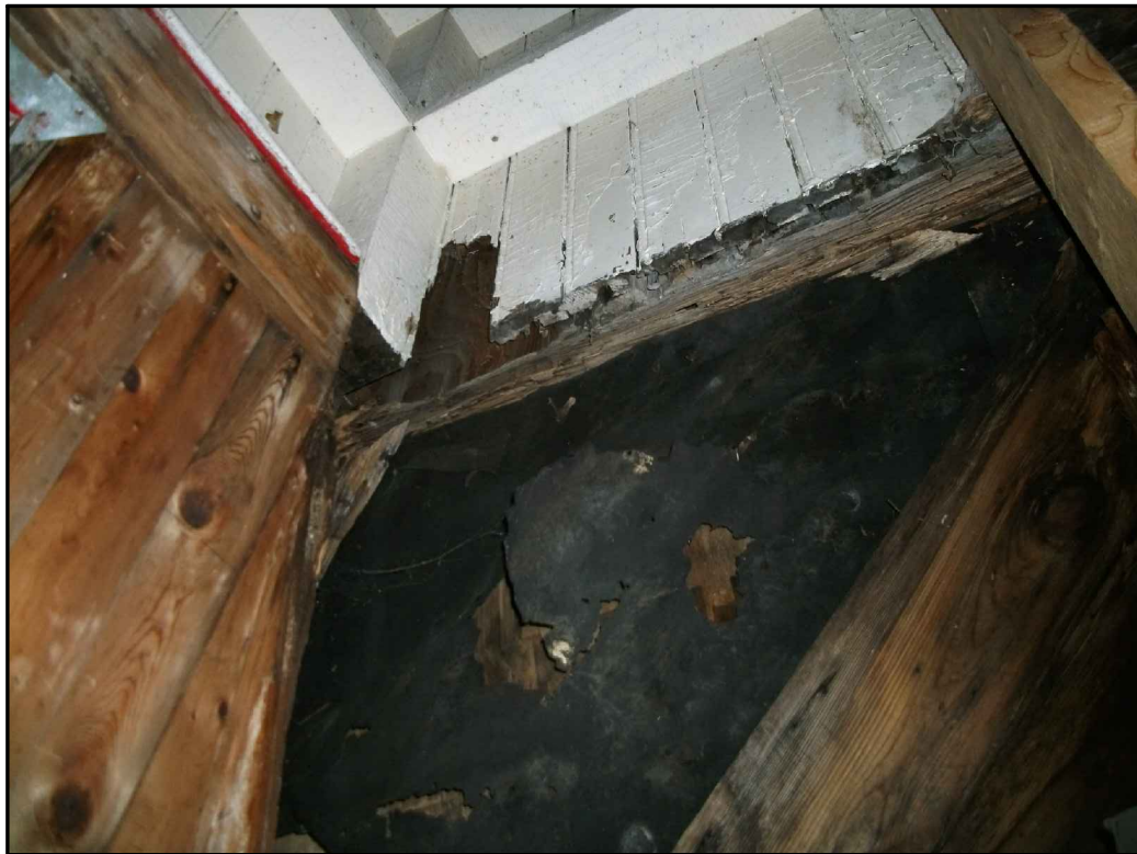
Photograph 15: Black insulating paper (non-ACM) visible on 3rd floor of Old Light Tower between layers of wood.
