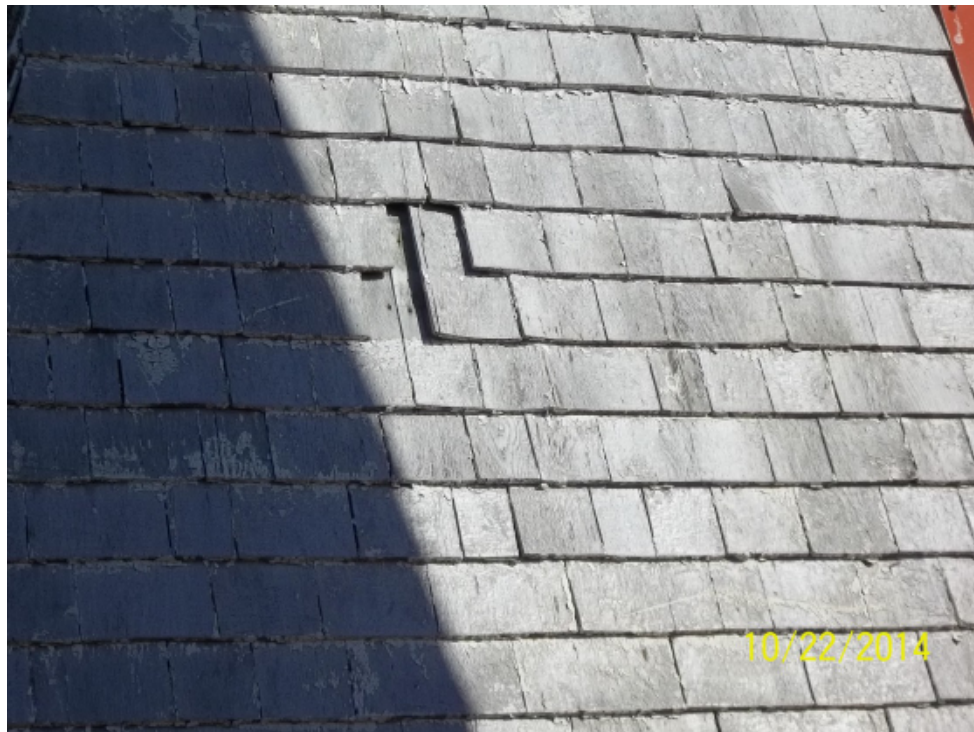
Photo 16: Some missing wood shingles on sloping wall.
