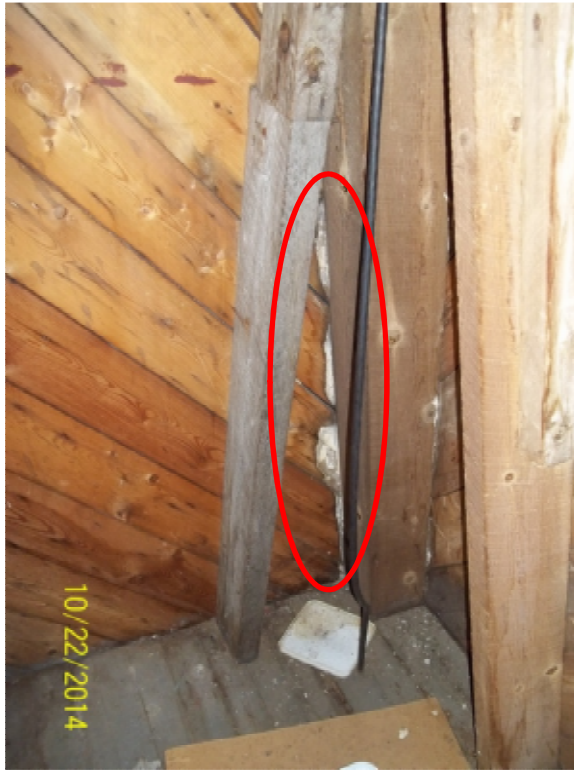
Photo 31: Dry rot around the corner post spreading onto diagonal lumber sheathing.
