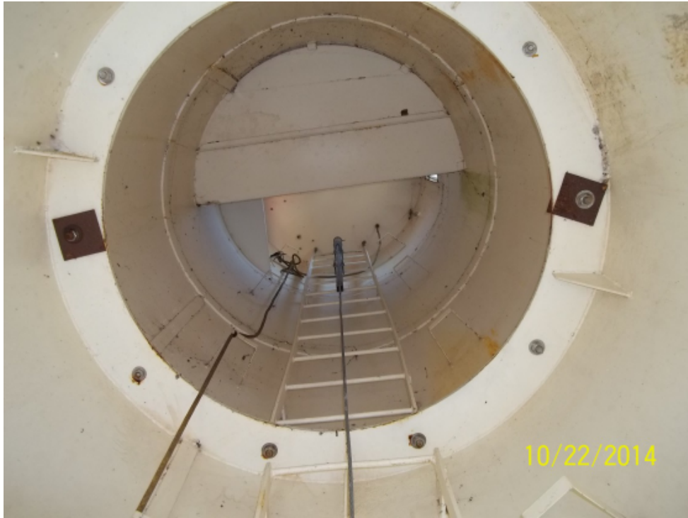
Photo 43: View from inside looking to the top of the steel tower. Bolted splice connection and ladder with cable for fall arrest device also shown.
