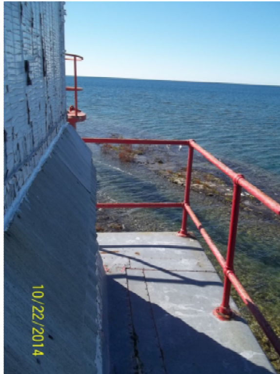
Photo 21: View northwest from exterior walkway; guard rail height below current heights, sheet steel roofing on walkway, caulked joints.
