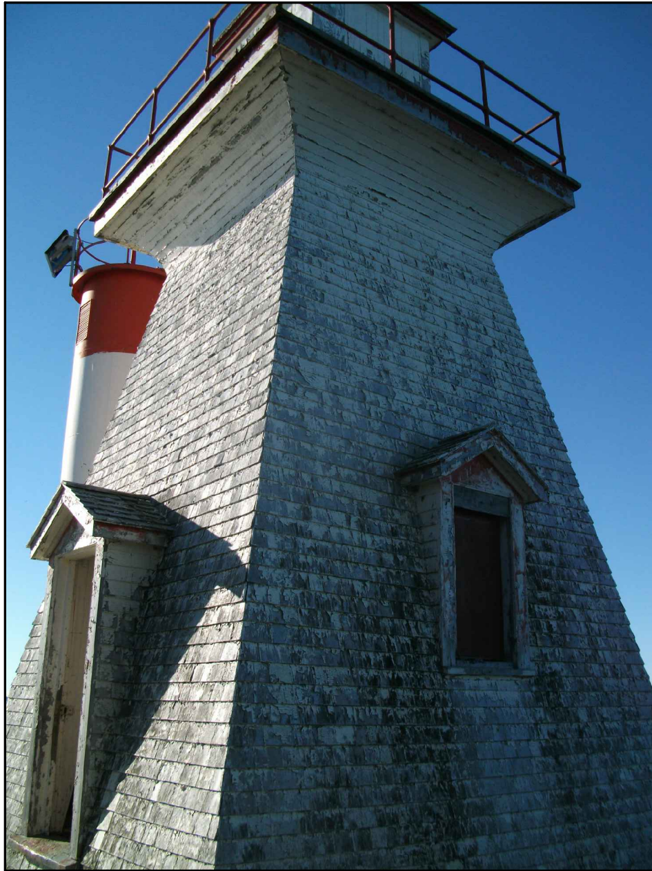
Photograph 11: White lead-based paint (poor condition) on exterior wood surface on 3rd floor of Old Light Tower.
