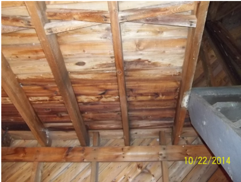
Photo 27: View of underside of second floor framing, material in good condition but showing water stains.
