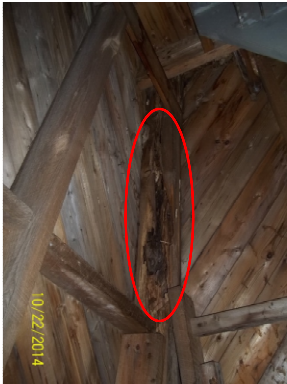
Photo 32: Southeast corner post – disintegrating.
