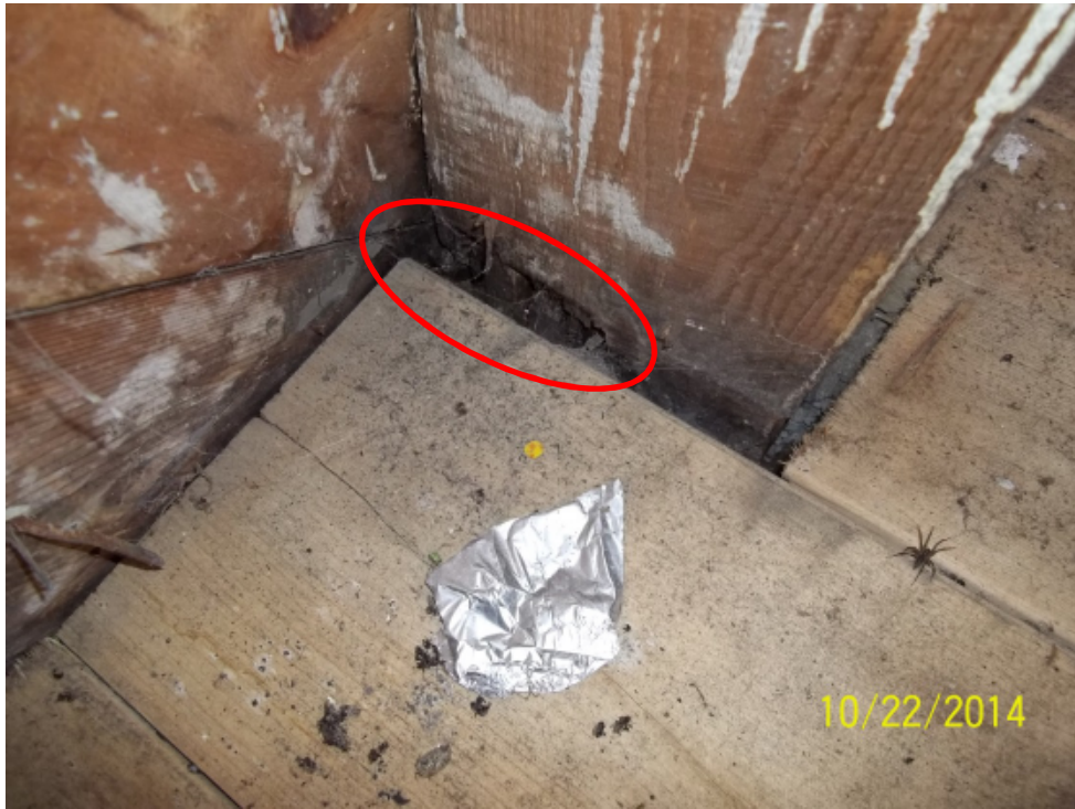
Photo 25: Side wall wood stud framing where the studs meet the ground floor. Note the wood rot at and below the floor level.
