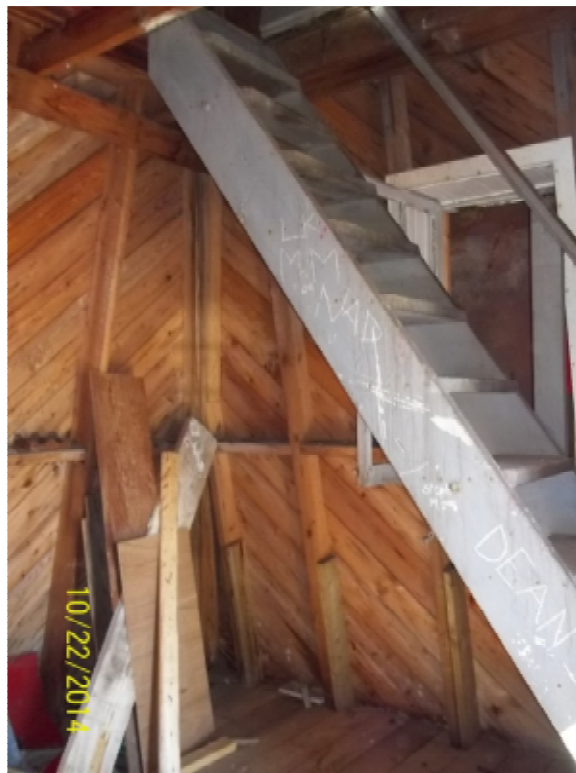
Photo 23: Interior east side with stairs to second level. Note the pressure treated spliced studs with the original studs at the ground floor.
