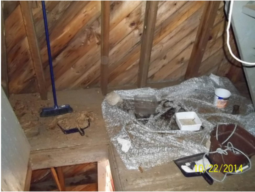
Photo 29: Second floor with access opening. Note the buckets and plastic used to contain water leaks.
