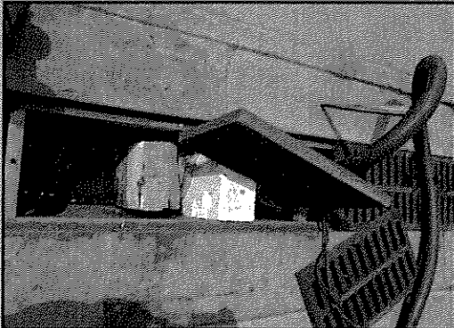
Example of styrofoam blocks used as a drain blocker on the NLW.
