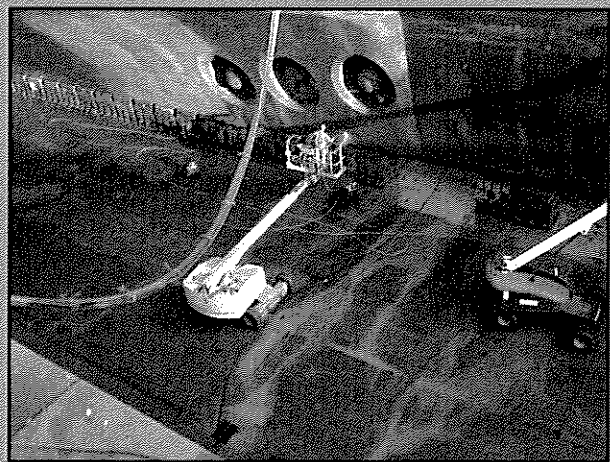
Antifoulant contaminated wash water entering the trench drain sump wells on dock bottom.
