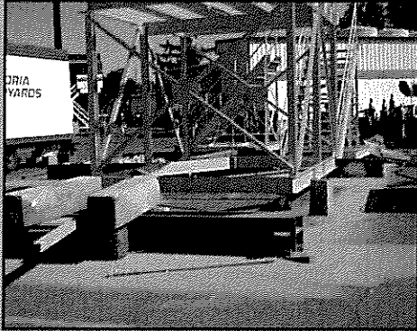
Ensure tarps are in place to prevent overspray impacting the surrounding work area.
