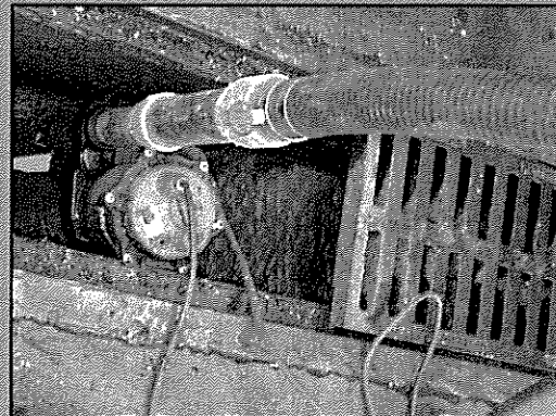
Example of a pump set up used to collect wash water on the NLW.
